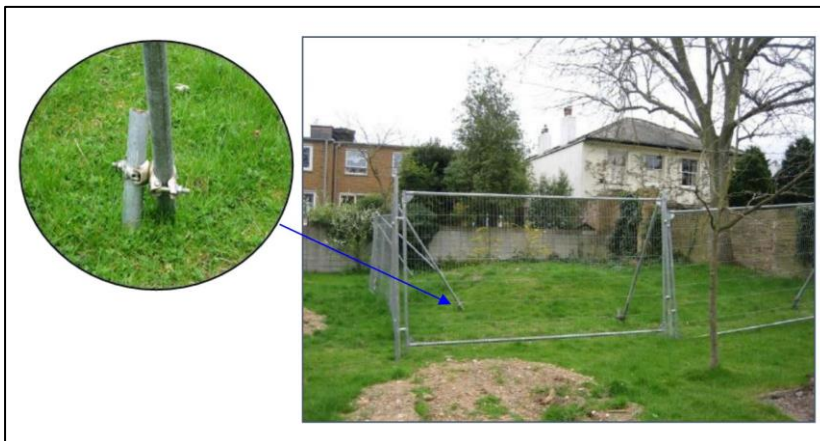
Figure 4.1: Example of mesh welded type barriers in-situ.
