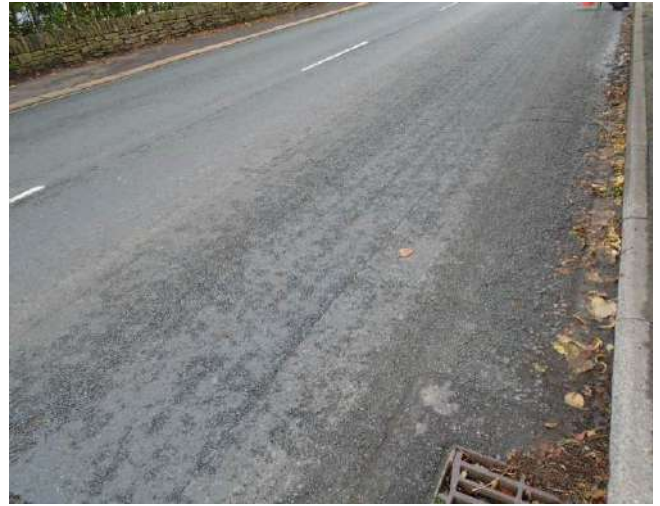
92. Erosion and scarring to road surface.
