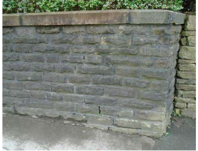
2. Cracking and disturbance to end of boundary wall near return.
