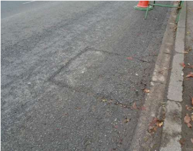
97. Historic repair, edges of repair are worn and uneven.
