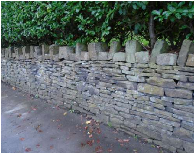
33. Dry stone wall. Numerous loose and defective stones present.
