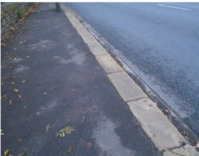
179. Views of kerb stones with erosion and damage present.
