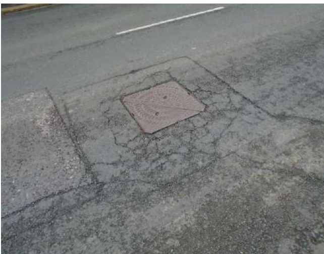
89. Cracking and disturbance to tarmacadam around inspection chamber.
