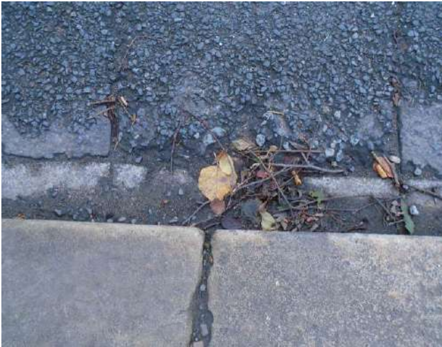
115. Cracked concrete edging adjacent to patch repair.
