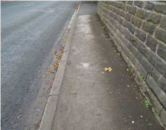
49. Cracked and splits within tarmacadam surface to pavement.
