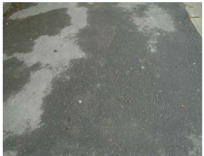
162. Worn tarmacadam surface with aggregate more exposed.
