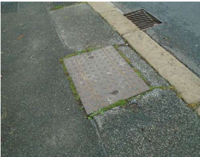
207. Cracking, splits and vegetation growth around inspection chamber.
