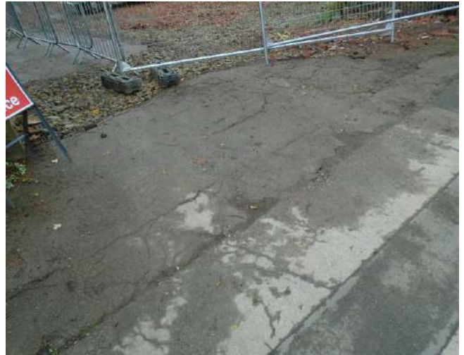
152. Cracking to tarmacadam in entrance to development site.
