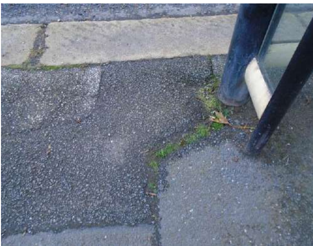
197. Worn/recessed tarmacadam adjacent to bus shelter. Uneven joints between different tarmacadam sections.
