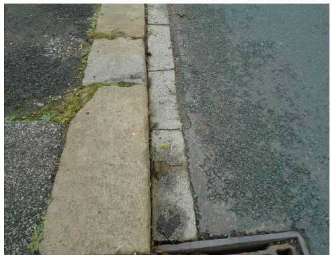
138. Cracking and misalignment to edgings alongside of carriageway in entrance to property adjacent to development site, 'Glen View'.
