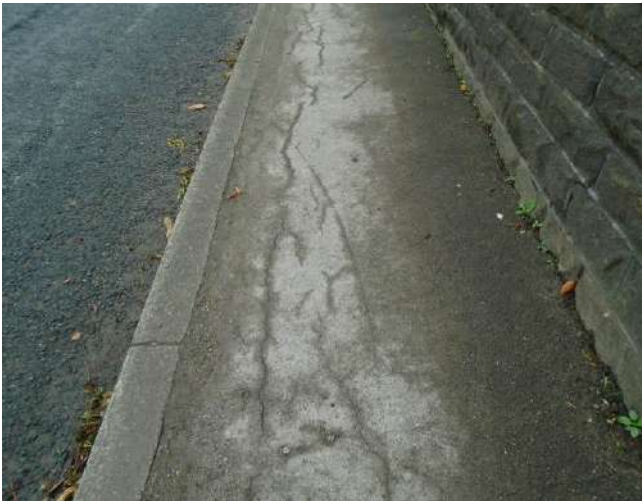
45. Cracks and splits to tarmacadam surface.
