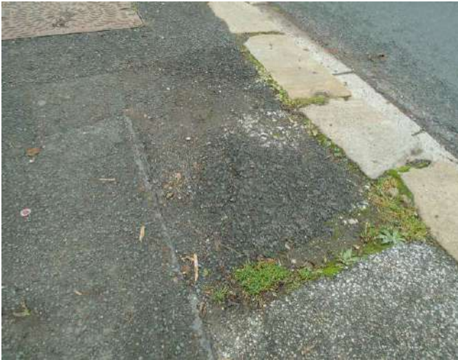
211. Vegetation growth, wear, uneven joints and erosion to tarmacadam surfacing.
