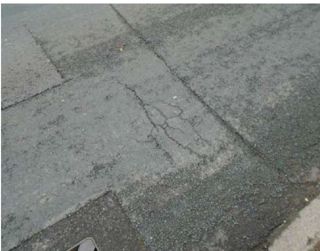
83. Cracking to tarmacadam.
