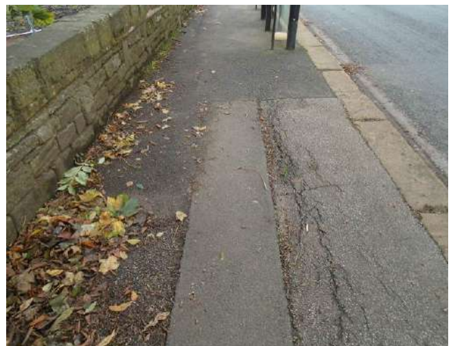
192. Scars and splits/cracks to tarmacadam surface. Paving is uneven approaching bus shelter.
