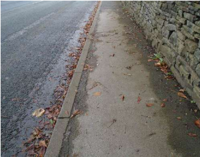
73. Isolated areas of cracking present to pavement. Edge of pavement uneven along kerb stone line.
