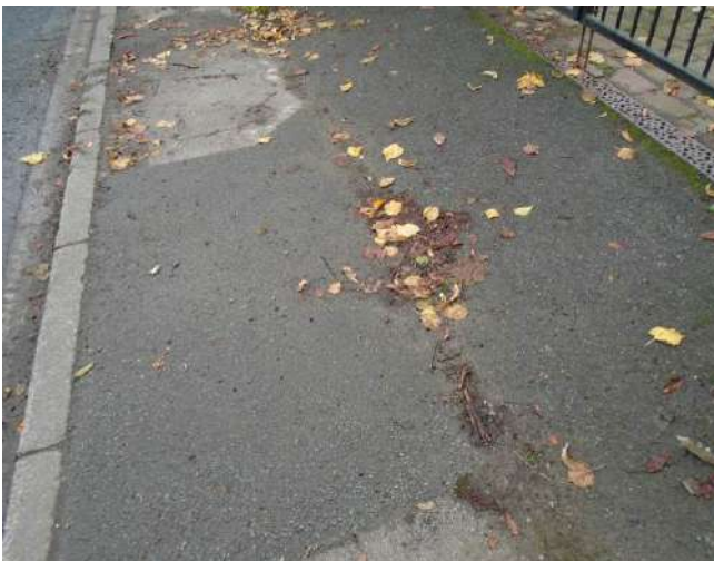
63. View of boundary line of number 6A and public footpath. Surface uneven as evidenced by leaves retained in low lying areas of pavement.
