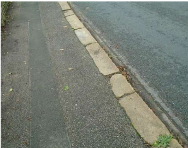
201. View of worn and eroded kerb stones to secondary entrance to development site.
