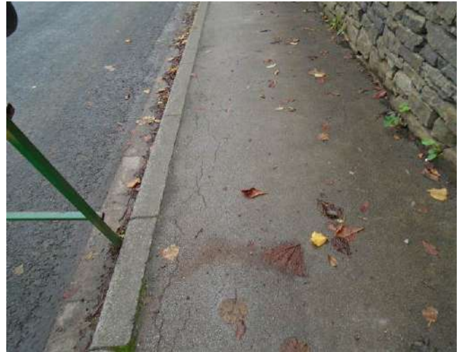
68. Cracking to tarmacadam surface of pavement. Edge of pavement uneven along kerb stone line.
