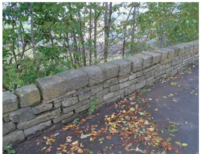
234. Dry stone boundary wall to development site. Isolated sections of mortar bedding to copings. Mortar bedding defective.
