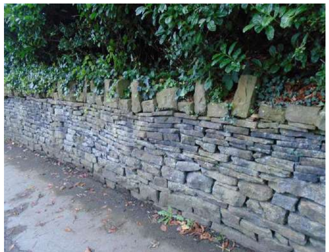
36. Dry stone wall. Numerous loose and defective stones present.
