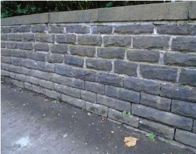
13. Erosion of mortar joints at low level to boundary wall.
