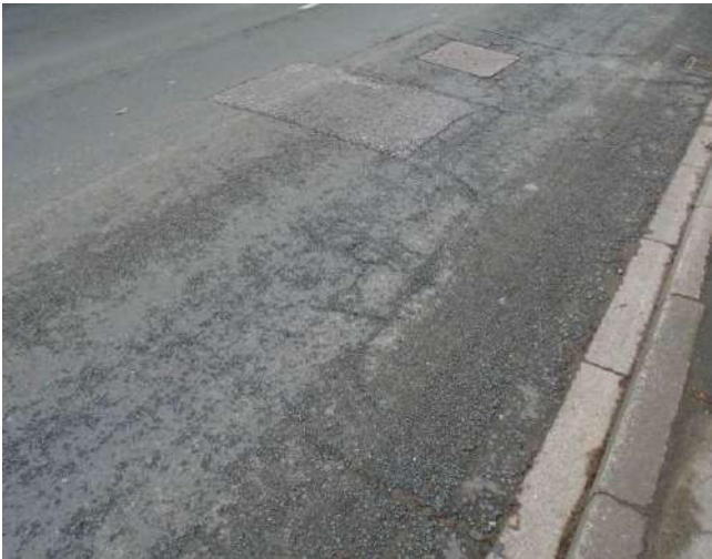
87. Scarring and cracking to road surface.
