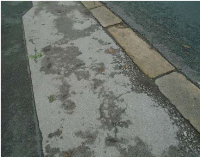
145. Cracking and erosion to tarmacadam adjacent to driveway entrance to 'Wynncliff'.
