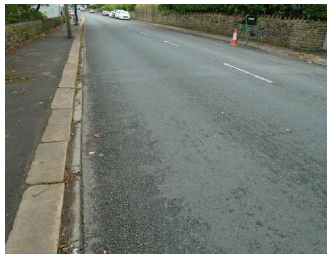
120. Erosion and wear to surface of tarmacadam roadway.
