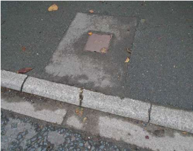
55. Cracking to concrete kerb stones.
