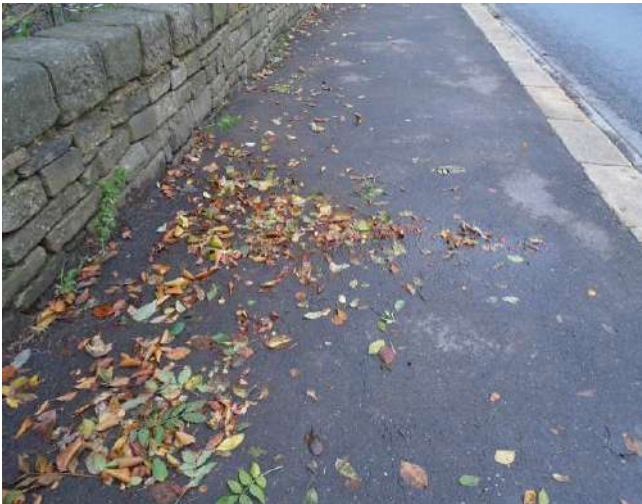
177. Uneven surfacing evidenced by area of standing water.
