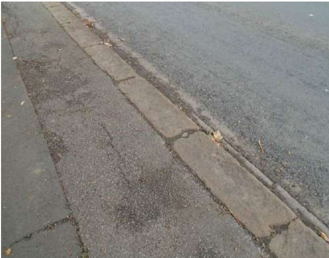
189. Worn and eroded kerb stones.
