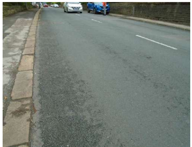
108. Erosion to surfacing of roadway.
