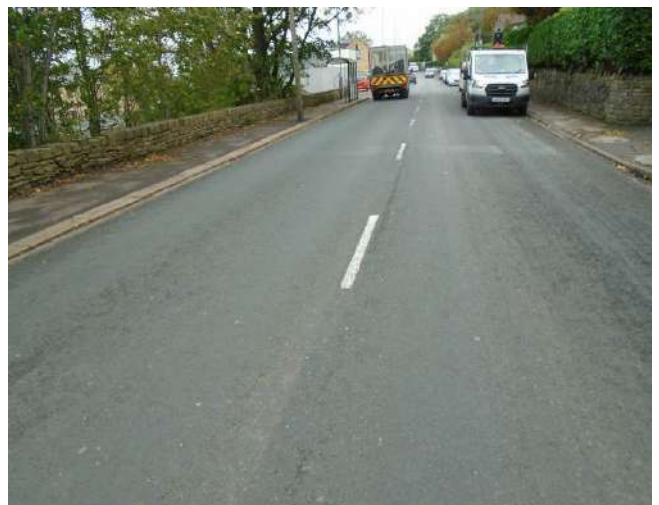
276. Thermoplastic line demarcation generally worn throughout extent of development site and beyond.
