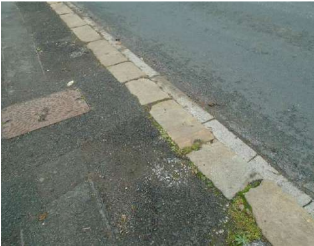
213. Damaged, eroded and worn kerb stones in entrance to property adjacent to development site.
