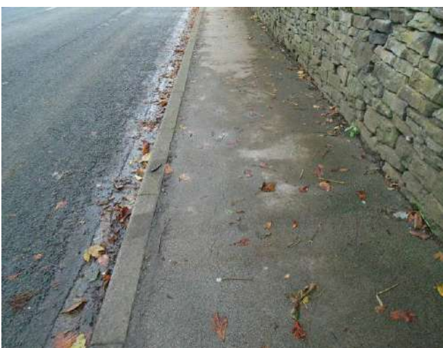
71. Isolated areas of cracking present to pavement. Edge of pavement uneven along kerb stone line.
