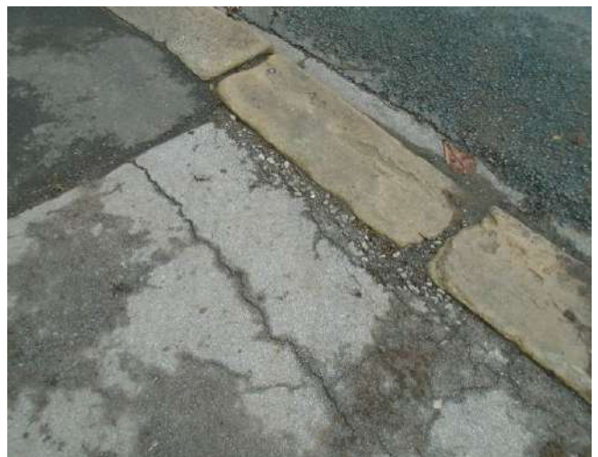
156. Eroded and worn tarmacadam and misaligned and eroded/worn kerb stones to dropped kerb to entrance into development site.
