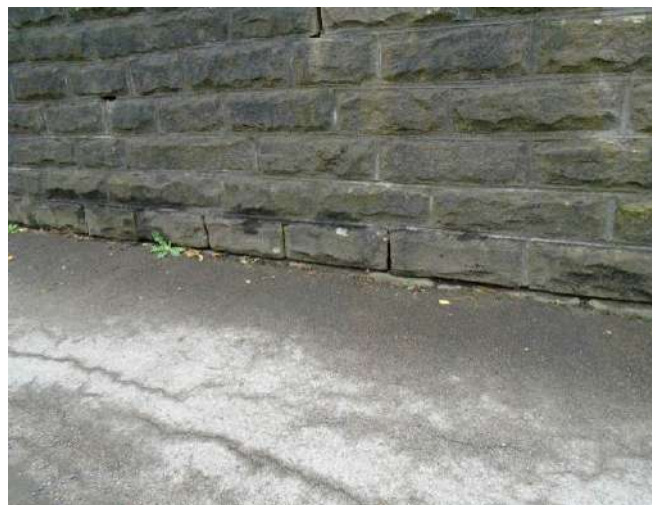
6. Erosion of mortar joints at low level.
