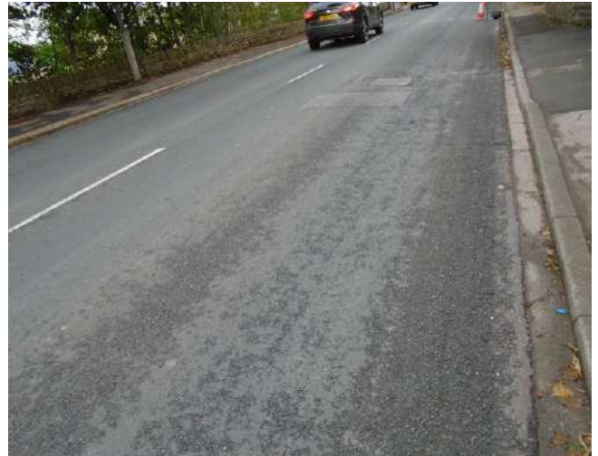
86. Wear and erosion to tarmacadam.
