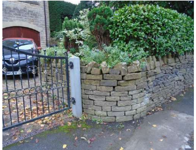
26. Return into driveway of 6A. Displacement to stonework.
