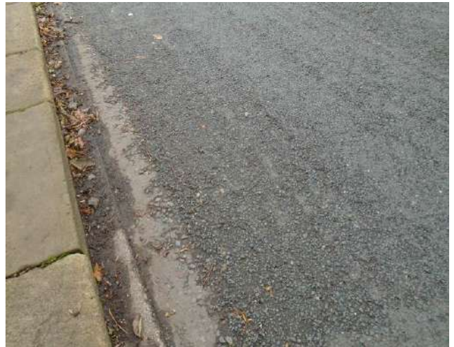
130. Erosion and wear to tarmacadam surface.
