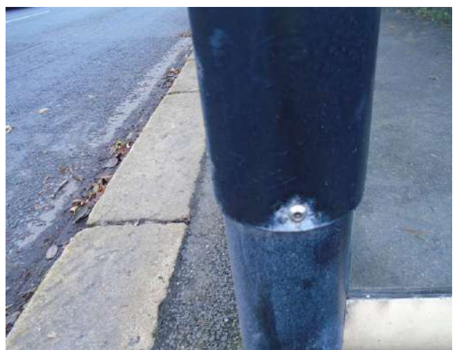
264. Pitting around screw fixings to access cover.
