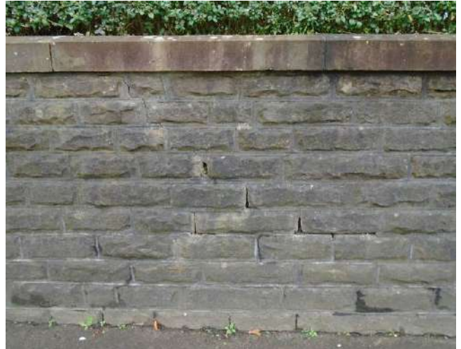
4. Cracking and defective mortar joints to wall.
