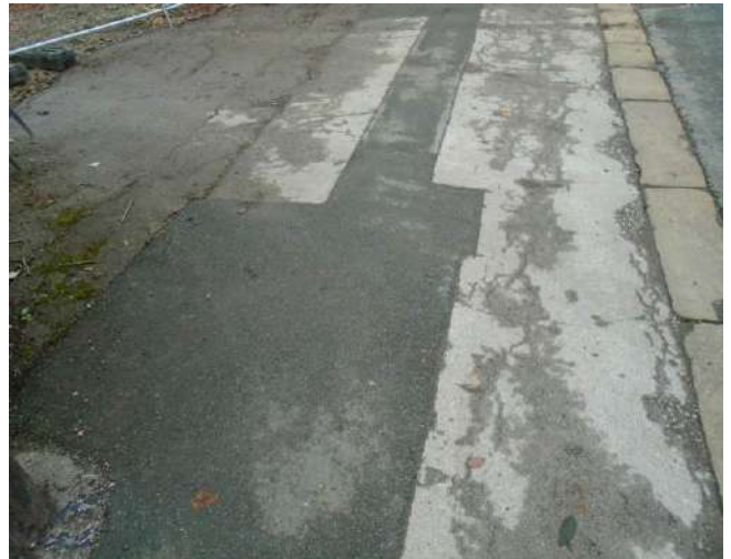
148. Patch repairs and cracking to tarmacadam.
