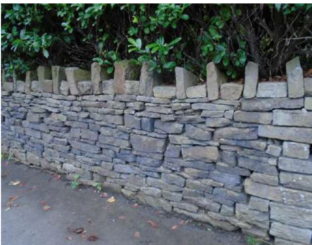
29. Dry stone wall. Numerous loose and defective stones present.
