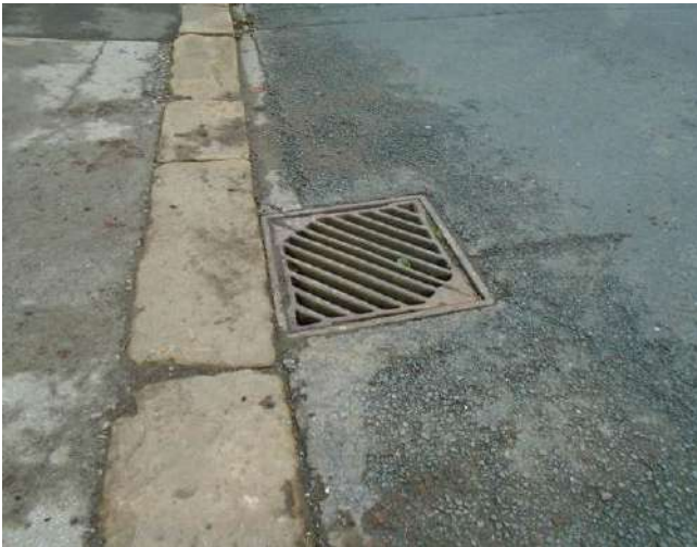
111. Gully adjacent to gateway to development site. Gully grate mis-seated and sunken within surrounding tarmac.
