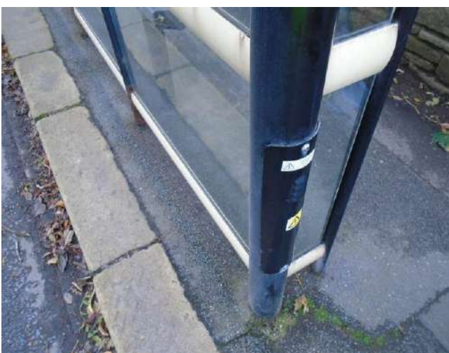
263. Soiling and discolouration of post to bus shelter.
