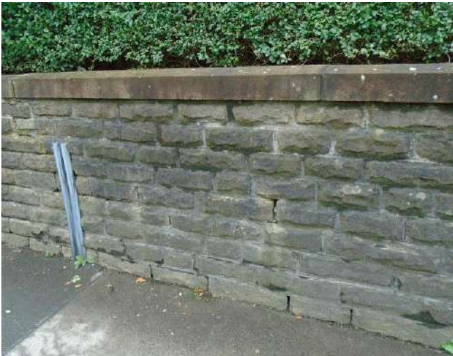
9. View of boundary wall, localised areas of open and defective mortar joints.
