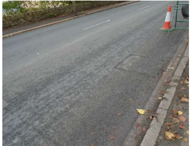
98. Erosion to tarmacadam surfacing.
