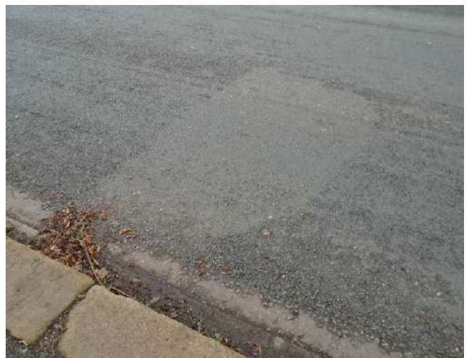
132. Non-matching section of surface adjacent to bus shelter.
