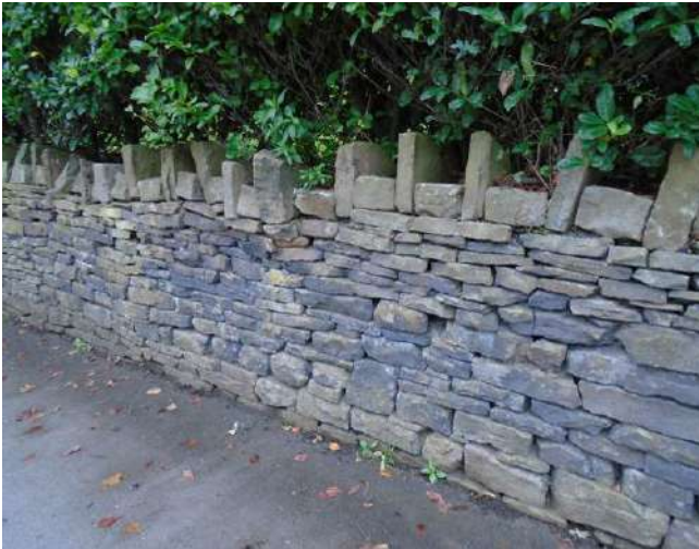
31. Dry stone wall. Numerous loose and defective stones present.
