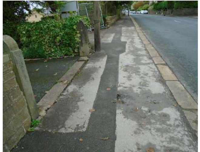
140. View along pavement looking north. Patch repair along line of excavation relating to utilities.
