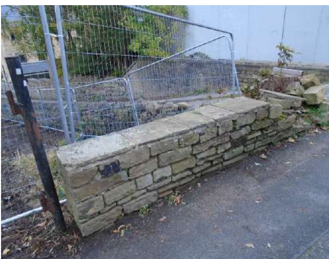
245. Dry stone wall to boundary of development site. Area of damage wall evident to corner returning to property on adjacent site.
