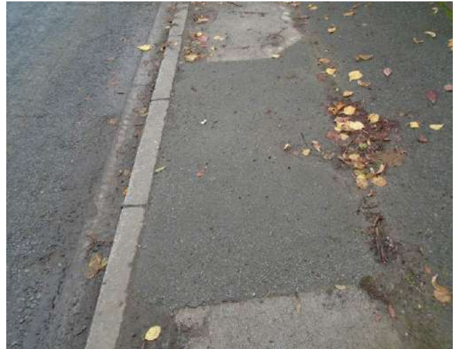
62. Patched repaired tarmacadam surface to pavement. Surface uneven as evidenced by leaves retained in low lying areas of pavement.
