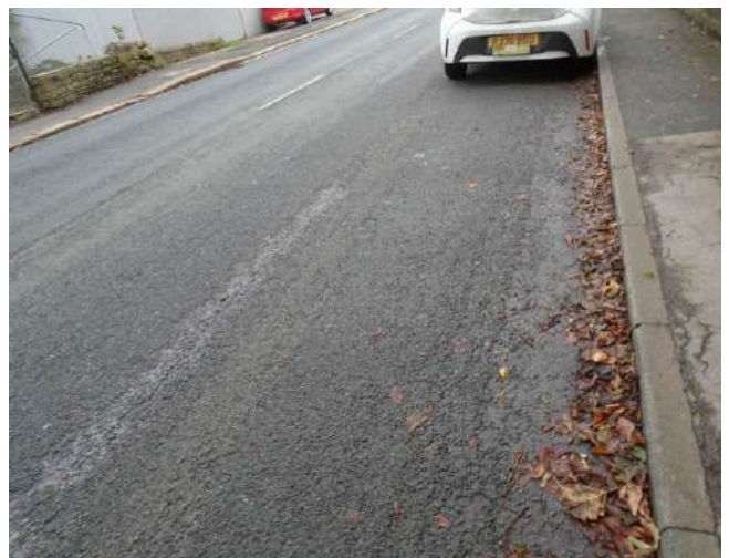
102. Worn/eroded surfacing to tarmacadam.
