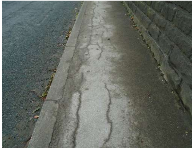
44. Cracks and splits to tarmacadam surface.
