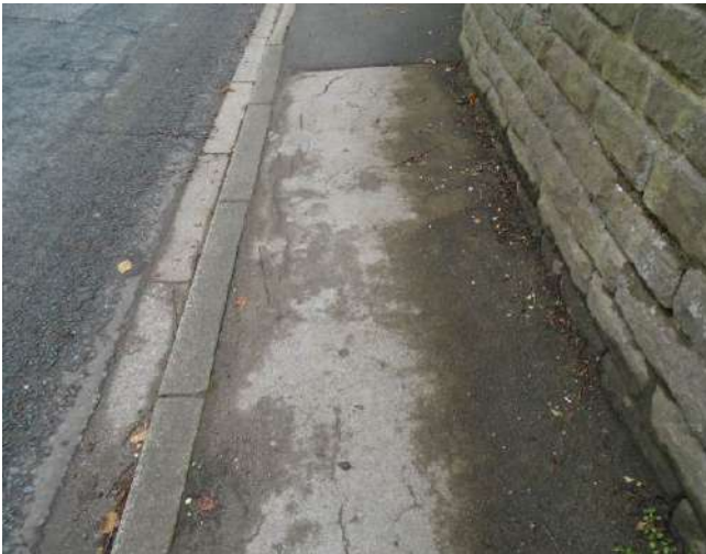
51. Cracks and splits to tarmacadam surface.
