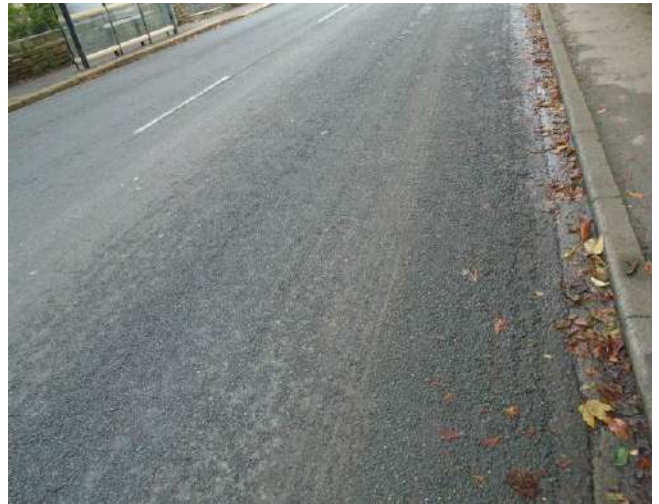
100. Worn/eroded surfacing to tarmacadam.
