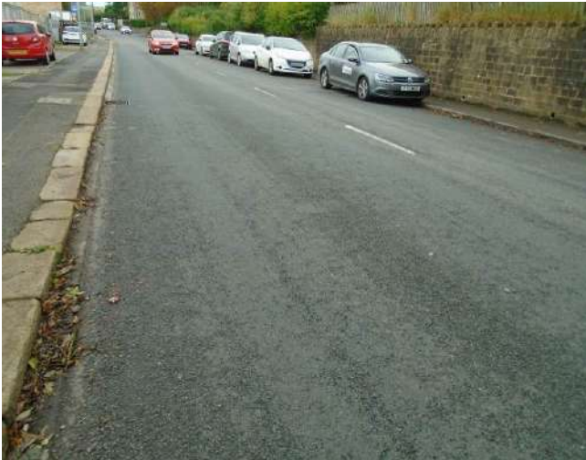
133. Worn surfacing to roadway.
