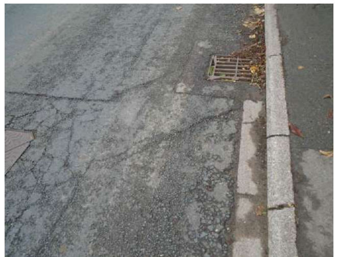
90. Patch repairs between inspection chamber and gully.
