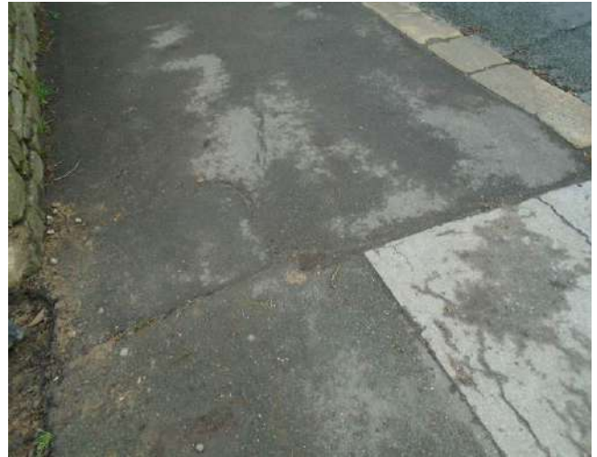
158. Patch repair to tarmacadam adjacent to development site entrance. Uneven area of tarmacadam present where various ages of tarmacadam abut.
