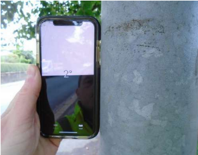
253. Lamp post is slightly out of plumb, leaning inwards towards the development site by approximately 2 degrees.
