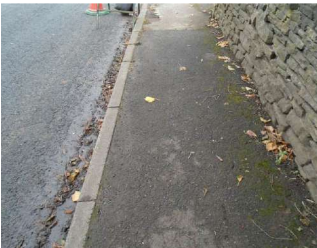
59. Localised cracking and eroded tarmacadam to footpath.
