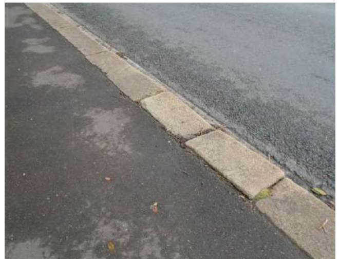
166. Uneven and misaligned/sunken kerb stones.
