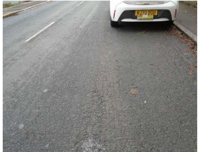
104. Cracking to road surface, worn and eroded tarmac.
