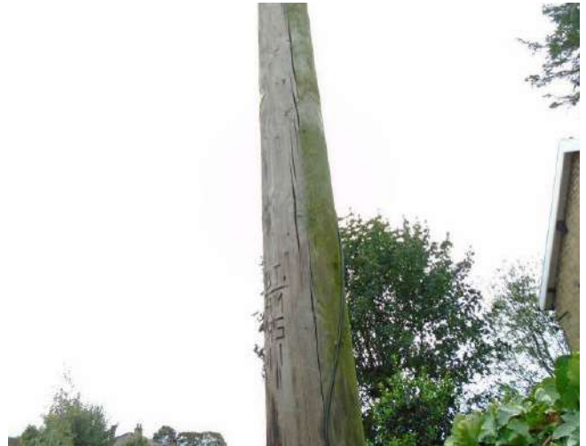
248. Examples of cracks and splits to telegraph post.
