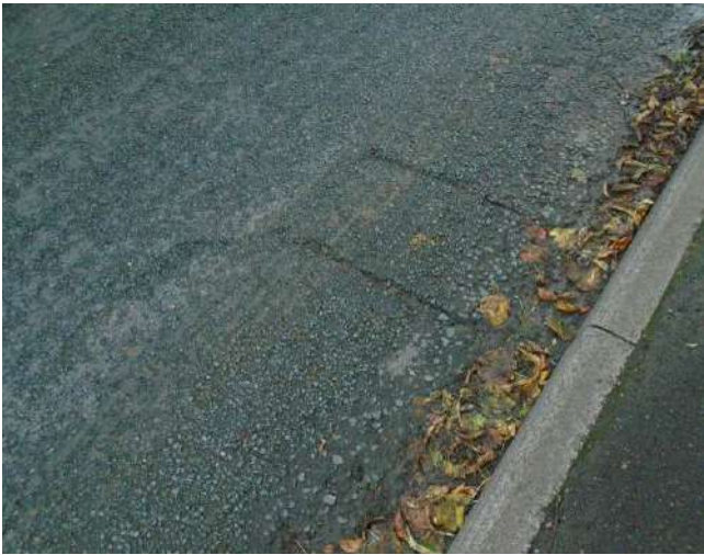
93. Cracks and disturbance to tarmacadam.
