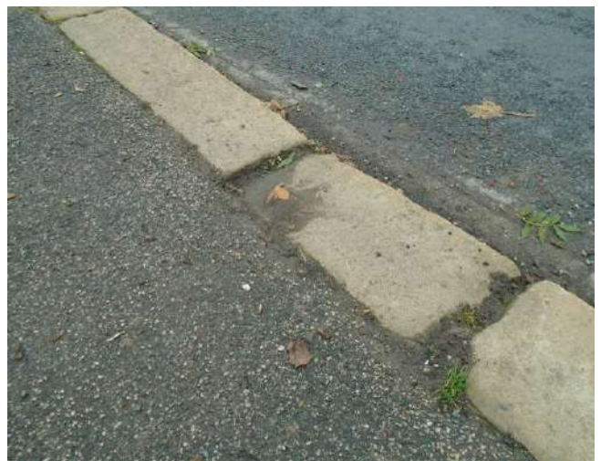
204. Misaligned kerb stones to secondary entrance into development site.
