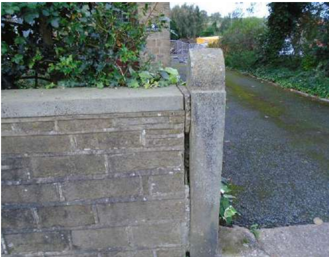
219. Damaged/defective pointing between 'Wynncliff' boundary wall and gate post.
