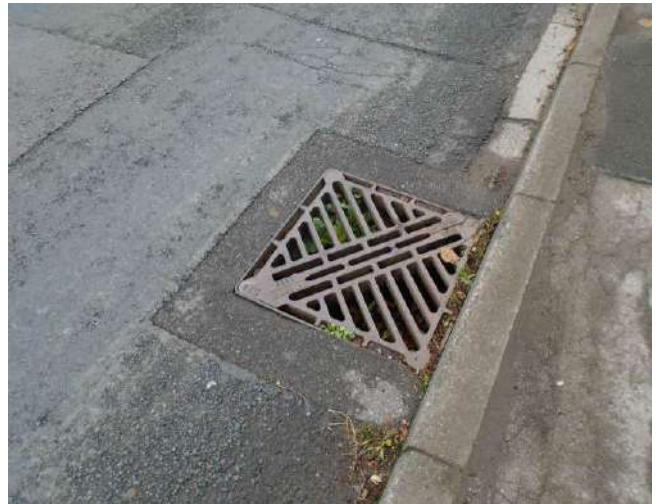
82. Patch repairs around gully.
