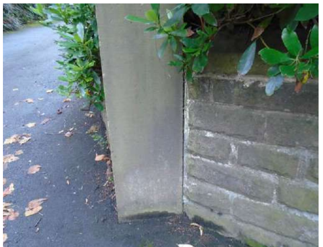
18. Cracking/open joint between gatepost and wall.
