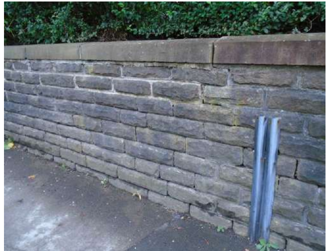
10. Localised areas of open and defective mortar joints.
