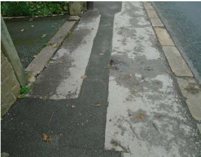
141. View of pavement in front of property adjacent to development site 'Wynncliff'. Patch repairs, cracking and damage evident to tarmacadam. Kerb stones are worn and eroded.
