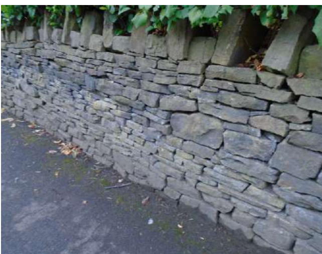
23. Section of dry stone wall. Assorted loose and defective stones present.
