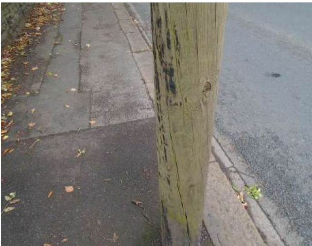
255. Examples of cracks and splits to telegraph pole.
