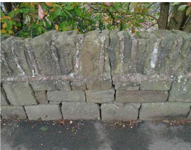
227. Cracking to boundary wall. Copings bedded on mortar.
