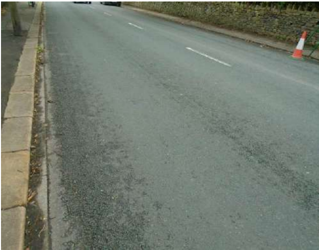
123. Erosion to tarmacadam surface.
