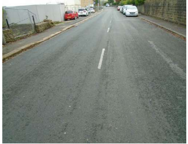
278. Thermoplastic line demarcation generally worn throughout extent of development site and beyond.
