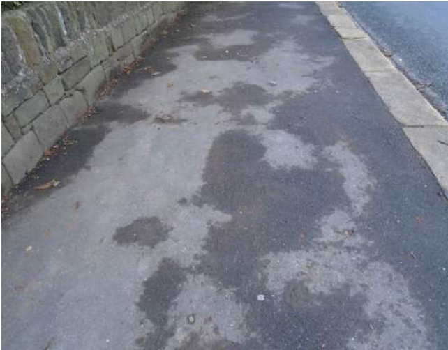
163. Surface of tarmacadam slightly uneven as evidenced by damper patches in lower sections.
