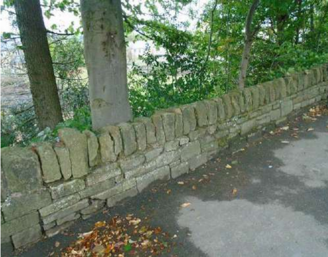
229. Boundary wall to development site. Section of wall leans inwards towards site.
