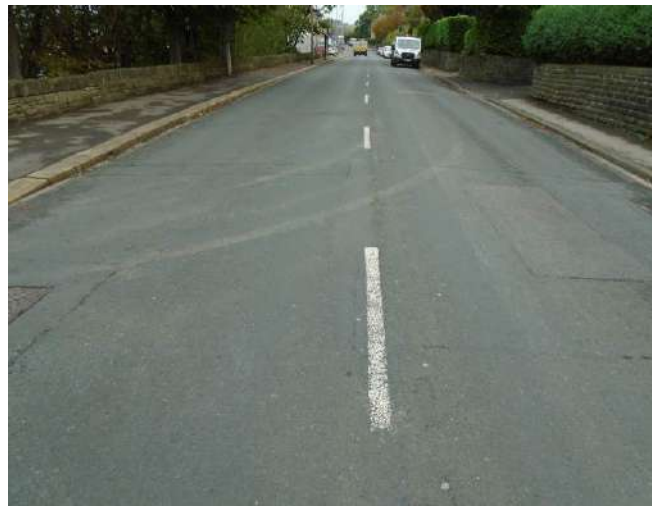
274. Thermoplastic line demarcation generally worn throughout extent of development site and beyond.
