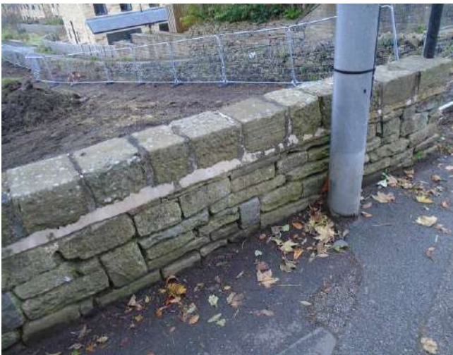
243. Dry stone wall to boundary of development site. Mortar bedding to copings.
