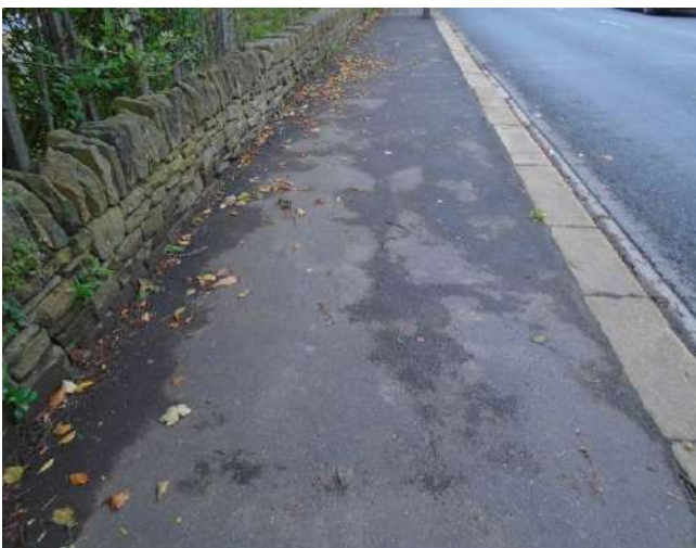
173. Cracking and scarring to tarmacadam surfacing of footpath. Kerb stones are eroded.
