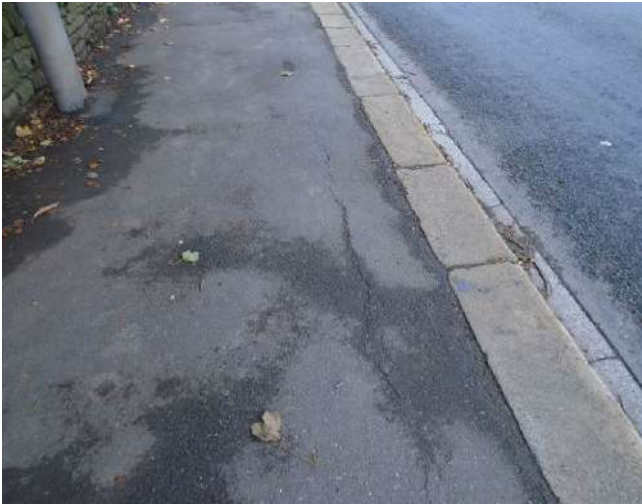
169. Cracking to tarmacadam surface adjacent to lamp post. Kerb edgings eroded and worn.
