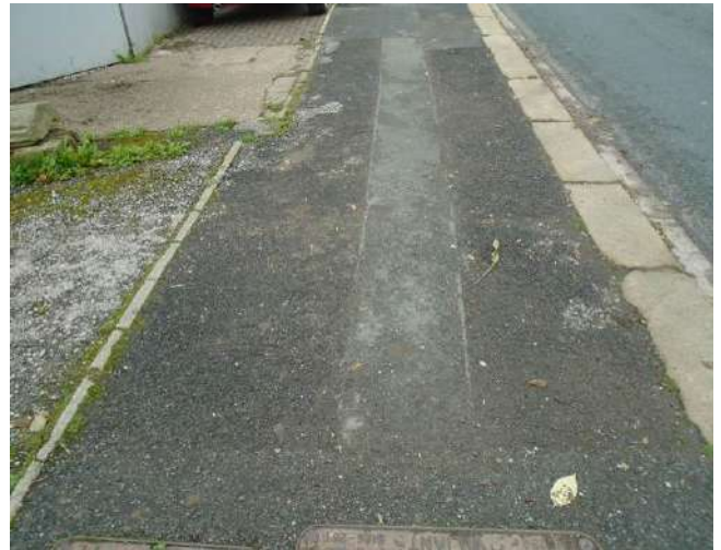
214. Worn tarmacadam surfacing to footpath. Surfacing is uneven and aggregate is exposed.
