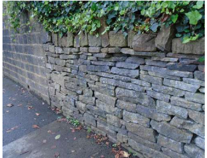
38. Dry stone wall. Numerous loose and defective stones present.
