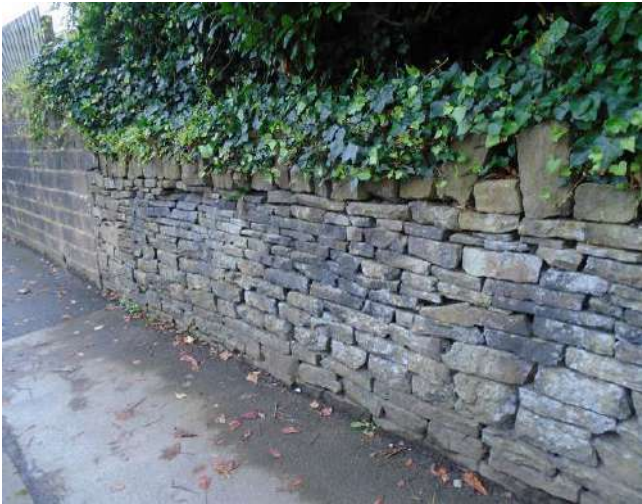
37. Dry stone wall. Numerous loose and defective stones present.
