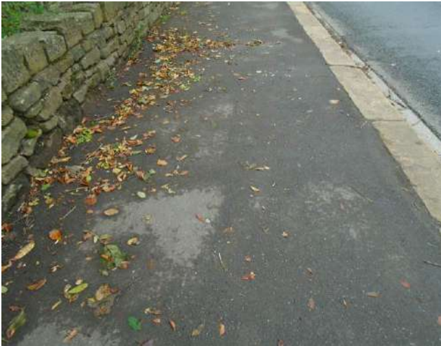
175. Scarring/cracking to pavement.
