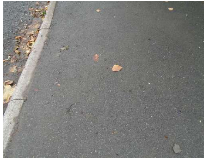
56. Localised indentations/scarring to tarmacadam to resurfaced area.
