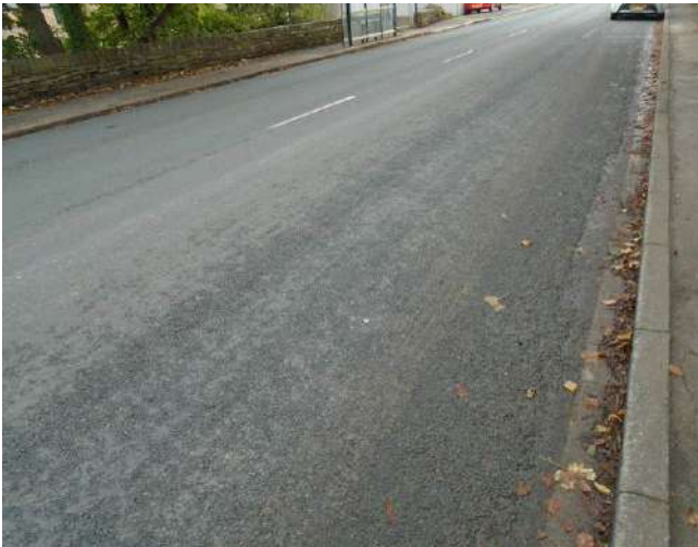
99. Worn surfacing to tarmacadam.
