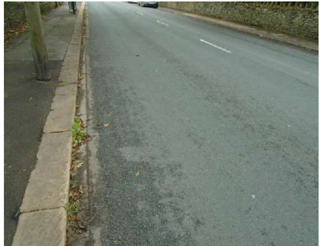
124. Erosion to tarmacadam surface.
