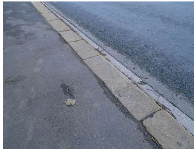
172. Examples of eroded and cracked kerb stones.
