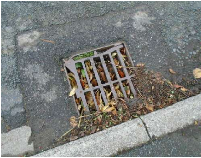
91. Gully blocked with vegetation/debris.
