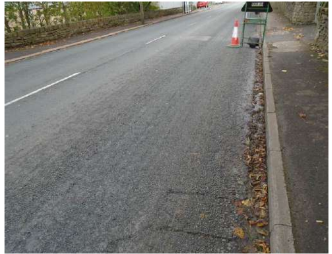
94. Erosion to road surface.
