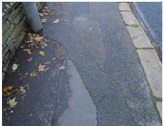
198. Tarmacadam surfacing has uneven/worn edges and cracking present in isolated areas.
