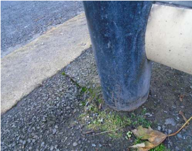
265. Corrosion to post at low level.
