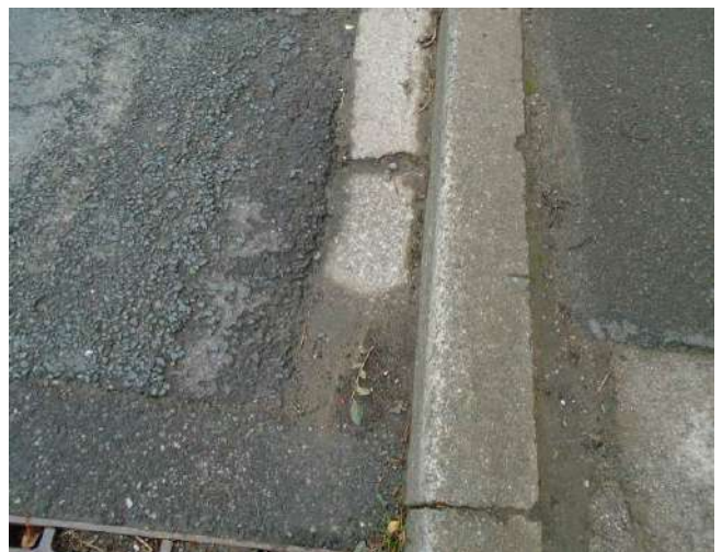
84. Cracking to concrete edgings.
