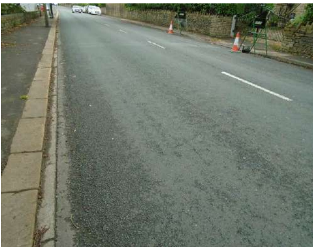
119. Erosion and wear to surface of tarmacadam roadway.
