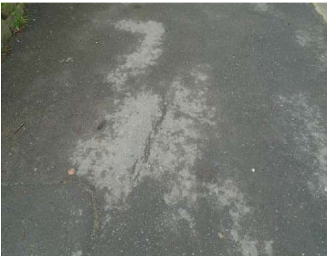
159. Scarring and cracks to tarmacadam surface.
