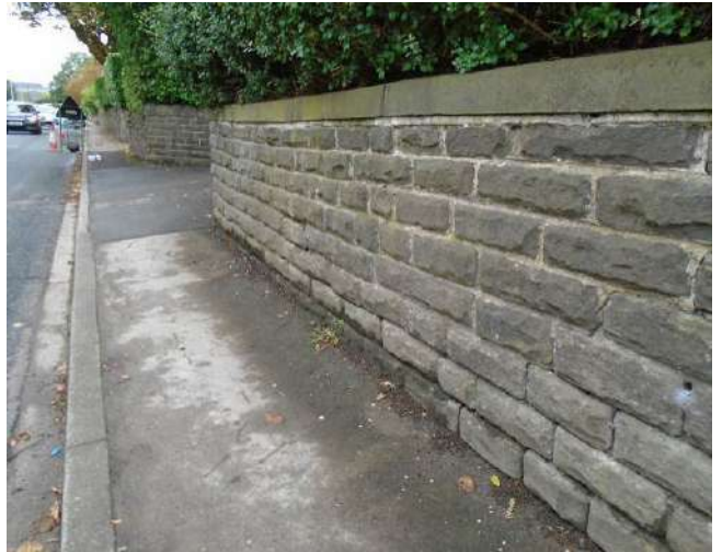
14. Erosion of mortar joints at low level to boundary wall.
