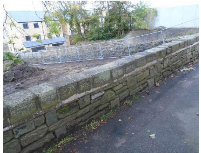
242. Dry stone wall to boundary of development site. Mortar bedding to copings.
