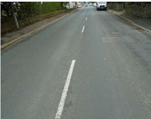
275. Thermoplastic line demarcation generally worn throughout extent of development site and beyond.
