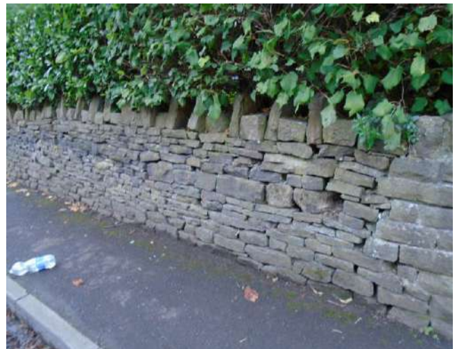
22. Section of dry stone wall. Assorted loose, missing and defective stones present.
