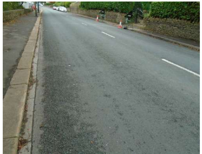
118. Erosion and wear to surface of tarmacadam roadway.
