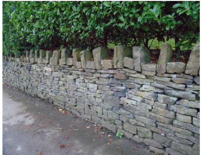
34. Dry stone wall. Numerous loose and defective stones present.
