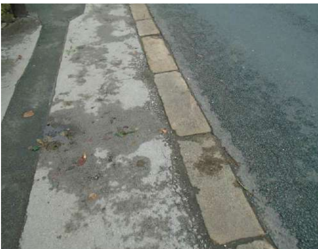
143. Worn, damaged and eroded kerb stones in front of 'Wynncliff'.
