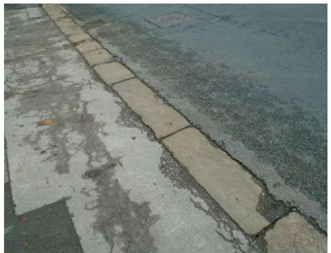
150. Damaged, eroded and worn kerb stones to entrance into development site.
