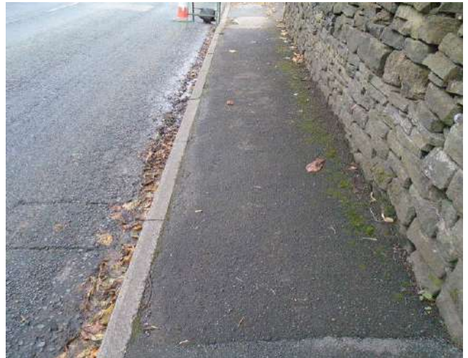
58. Localised cracking and eroded tarmacadam to footpath.
