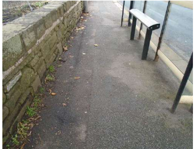
194. Areas of uneven tarmacadam adjacent to bus shelter.
