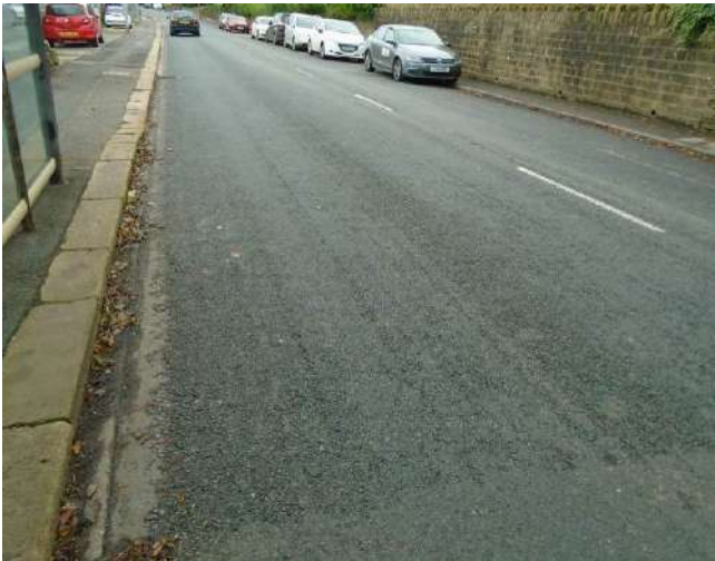
129. Erosion to tarmacadam surfacing.
