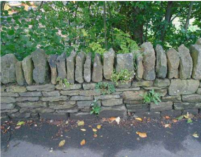
231. Vegetation growth present to boundary wall.
