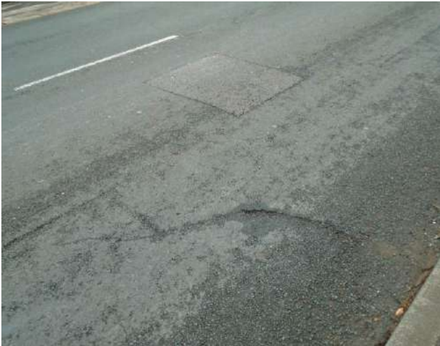
79. Indentations/scarring and patch repairs.
