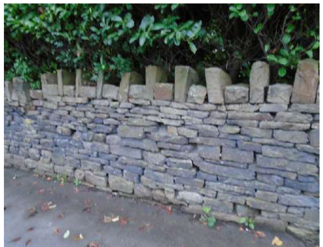
30. Dry stone wall. Numerous loose and defective stones present.
