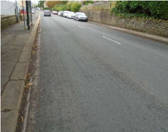
127. Erosion to tarmacadam surfacing.
