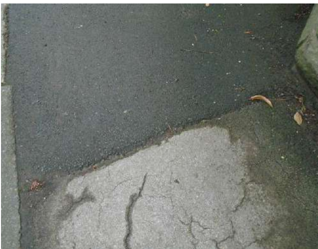
53. Poor joint to original and resurfaced tarmacadam at entrance to May Bank Villa.
