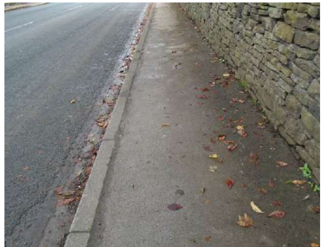
70. Isolated areas of cracking present to pavement. Edge of pavement uneven along kerb stone line.
