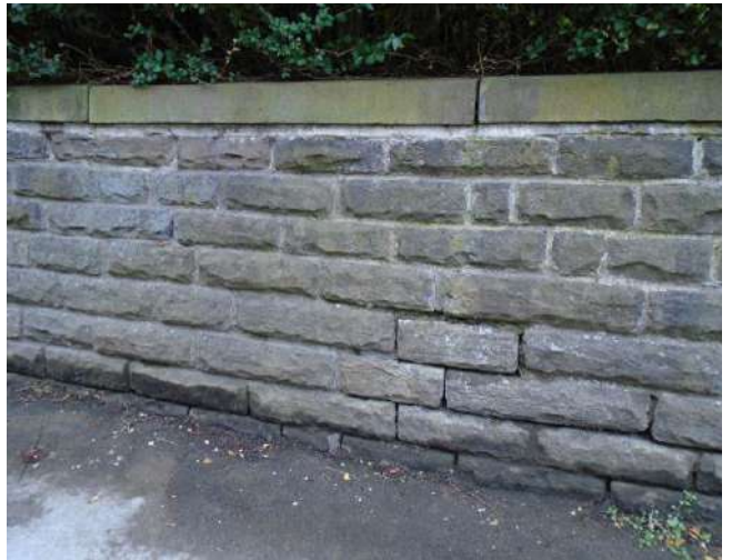
16. Erosion of mortar joints to boundary wall.
