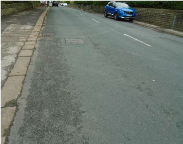
109. Erosion to surfacing of roadway.
