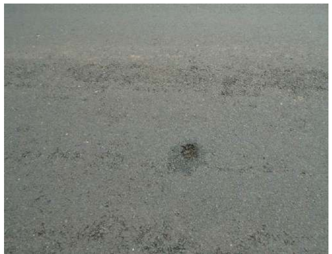
126. Worn/indented tarmacadam to surface of roadway.
