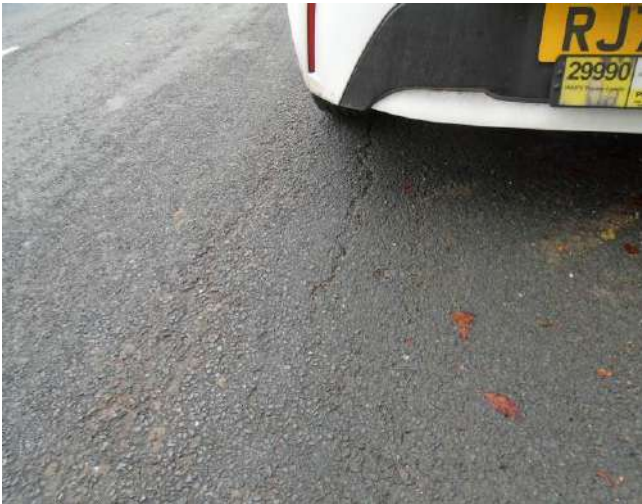
105. Cracking to tarmac.
