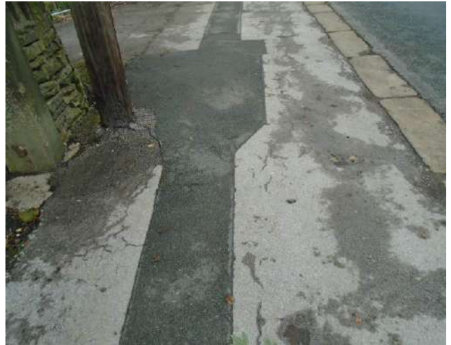
146. Patch repairs and cracking to original tarmacadam.
