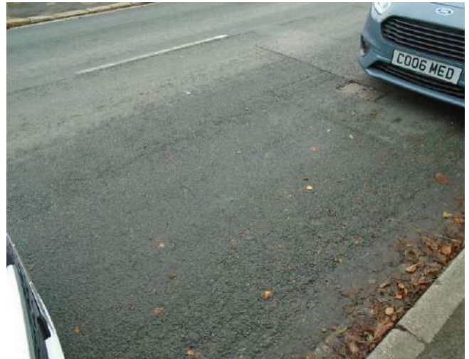
106. Patch repairs to road surface. Tarmac uneven around water inspection chamber.
