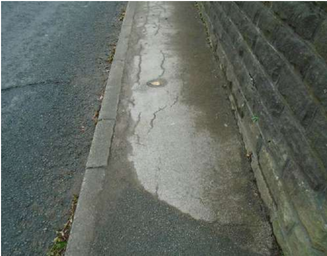
43. Cracks and splits to tarmacadam surface.
