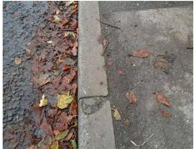
76. Damage to kerb stone adjacent to change in tarmac surfacing.
