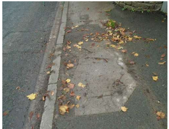
64. Disturbance to tarmacadam surface within driveway entrance area to 6A.
