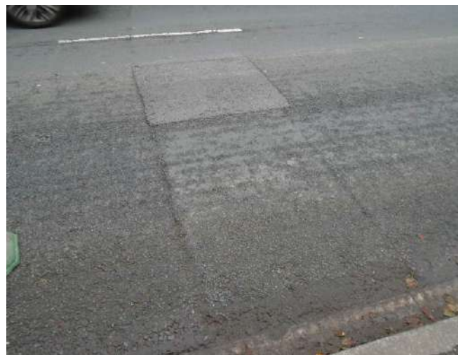
96. Patch repairs to tarmacadam and worn joints between previous repairs.
