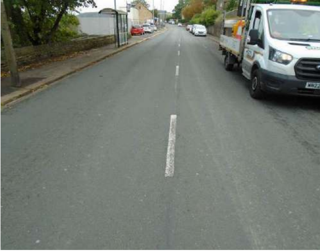
277. Thermoplastic line demarcation generally worn throughout extent of development site and beyond.
