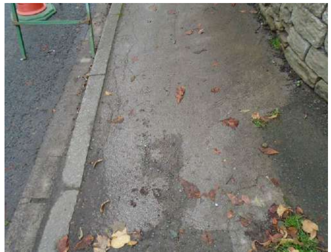
66. Cracking to tarmacadam surface of pavement. Edge of pavement uneven along kerb stone line.
