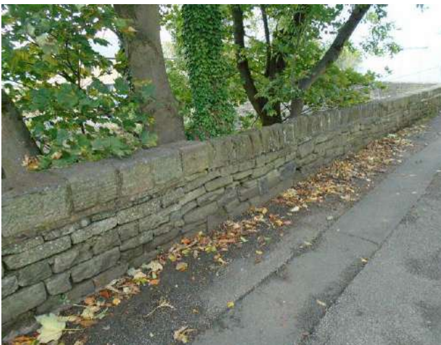
239. Dry stone wall to boundary of development site. Areas of misaligned and disturbed stonework present to wall. Mortar bedding to copings locally cracked/defective.
