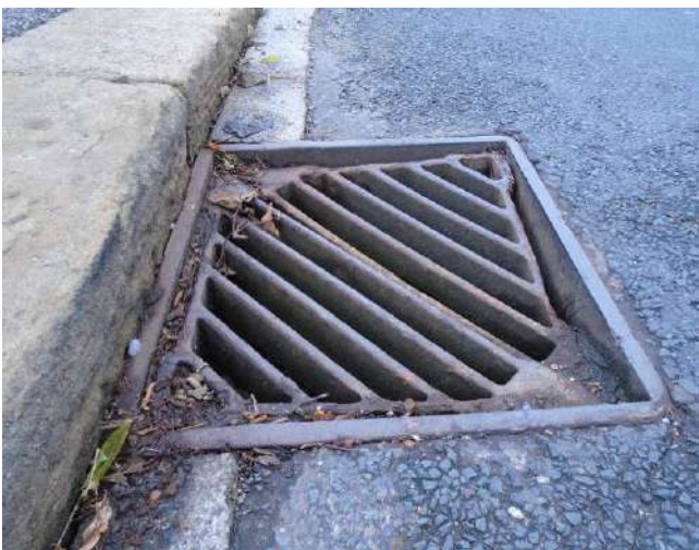
137. View of gully adjacent to property neighbouring development site, 'Glen View'. Gully is corroded, sunken and mis-seated.
