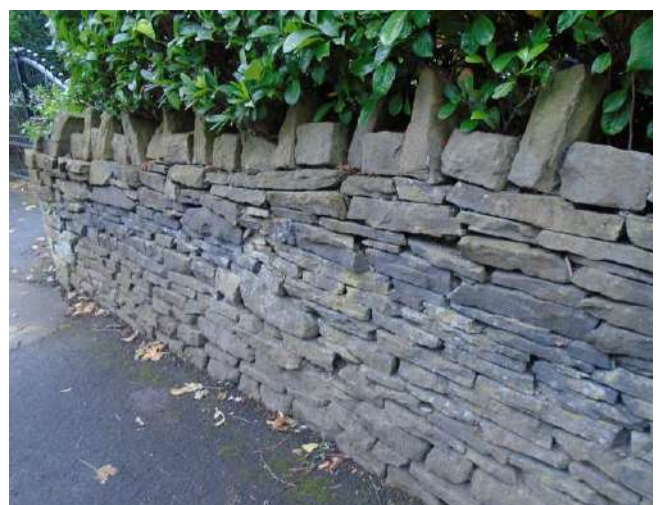
24. Section of dry stone wall. Assorted loose and defective stones present.
