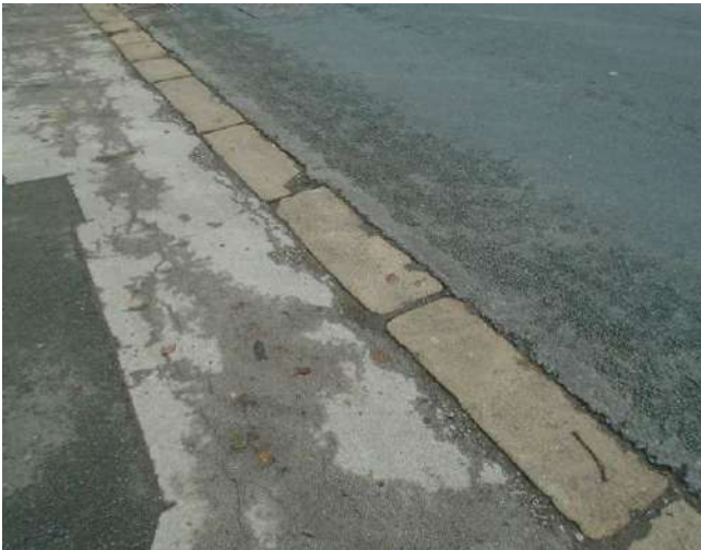
147. Eroded, worn and damaged kerb stones at entrance into development site.
