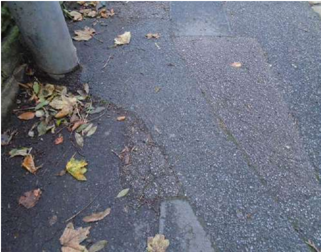
199. Tarmacadam surfacing has uneven/worn edges and cracking present in isolated areas.
