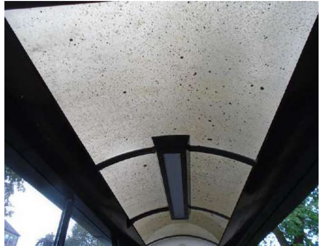
266. Soiling and algae to roof of bus shelter.
