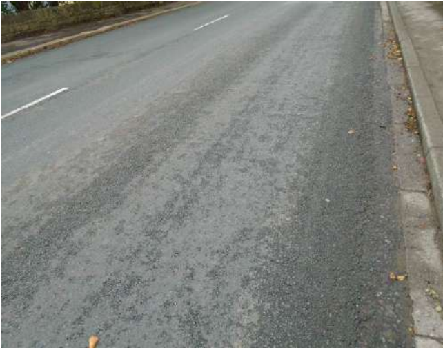
85. Wear and erosion to tarmacadam.
