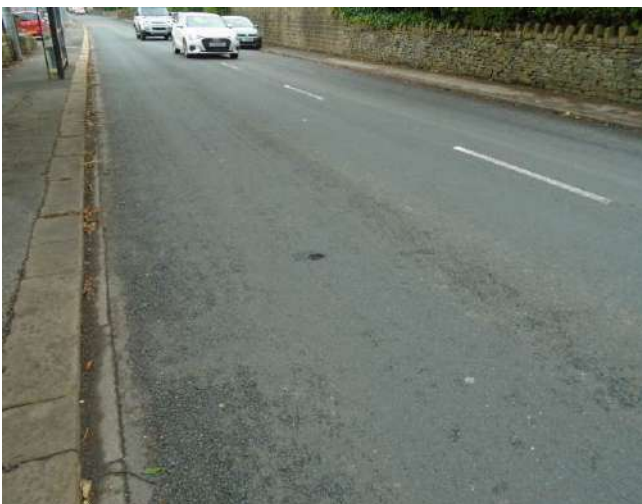
125. Erosion to tarmacadam surface.
