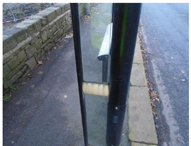
258. Scratched, graffiti and soiling to post of bus shelter.
