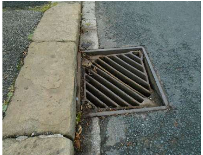
136. View of gully adjacent to property neighbouring development site, 'Glen View'. Gully is corroded, sunken and mis-seated.
