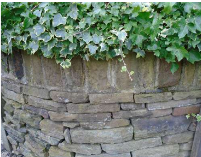
221. View of dry stone wall boundary to 'Wynncliff'. Isolated areas of mortar present mainly along copings, cracked and defective in areas.
