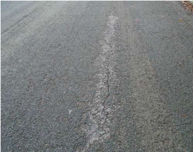
103. Cracking to road surface.
