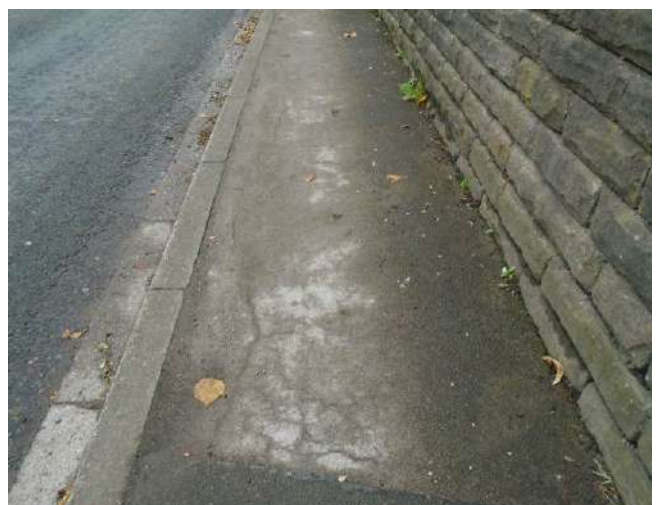
48. Cracked and splits within tarmacadam surface to pavement.
