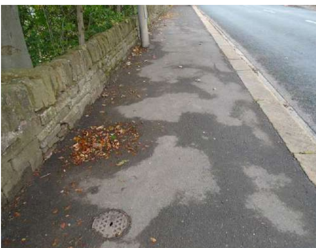
167. View of tarmacadam footpath. Recesses/uneven surfacing evident where leaves and soiling have accumulated.
