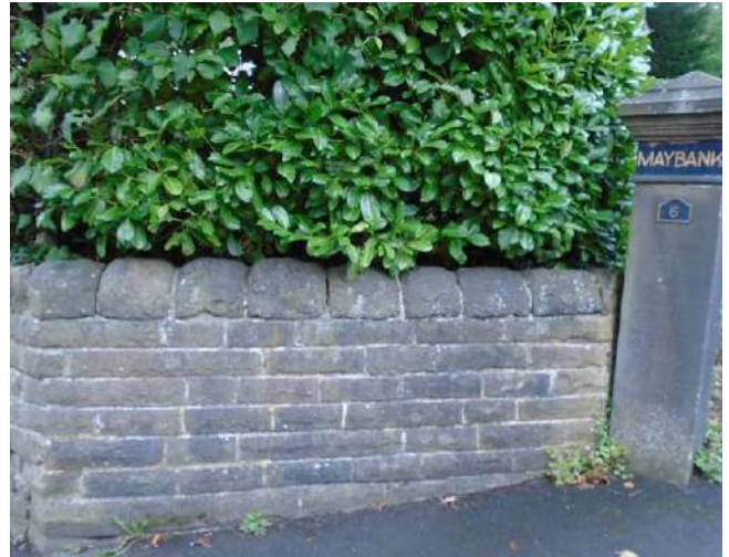
20. View of return wall to May Bank Villas. Open joint between gatepost and wall. Gatepost is leaning.
