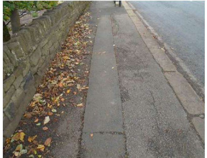
188. Splits/cracks and scarring of tarmacadam surface.
