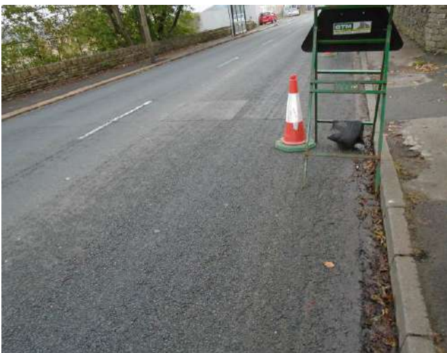
95. Erosion to road surface.
