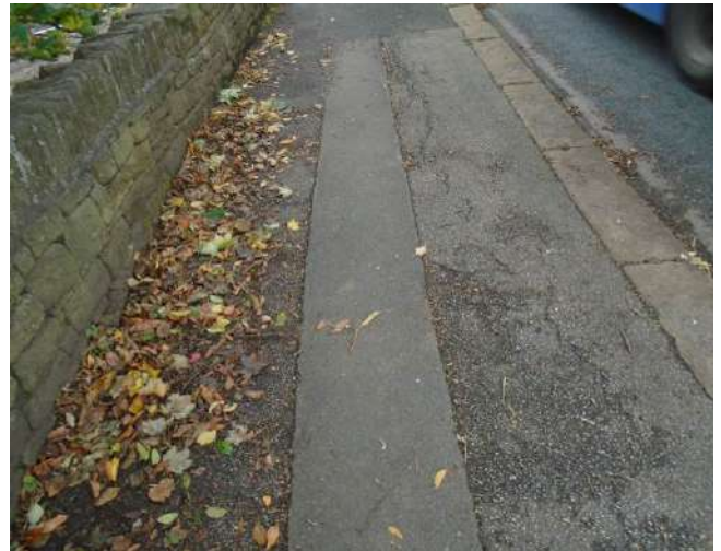
190. Scars and splits/cracks to tarmacadam surface. Paving is uneven approaching bus shelter.
