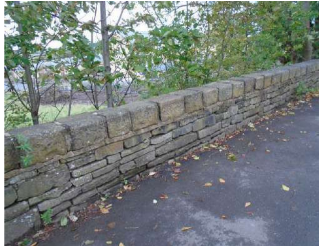
236. Dry stone wall to boundary of development site. Mortar bedding to copings locally cracked/defective.
