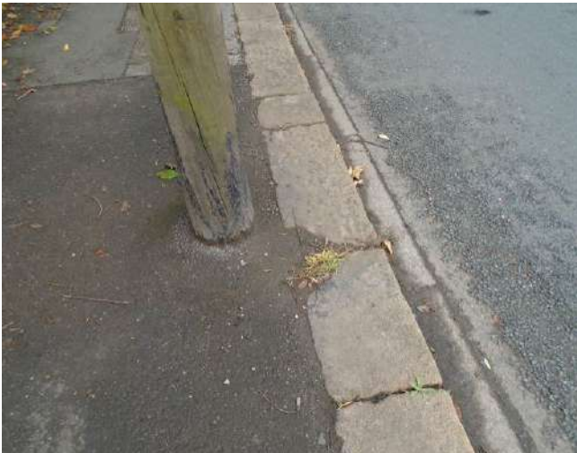
183. Cracked and split kerb stones adjacent to telegraph pole. Vegetation growth present to kerb stones.
