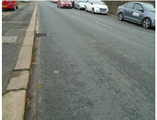
134. Worn surfacing to roadway.
