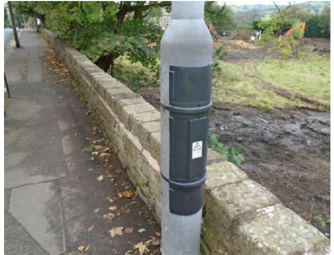
272. Non-matching inspection cover to lamp post.
