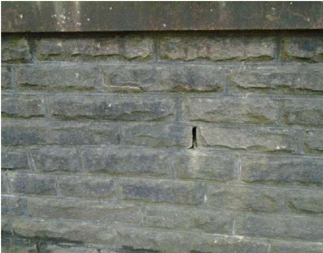
7. Defective mortar joint.
