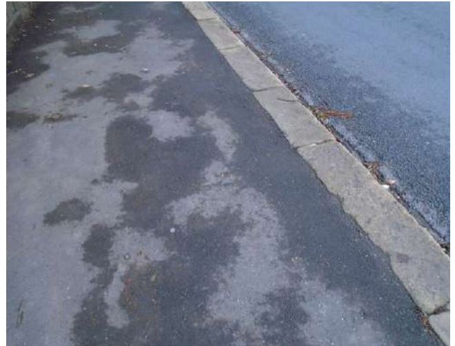
164. Wear/erosion to kerb stones.
