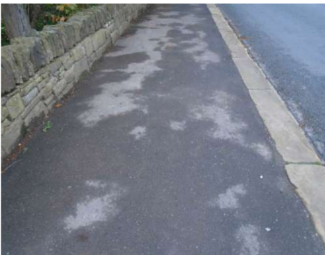
161. View of tarmacadam footpath. Erosion and wear to kerb stones.
