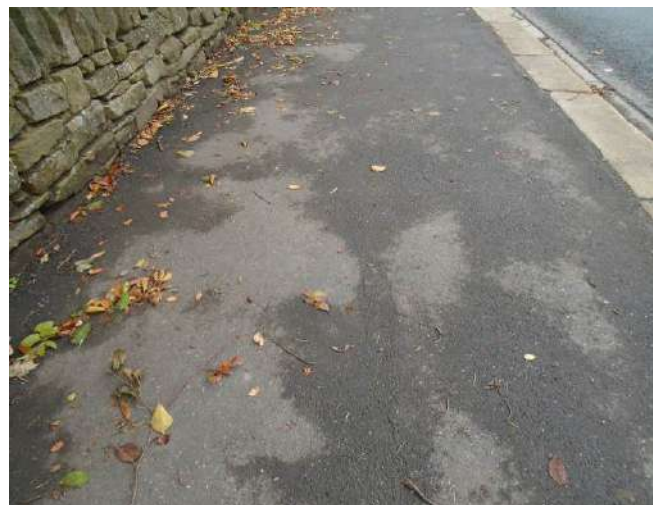
174. Surface of footpath uneven approximately centrally to width of footpath.
