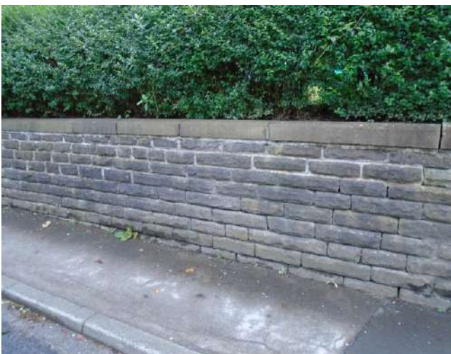
11. View of boundary wall, localised areas of open and defective mortar joints.
