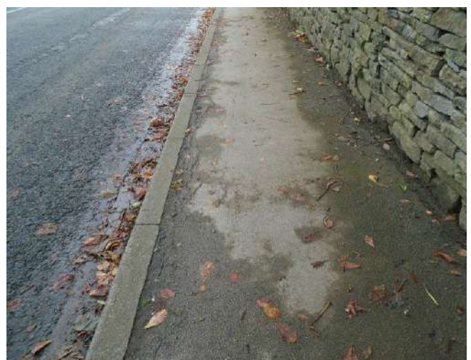
72. Isolated areas of cracking present to pavement. Edge of pavement uneven along kerb stone line.
