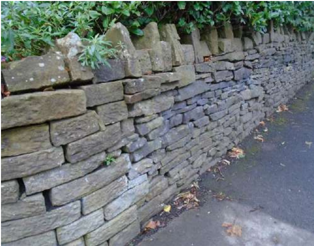
25. View of dry stone wall. Various areas of displacement of stones present. Wall leans and has various indentations.
