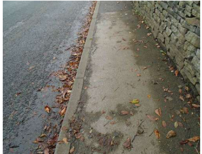
74. Isolated areas of cracking present to pavement. Edge of pavement uneven along kerb stone line.
