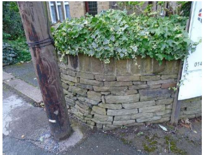
220. View of dry stone wall boundary to 'Wynncliff'. Isolated areas of mortar present mainly along copings, cracked and defective in areas.
