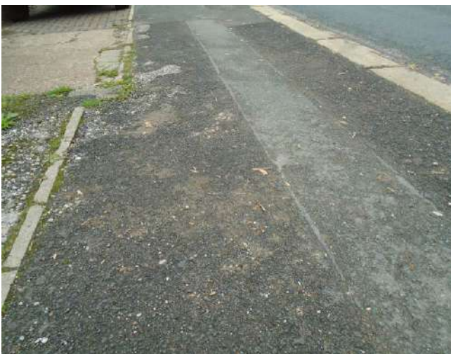
215. Worn tarmacadam surfacing to footpath. Surfacing is uneven and aggregate is exposed.
