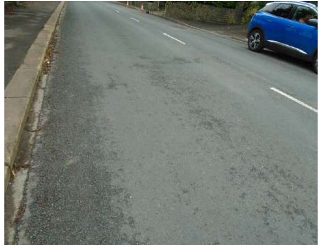
116. Erosion and wear to surface of tarmacadam roadway.
