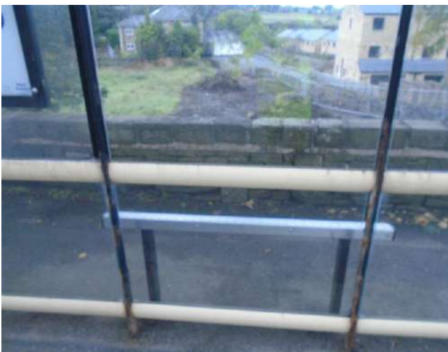
269. Corrosion to frame members of bus shelter.
