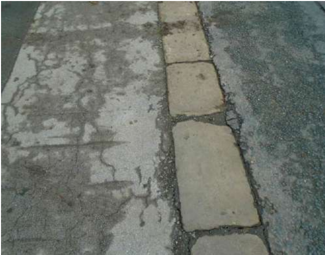
151. Cracked kerb stones at entrance into development site.
