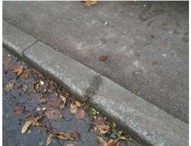
50. Example of cracking and damage to kerb stone.
