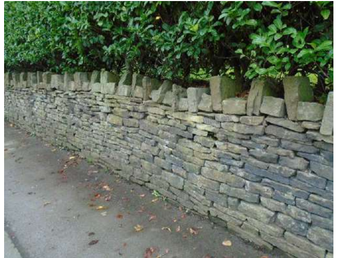
32. Dry stone wall. Numerous loose and defective stones present.
