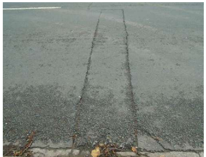
114. Cracking adjacent to, and worn joints to perimeter of, patch repair.
