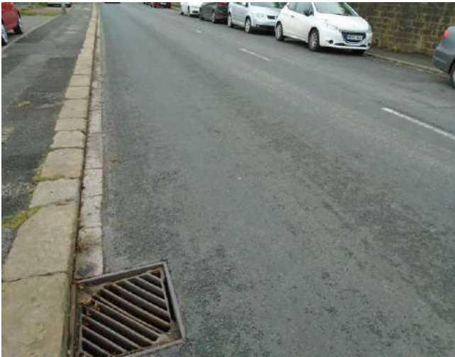
135. Worn surfacing to roadway.
