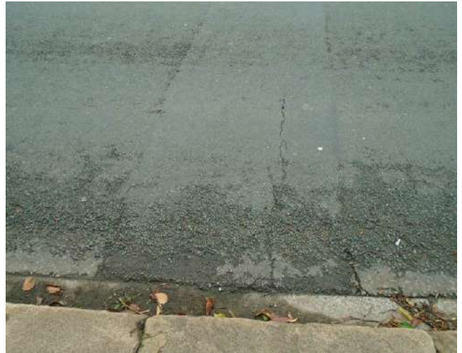
122. Cracks and splits to tarmacadam to patch repair.
