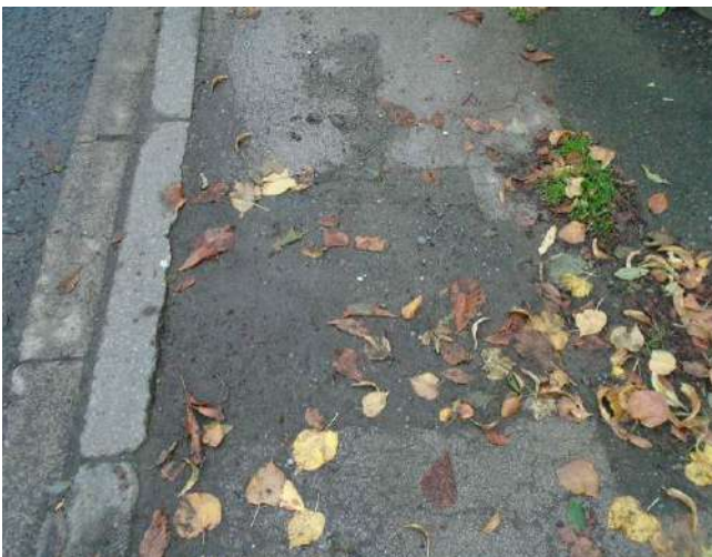
65. Previous patch repair. Surface of footpath uneven and locally eroded.
