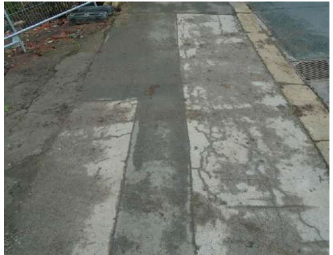
154. Cracking to tarmacadam. Patch repairs also present.
