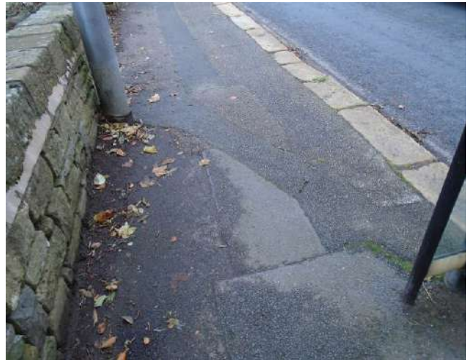
196. Various ages of tarmacadam present to footpath adjacent to bus shelter.
