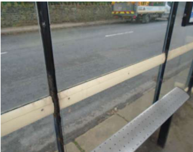
261. Corrosion to frame members to bus shelter.
