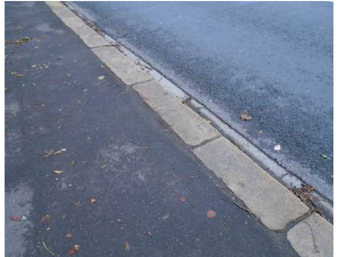
176. Worn, eroded and disturbed kerb stones.
