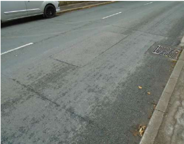
81. Patch repairs and scarring to road surface/joints.
