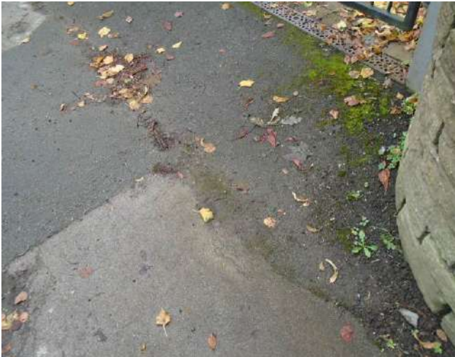
61. Damage to tarmacadam joints to areas of patch repair.
