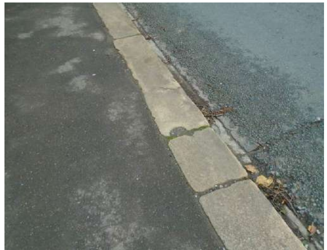
160. Eroded kerb stones.
