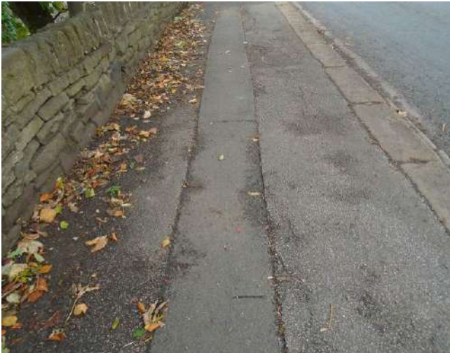
187. Splits/cracks and scarring of tarmacadam surface.
