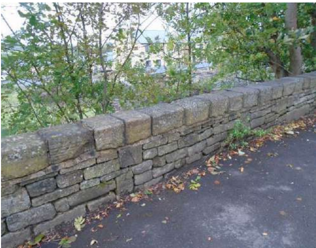
237. Dry stone wall to boundary of development site. Vegetation growth present to wall. Mortar bedding to copings locally cracked/defective.
