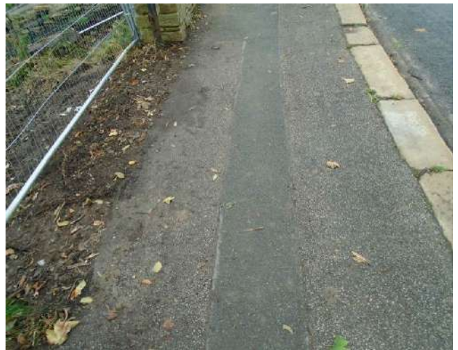
202. Tarmacadam surface to footpath with patch repaired section present centrally to pavement.
