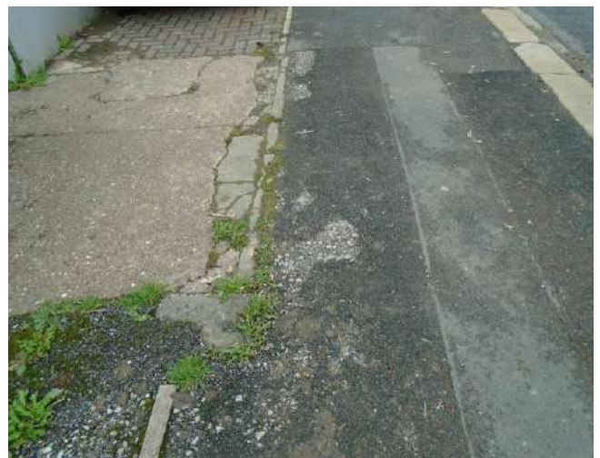
216. Worn tarmacadam surfacing to footpath. Surfacing is uneven and aggregate is exposed.
