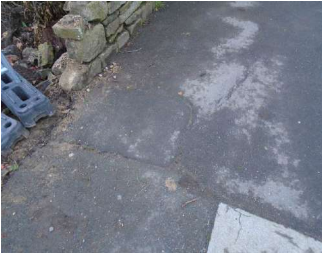
157. Patch repair to tarmacadam adjacent to development site entrance. Uneven area of tarmacadam present where various ages of tarmacadam abut.
