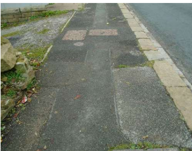
209. Uneven, disturbed and worn tarmac surfacing including patch repairs within entrance area into property adjoining development site, 'Glen View'.
