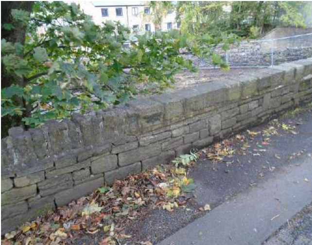
241. Dry stone wall to boundary of development site. Mortar bedding to copings.
