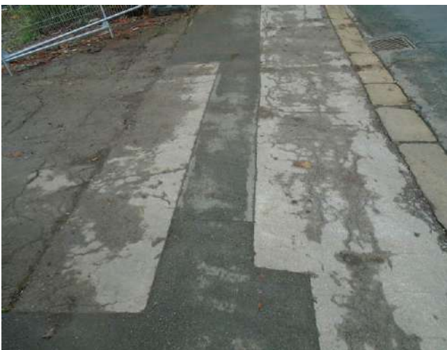
149. Cracking and patch repairs to tarmacadam.
