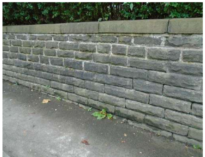
12. Eroded mortar joints to boundary wall.
