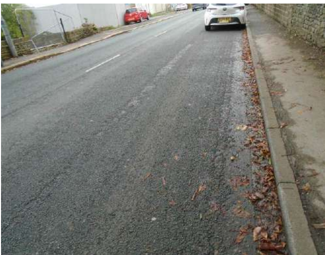
101. Worn/eroded surfacing to tarmacadam.
