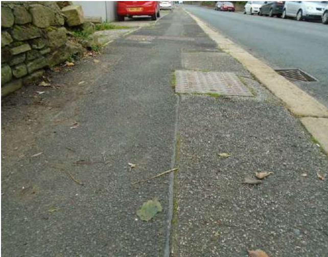
205. Uneven surfacing around inspection chamber.
