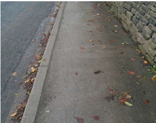
69. Cracking to tarmacadam surface of pavement. Edge of pavement uneven along kerb stone line.
