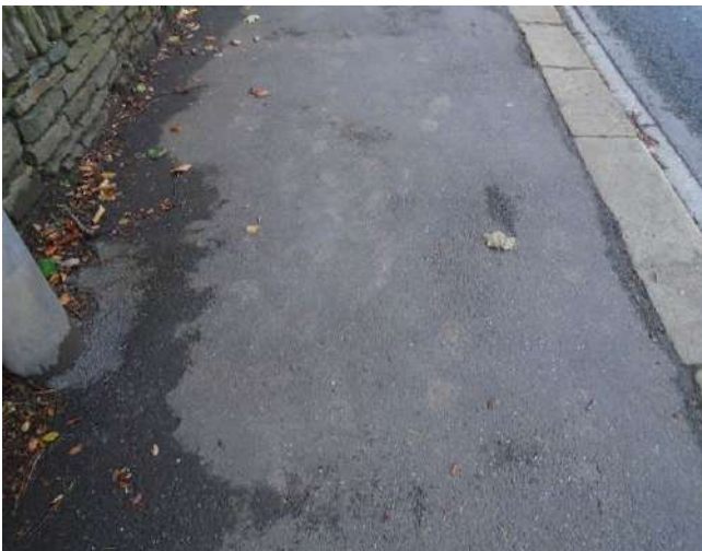
171. Isolated areas of scarring and cracking to tarmacadam surface adjacent to lamp post.
