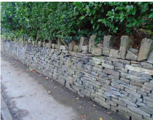
35. Dry stone wall. Numerous loose and defective stones present.
