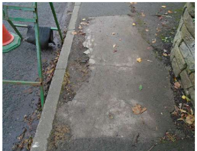
60. Damaged/defective tarmacadam adjacent to drop kerbs to number 6A. Tarmacadam is damaged adjacent to kerb stones and boundary wall, damage present to both sides of footpath.
