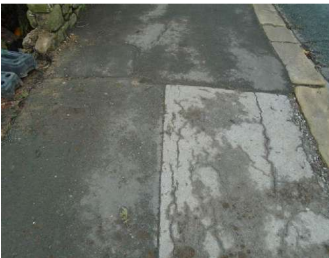
155. Cracking and splits to tarmacadam surface of pavement. Patch repairs also evident.
