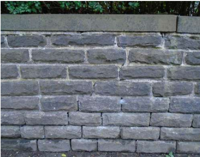
15. Cracking to mortar joints to boundary wall.
