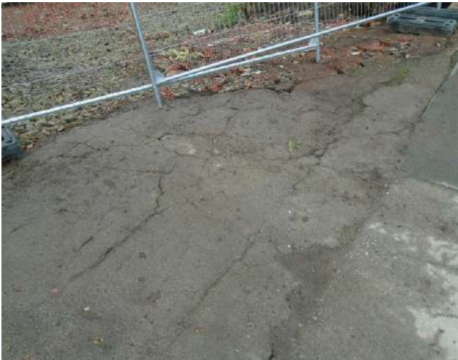
153. Cracking to tarmacadam in recessed entrance to development site.
