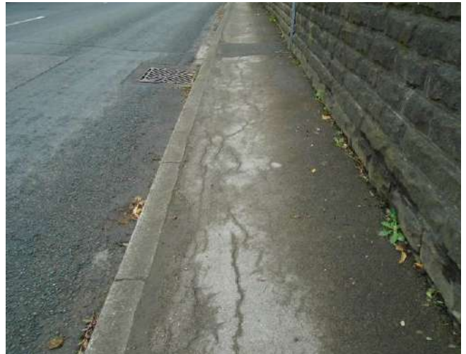
46. Cracks and splits to tarmacadam surface.
