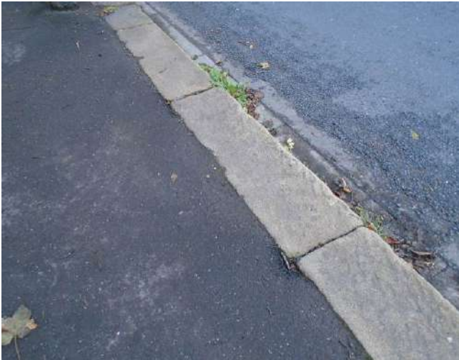
181. Erosion of edges of footpath adjacent to telegraph pole.
