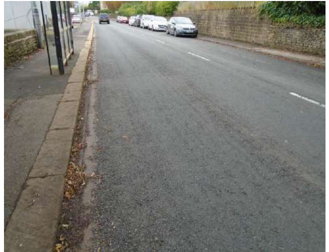
128. Erosion to tarmacadam surfacing.
