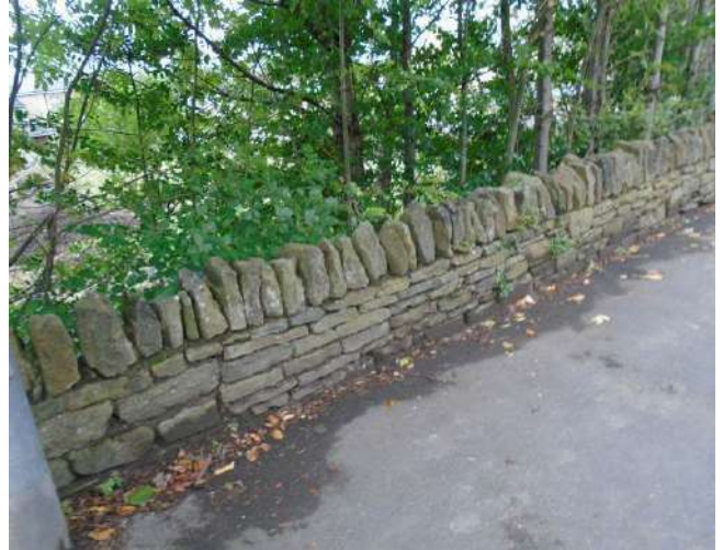
230. View of dry stone boundary wall. Vegetation growth present to wall.
