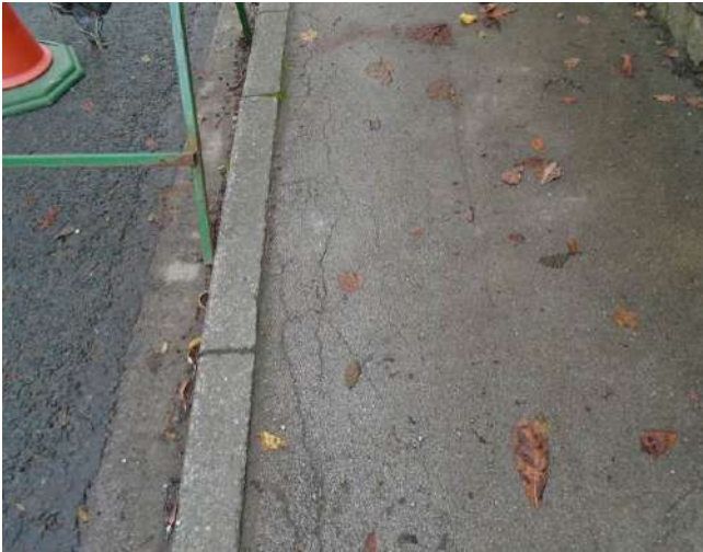
67. Cracking to tarmacadam surface of pavement. Edge of pavement uneven along kerb stone line.
