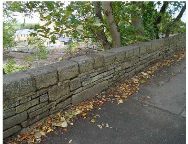
238. Dry stone wall to boundary of development site. Mortar bedding to copings locally cracked/defective.
