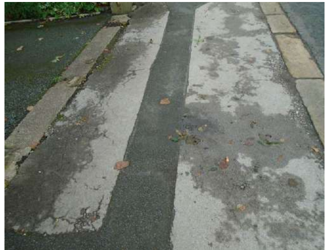
142. Patch repair in front of 'Wynncliff'. Section of uneven paving present where standing water is evident.
