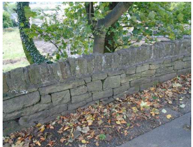
240. Dry stone wall to boundary of development site. Mortar bedding to copings locally cracked/defective.
