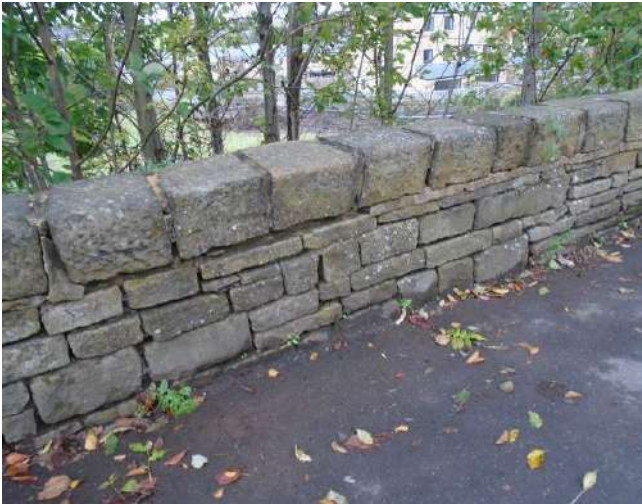
235. Dry stone boundary wall to development site. Isolated sections of mortar bedding to copings. Mortar bedding defective.
