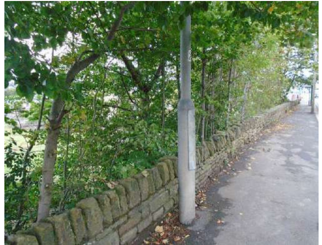
250. View of base of lamp post. Lamp post is slightly out of plumb, leaning inwards towards the development site by approximately 2 degrees.
