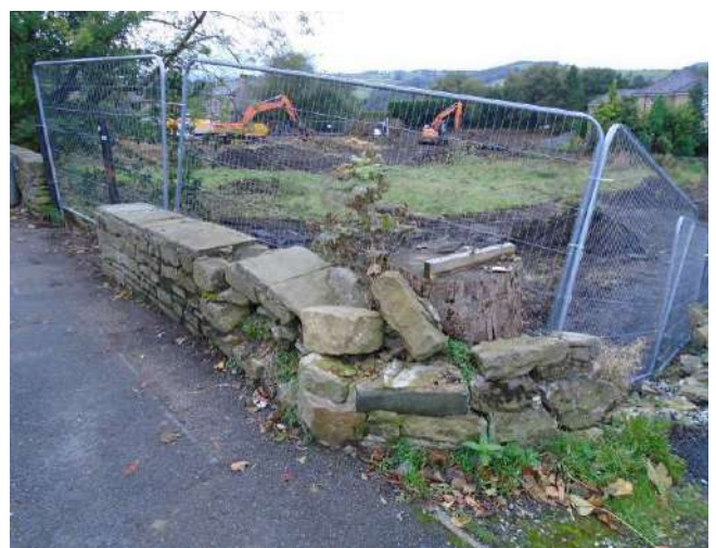
246. Damaged/collapsed wall to boundary of development site at return to property adjoining development site, 'Glen View'.
