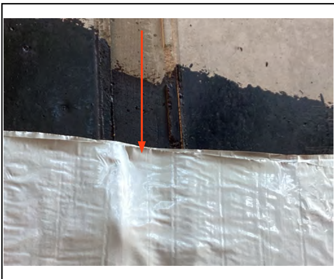
Slight groove within retaining wall to be aware of when sealing GRSAM
