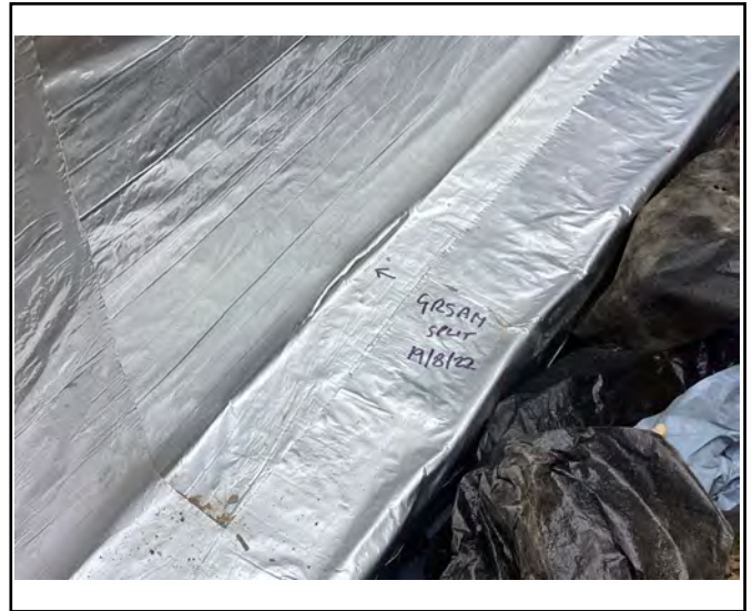
Area of damage (1) following a
