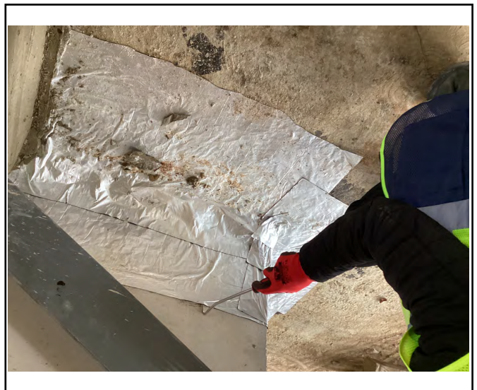
View showing pipe penetration which may prove difficult to seal.
