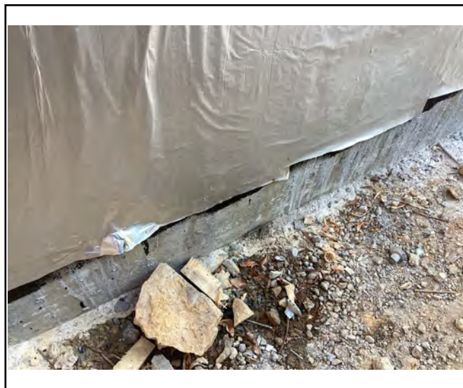
Loose edges of GRSAM remediated during verification visit
