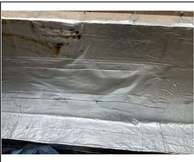
View of one of two areas of GRSAM where the substation wall incomplete
