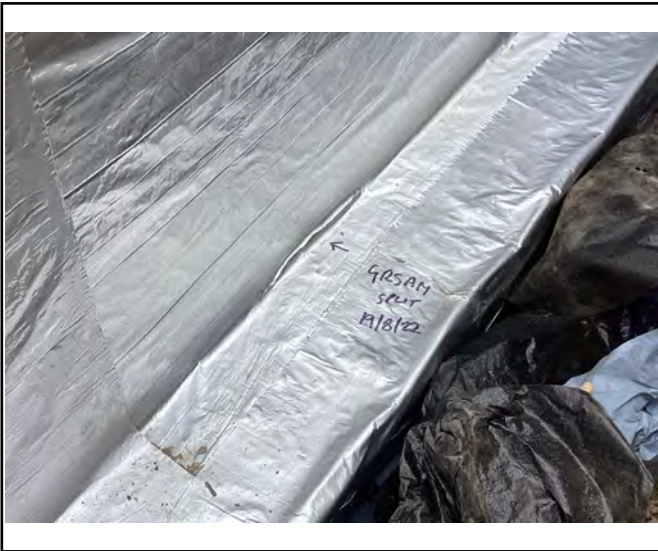
Area of damage (1) where the
