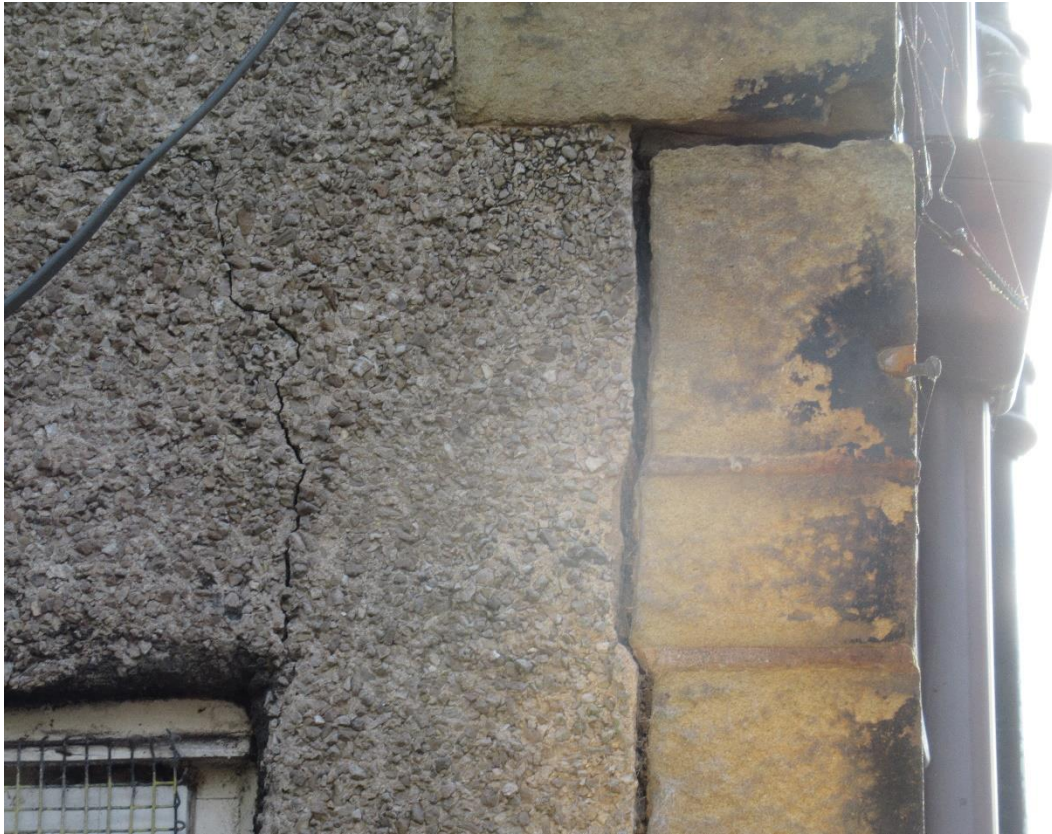
Photograph 11 – Gap between stone and render at northwestern corner of Building 1.
