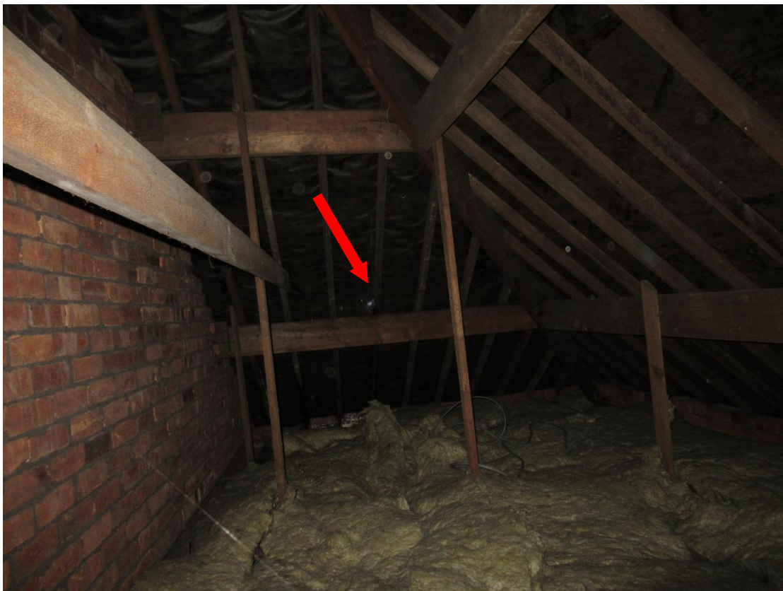
Photograph 16 – Light ingress from tear in bitumen felt in Loft Space 1 of Building 1.
