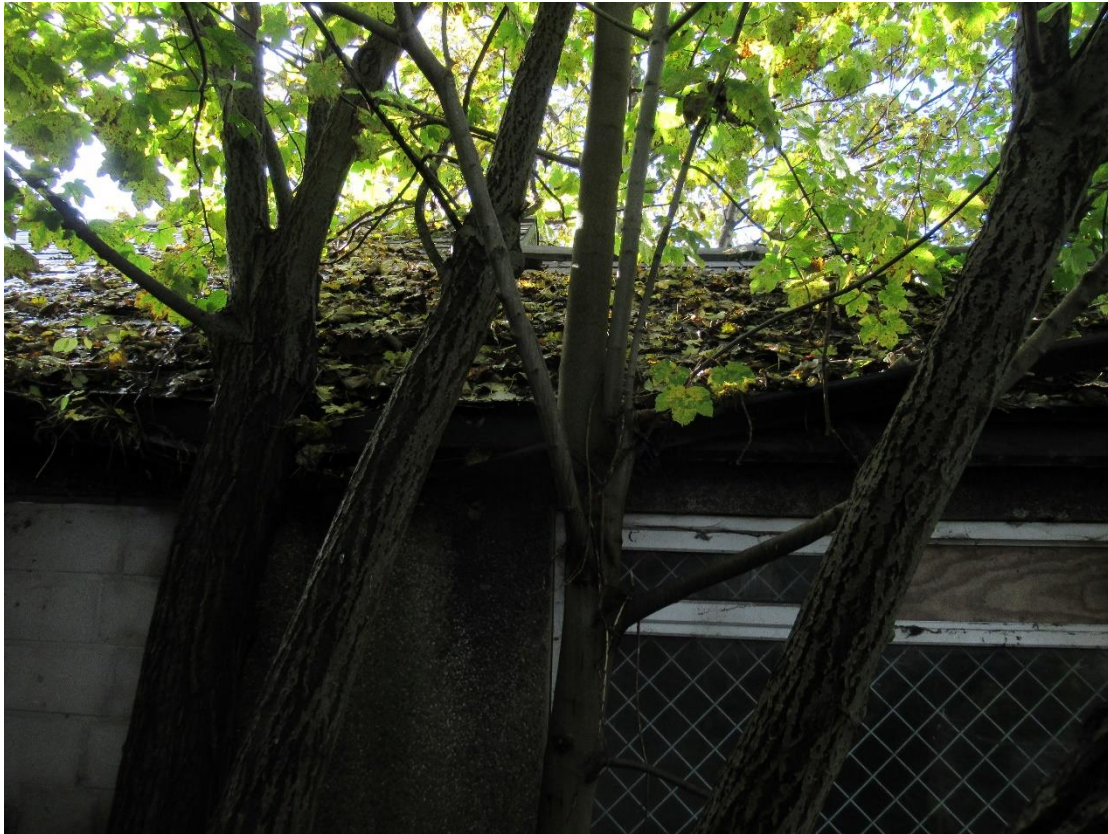
Photograph 37 – Damaged soffit box and roof from tree growth on Building 3.
