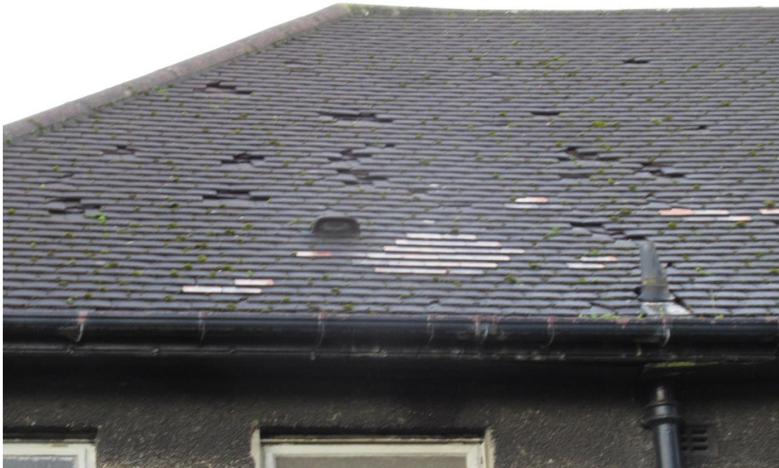
Photograph 7 – Example of missing roof tiles on Building 1.
