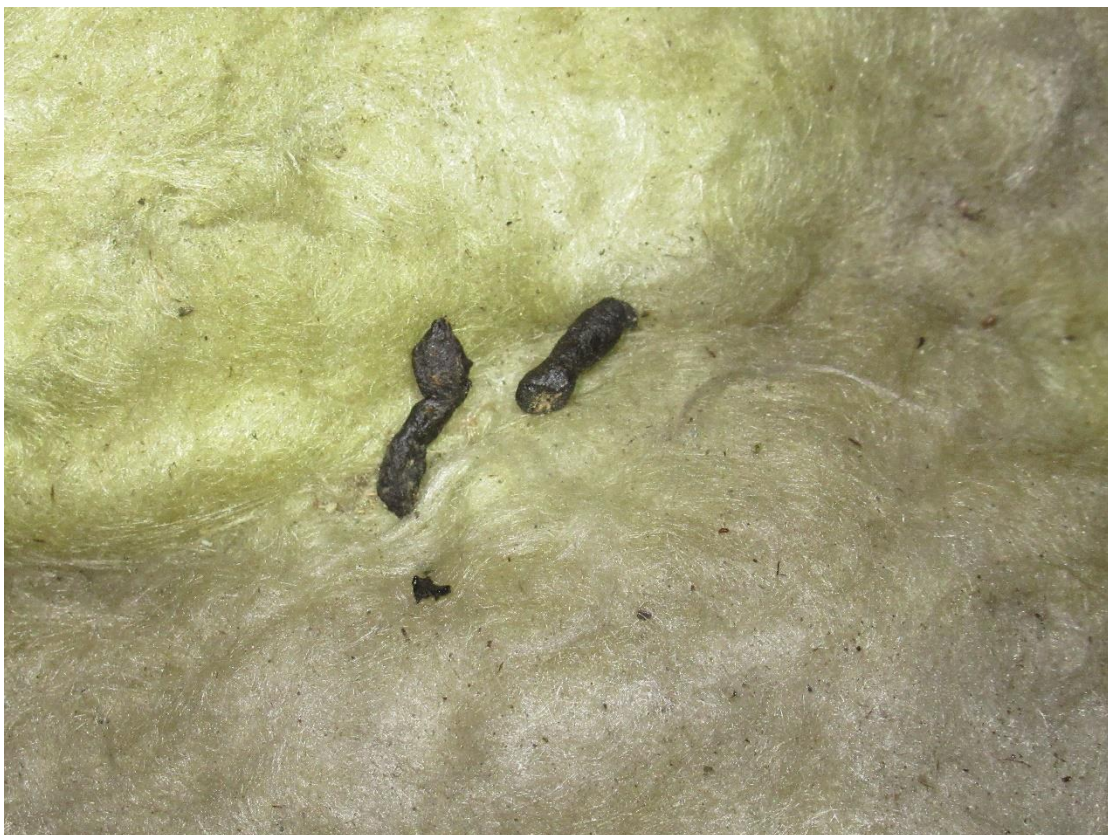
Photograph 14 – Rat droppings found in Loft Space 1 in Building 1.
