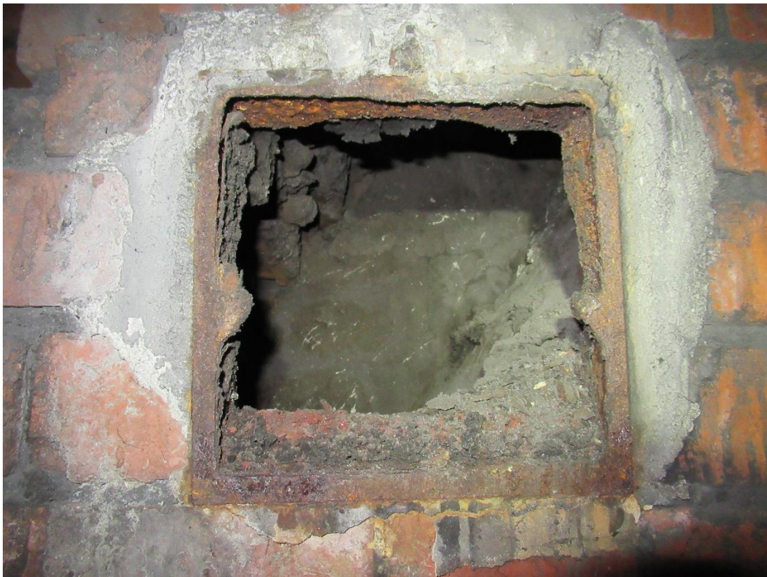
Photograph 24 – Hole into chimney in Loft Space 4 in Building 1.
