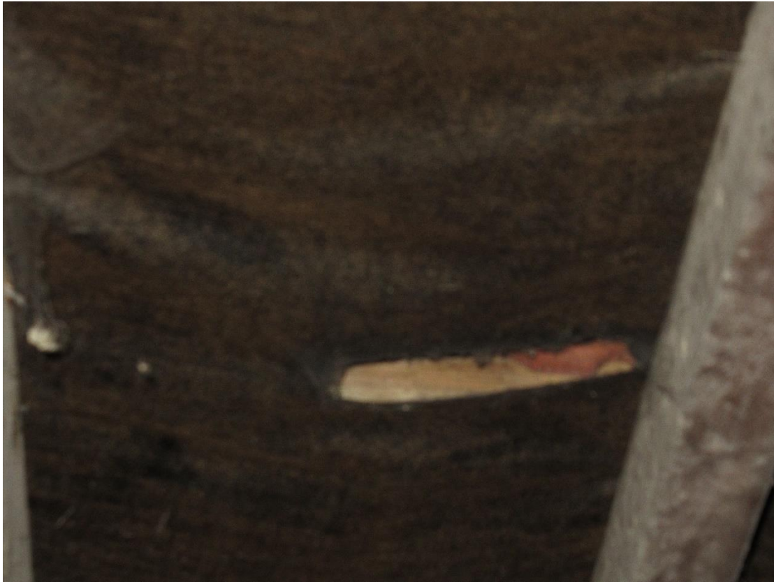
Photograph 21 – Tear in bitumen felt in Loft Space 3 in Building 1.
