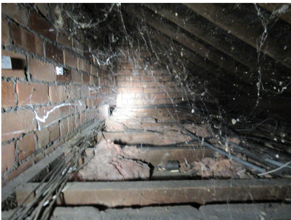
Photograph 40 – Heavily cobwebbed Loft Space 5 in Building 3.
