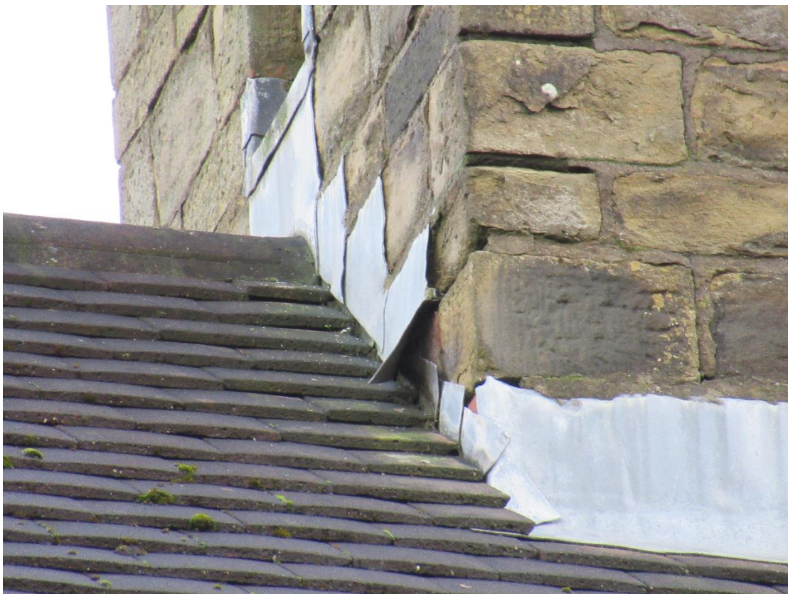
Photograph 8 – Raised flashing where chimney meets roof on Building 1.
