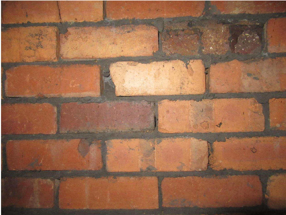
Photograph 15 – Example of gaps in mortar joints of brickwork found in loft spaces of Building 1.
