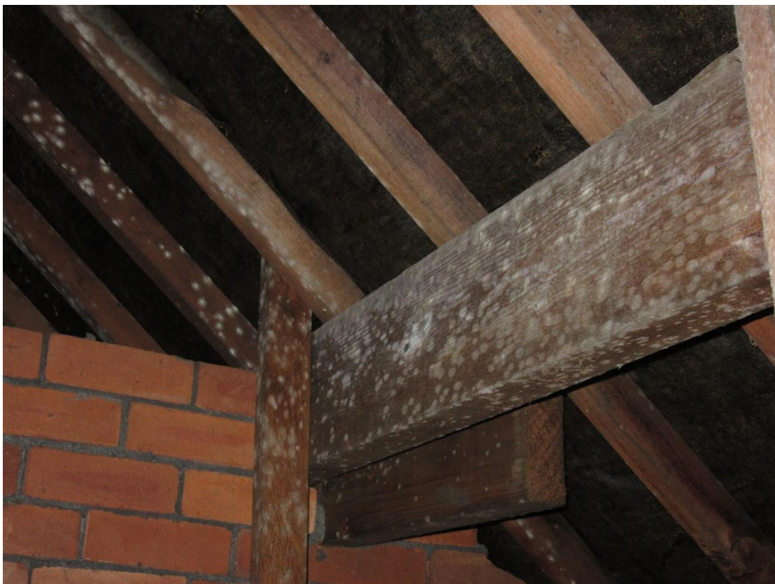
Photograph 22 – Mold on wooden beams in Loft Space 3 in Building 1.
