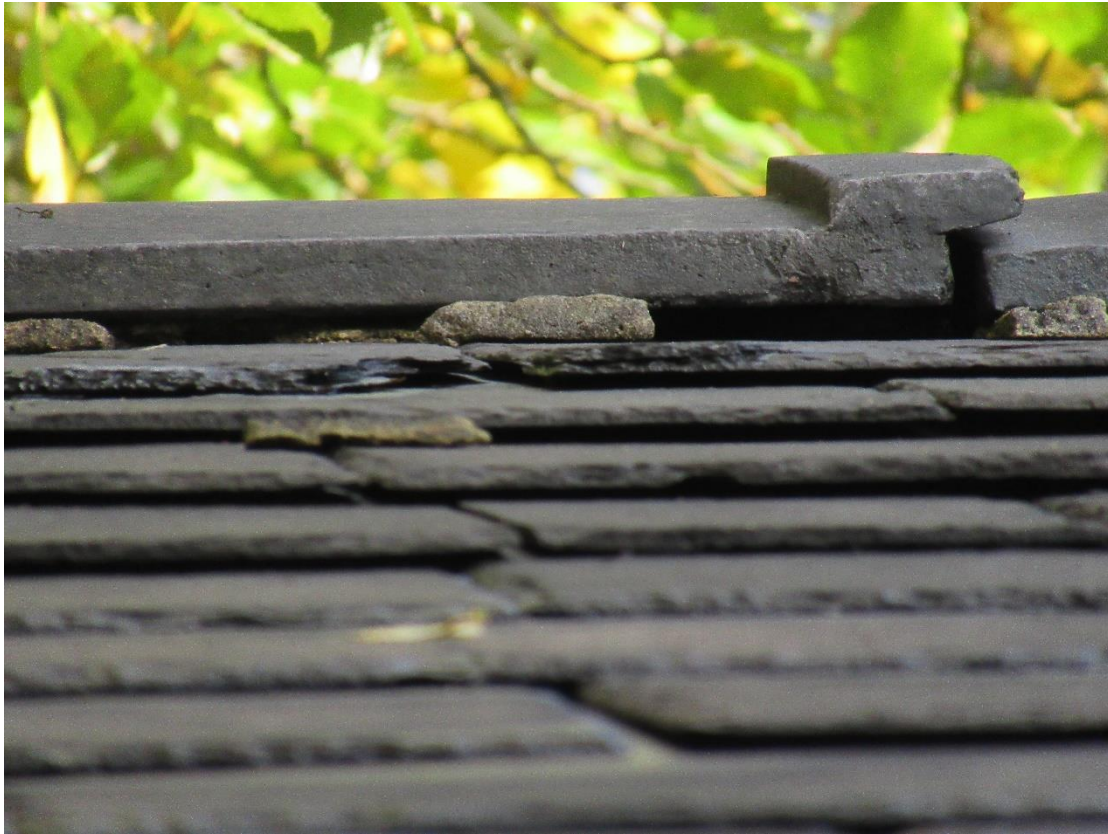
Photograph 33 – Gap under ridge tile on roof of Building 3.
