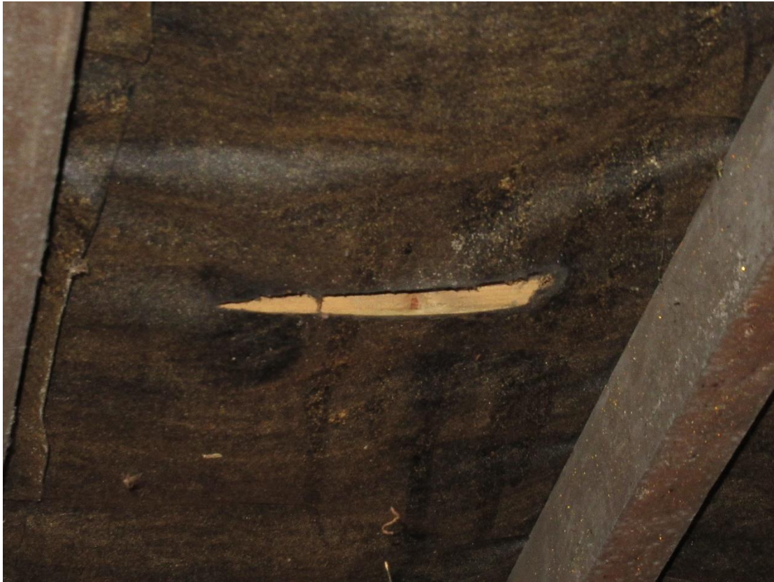
Photograph 25 – Tear in Bitumen felt in Loft Space 4 in Building 1.
