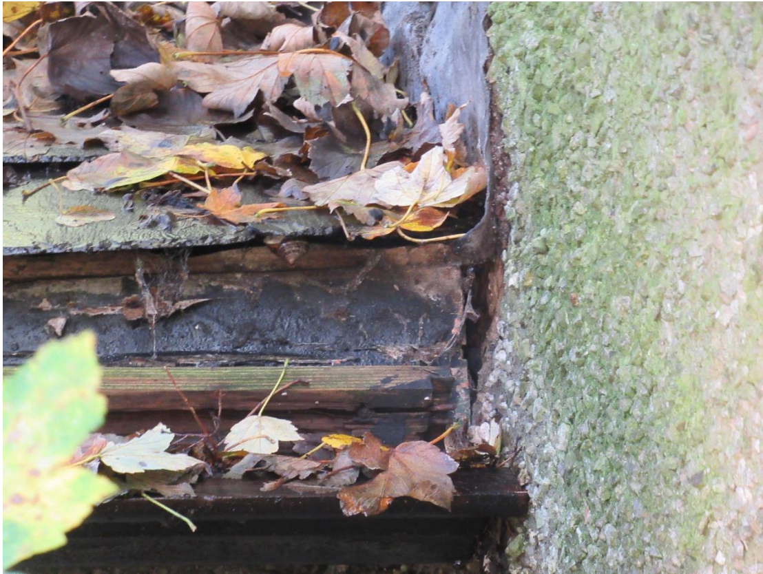
Photograph 35 – Gap between soffit box and wall on Building 3.
