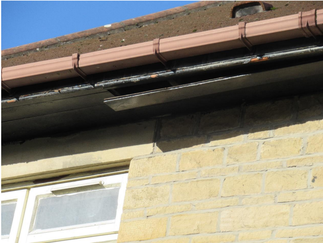
Photograph 9 – Example of gap in soffit box on Building 1.
