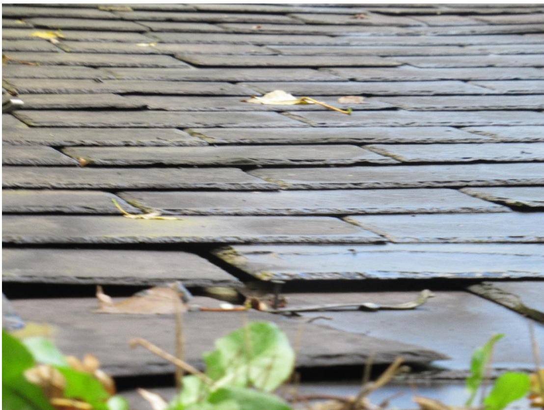
Photograph 34 – Raised roof tiles on roof of Building 3.
