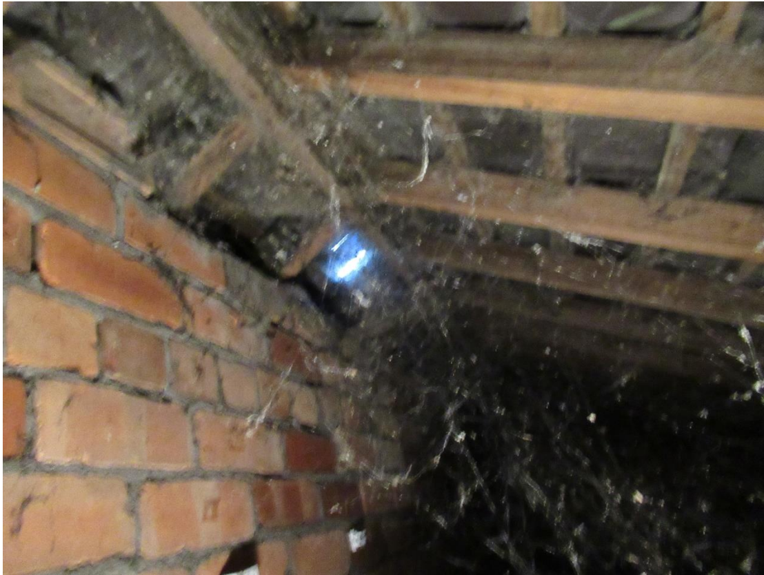
Photograph 41 – Light ingress seen within Loft Space 5 in Building 3.
