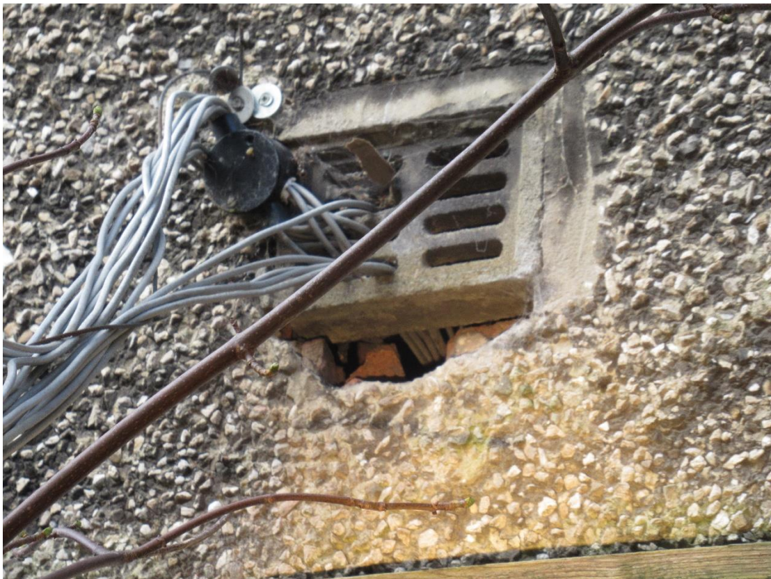
Photograph 38 – gap under grate on wall of Building 3.
