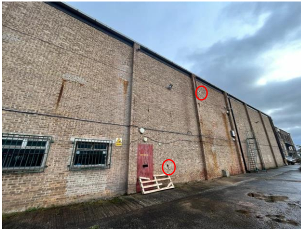
Photo 1: The southern aspect of the building. Missing brick circled.
