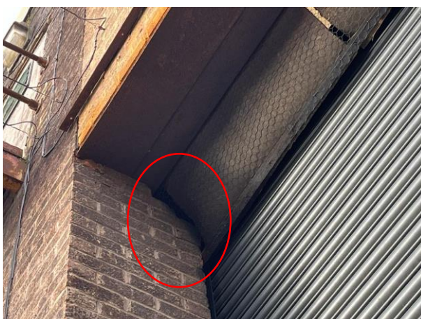
Photo 5: Gap under the roller door.
