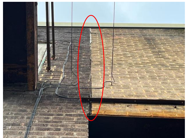
Photo 4: Areas of missing mortar around additions/ renovations to the building.
