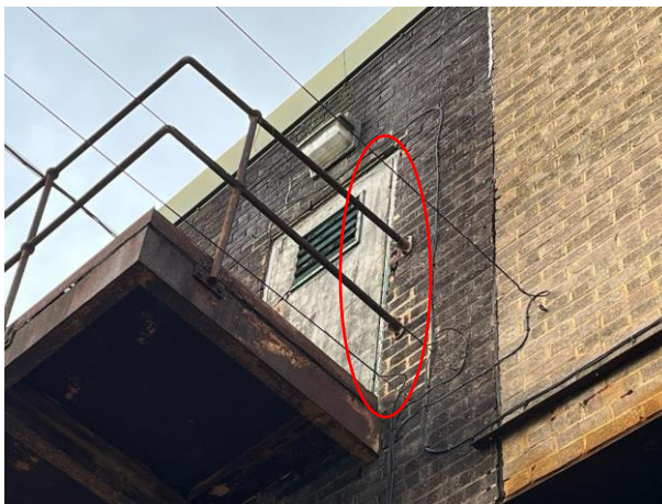
Photo 3: The doorframe on the eastern aspect of the building with significant amounts of missing mortar, as circled.
