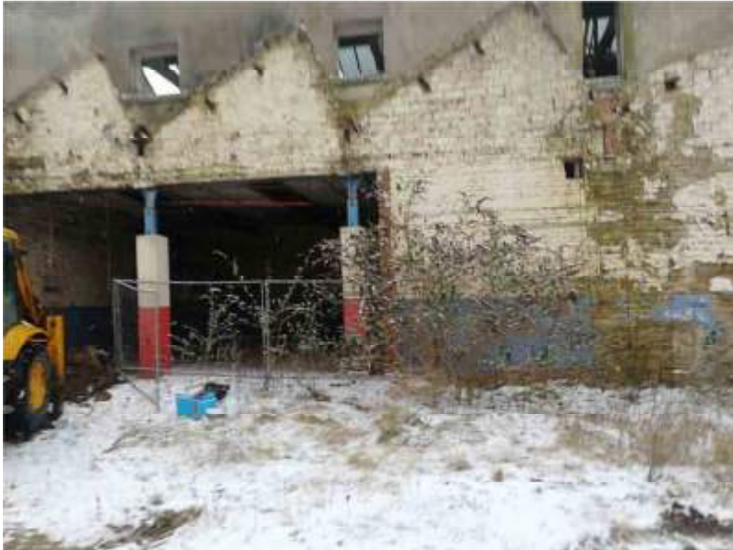
Photograph 14: Large dilapidated building in Area A.
