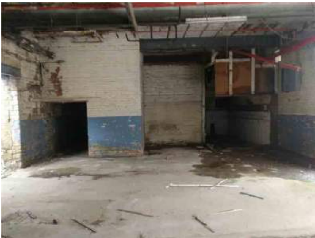
Photograph 15: Inside the dilapidated building in photograph 14.
