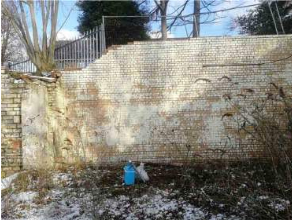
Photograph 18: Retaining wall at northern boundary of Area B (above sandstone retaining wall in photograph 1).
