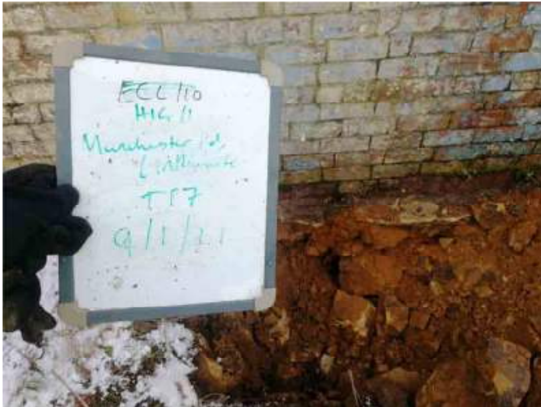
Photograph 8: Exposed foundations in TP7
