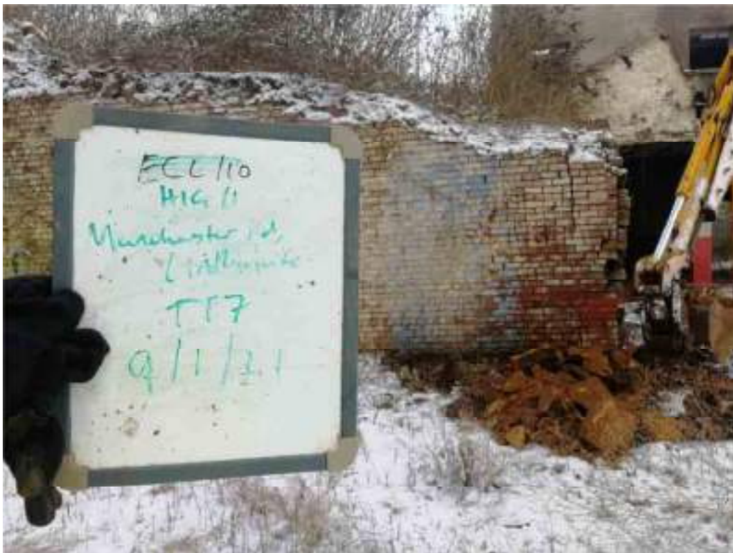
Photograph 7: Location of TP7 undertaken to expose foundations of brick retaining wall in photograph 6.
