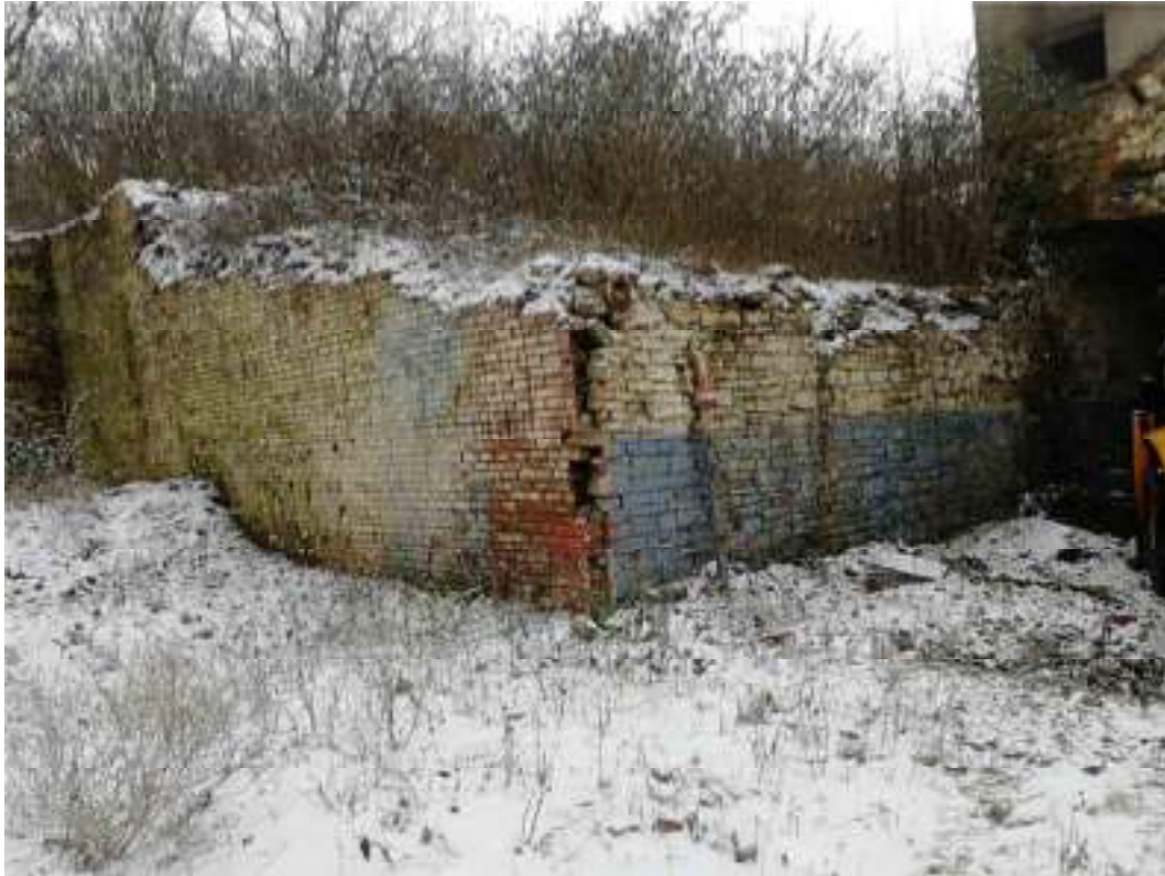
Photograph 6: Damage to the brick retaining wall. Photograph taken facing south.
