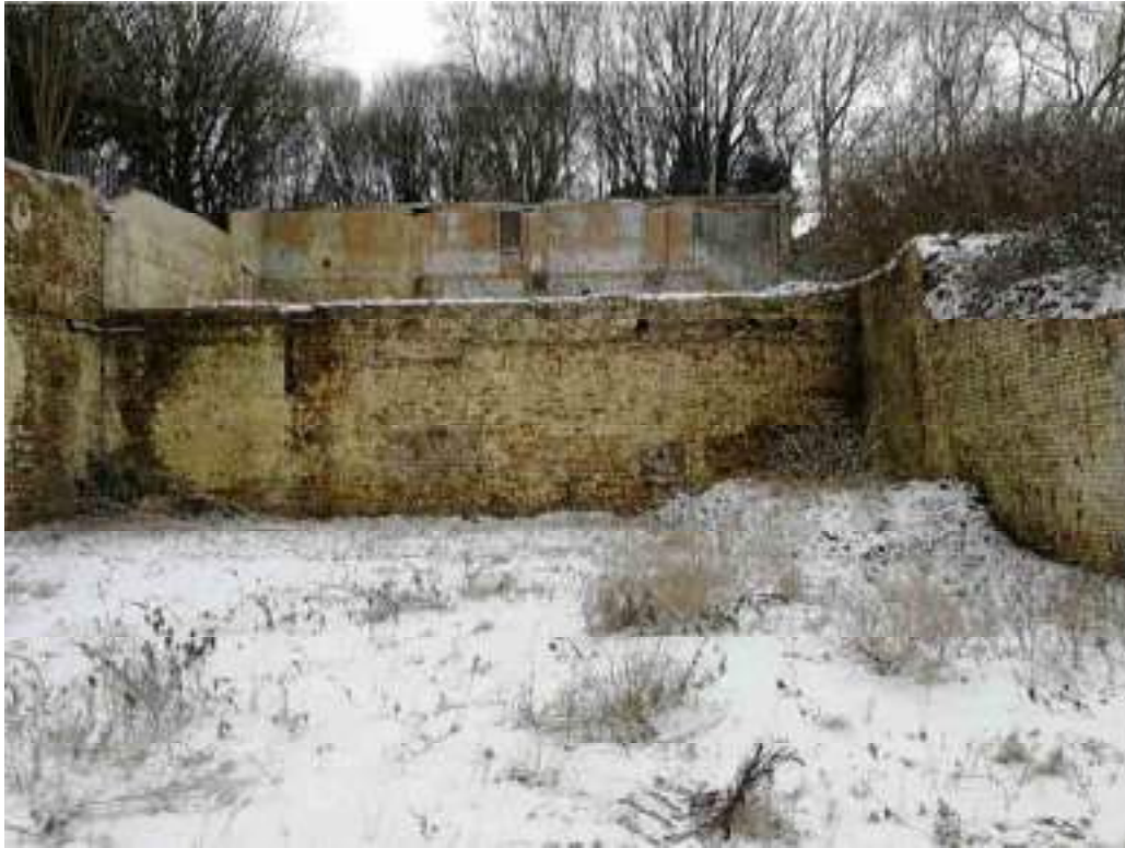
Photograph 1: Sandstone retaining wall in background, brick retaining wall to the right. Photograph facing south.
