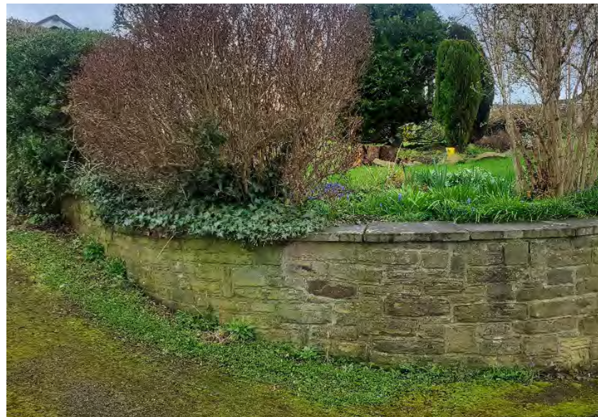
OVERGROWN DRIVEWAY AND SHARED WALL WITH 193
