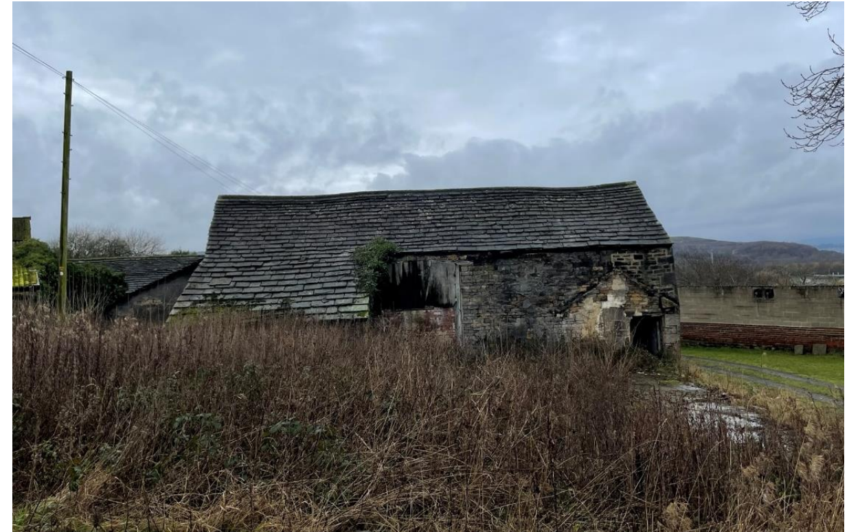
Figure 25 View of Stone Barn C from east showing listing of roof to south.
