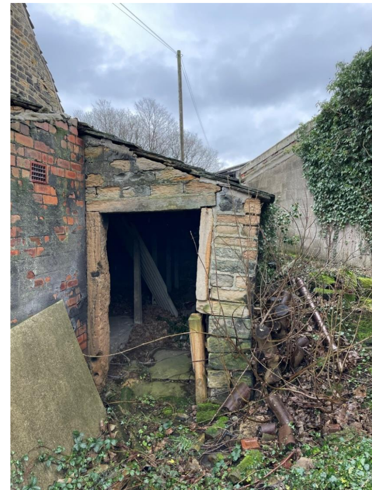
Figure 23 Distortion of south-west corner of southern extension, viewed from west with tree stub adjacent.
