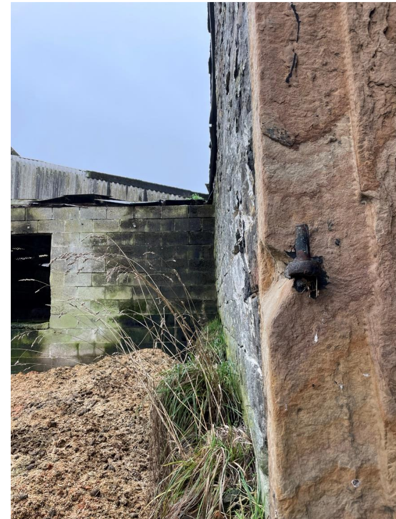
Figure 14 Distortion of east elevation, south of large opening.
