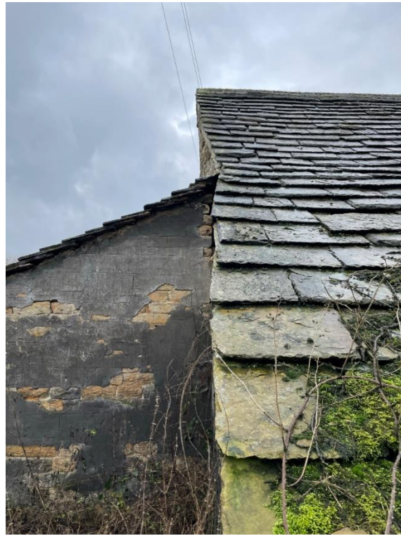
Figure 21 Distortion of south gable view from east.
