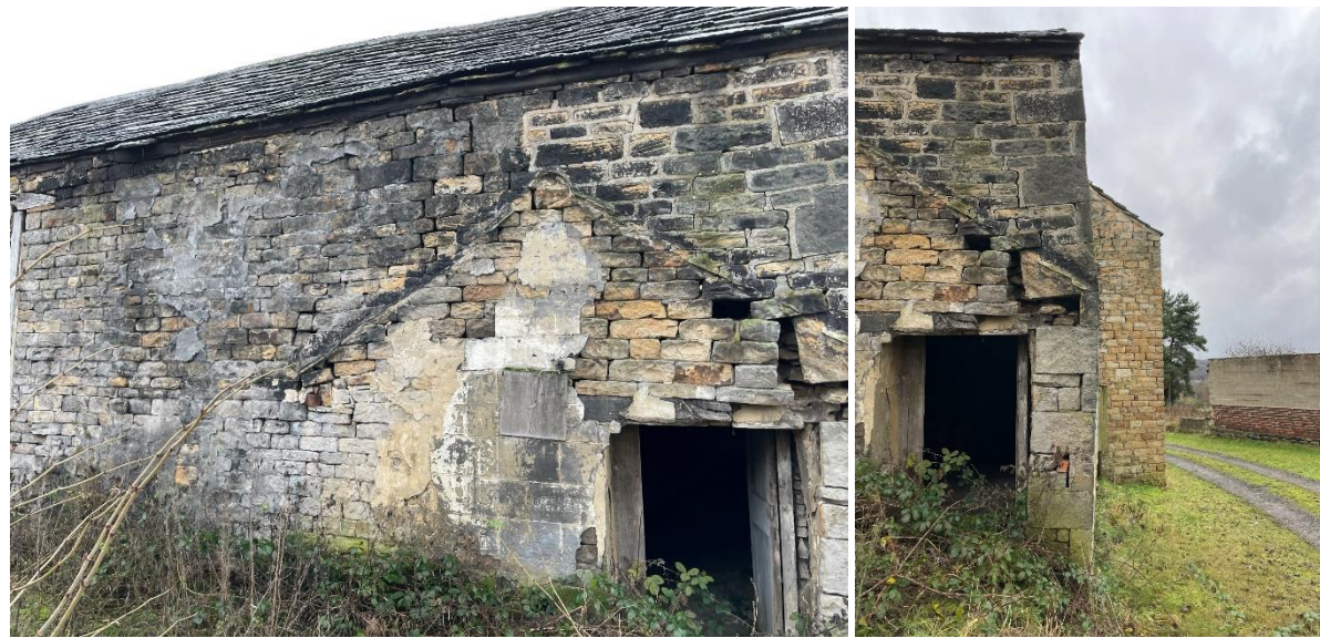
Figure 18 (a) North end of east elevation; (b) Distortion of north gable elevation.
