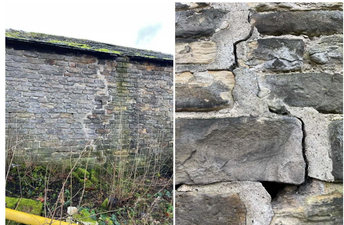
Figure 28 (a) Repointed crack to east elevation; (b) Cracking to repointed mortar joints.
