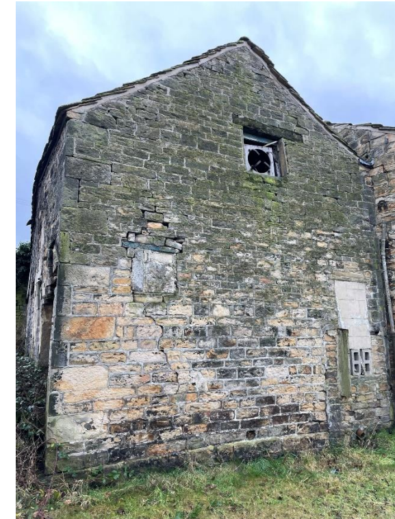
Figure 19 North gable elevation with cracking.
