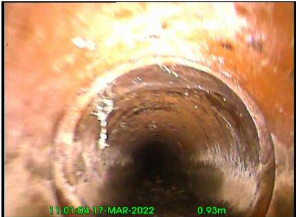
Photo: 5_7A 1.1m, Joint displaced, large
