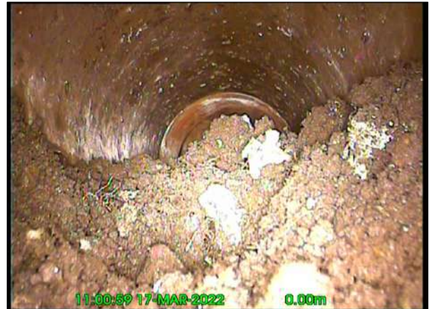
Photo: 5_3A 0m, Settled deposits, fine, 30% cross-sectional area loss, Start
