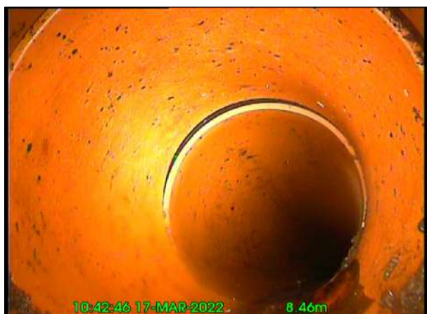
Photo: 2_11A 8.8m, Joint displaced, medium
