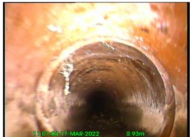
Photo: 5_6A 0.9m, Settled deposits, fine, 15% cross-sectional area loss, Start
