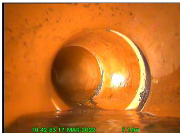
Photo: 2_10A 7.2m, Joint displaced, medium
