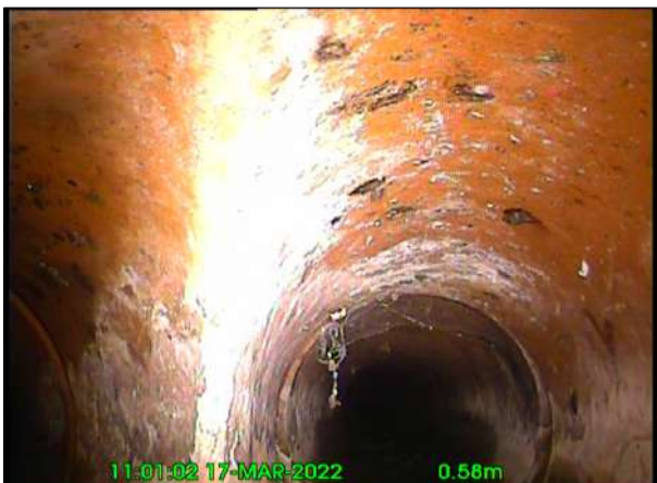
Photo: 5_4A 0.45m, Connection other than junction, at 9 o'clock, diameter 150mm
