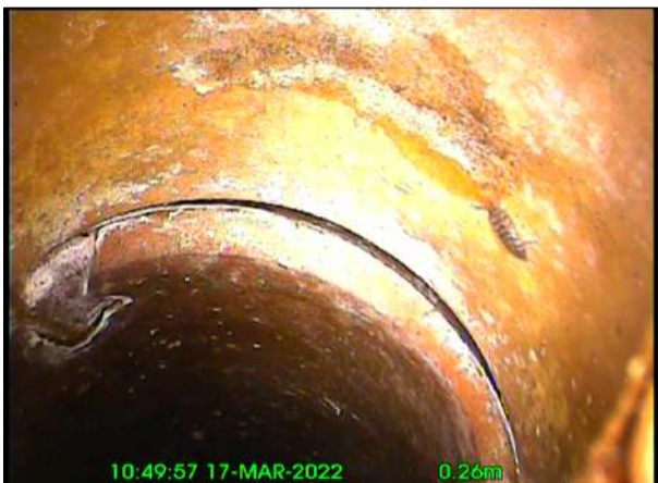
Photo: 4_4A 0.5m, Joint displaced, medium
