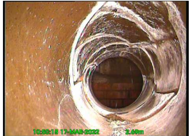
Photo: 4_8A 3m, Fracture, multiple at joint, from 9 to 5 o'clock, Start
