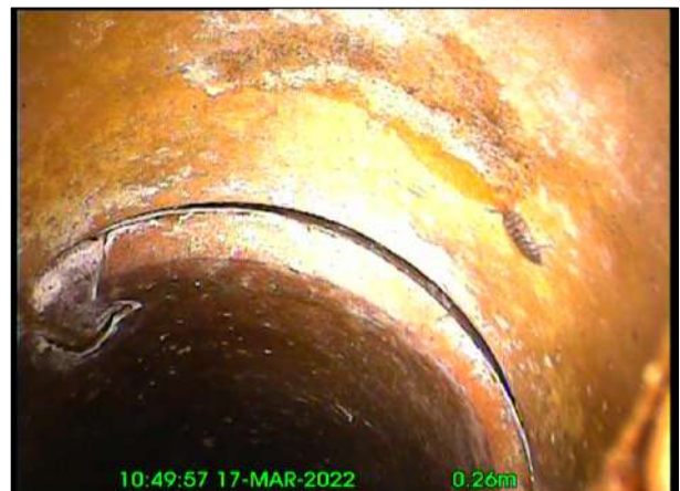
Photo: 4_5A 0.5m, Fracture, circumferential at joint, from 10 to 11 o'clock
