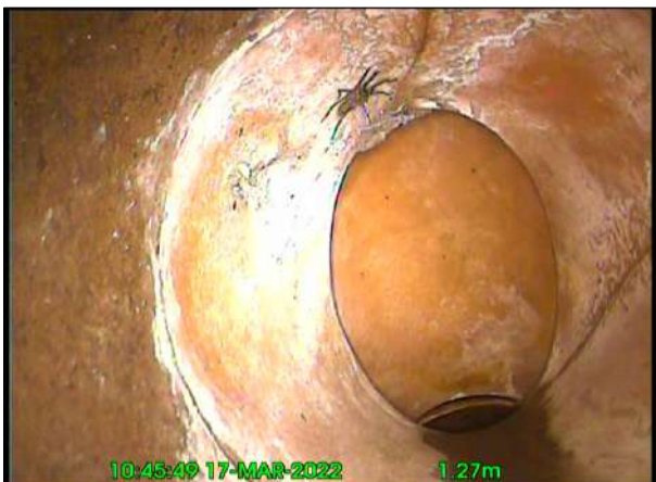
Photo: 3_4A 1.6m, Crack, circumferential at joint, from 12 to 3 o'clock
