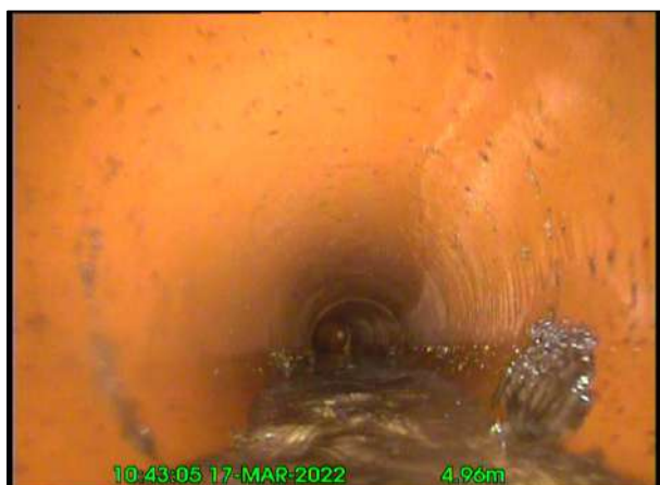
Photo: 2_7A 5m, Turbid water level, 20% of the vertical dimension
