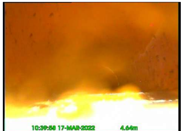
Photo: 2_6A 4.65m, Turbid water level, 20% of the vertical dimension
