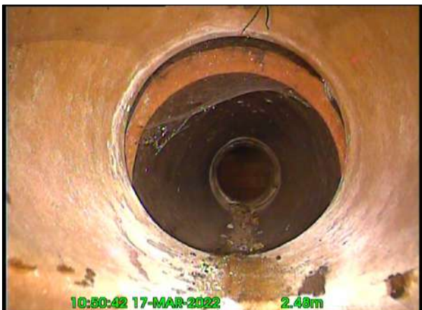
Photo: 4_9A 3.1m, Joint displaced, large
