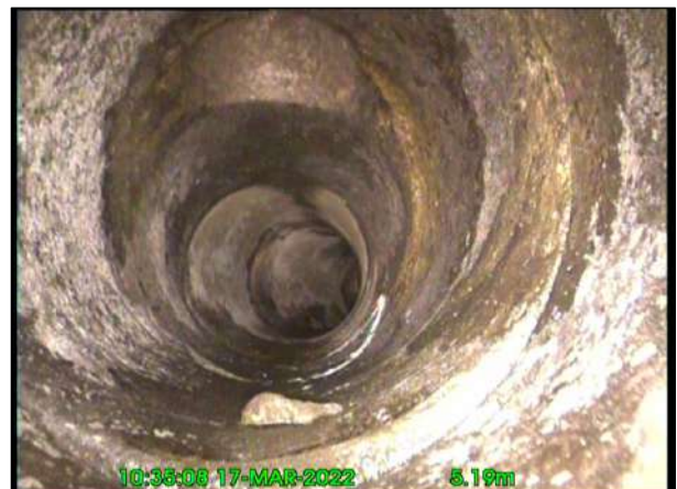
Photo: 1_5A 5.8m, Connection other than junction, at 12 o'clock, diameter 100mm
