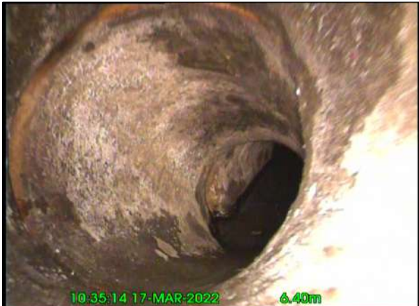
Photo: 1_6A 6.6m, Line deviates right
