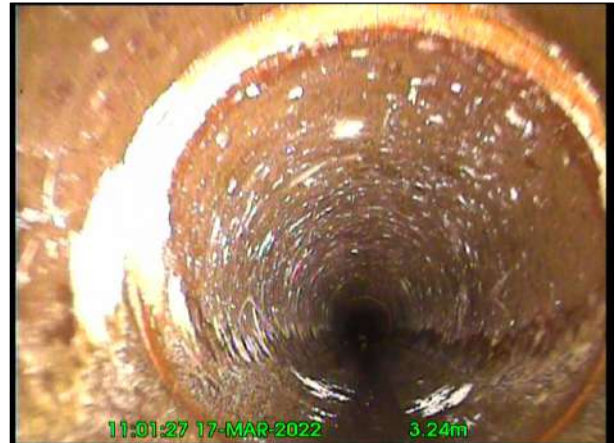
Photo: 5_9A 3.5m, Joint displaced, medium
