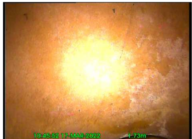
Photo: 3_5A 1.7m, Line deviates down
