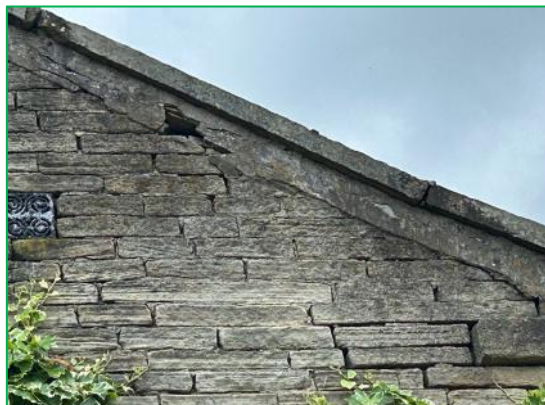
Showing crevices and holes in the stonework on the northeast elevation of the large barn
