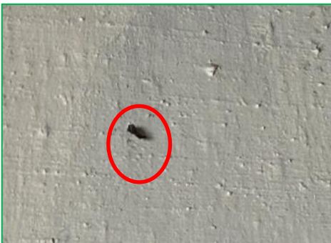
Bat dropping found on the northeast wall of the garage
