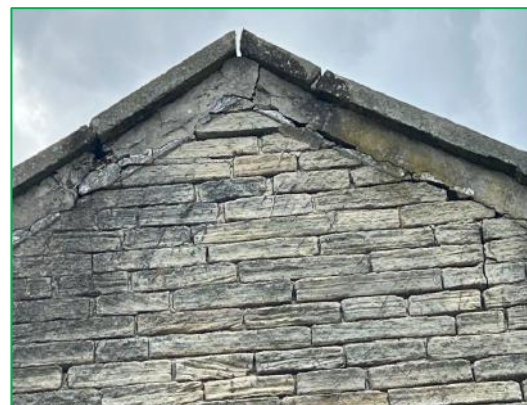
Showing crevices and holes in the stonework on the northeast elevation of the workshop and garage
