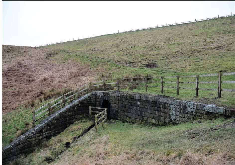
Plate 1. The Draw-off Culvert/Valve Tunnel at the base of the dam, looking south-west
