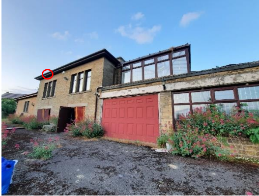
Photograph 1 – Emergence point on the western elevation, recorded on two separate occasions
