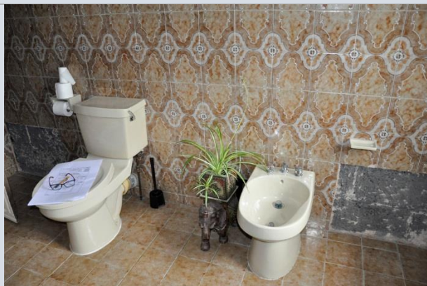
Figure 21: Removing modern bathroom tiles confirmed the presence of a modern blockwork wall with a void for services to the rear in the eaves void
