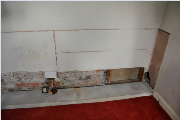
Figure 17: Blocked door opening in wall between existing study and pantry confirmed by removal of modern plasterboard
