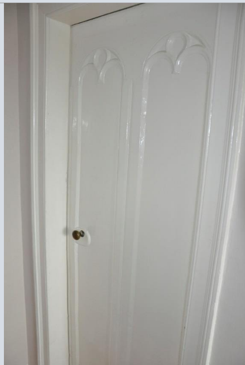
Figure 24: First floor contains other Neo-Gothic panelled doors, all appear to have been adjusted to fit i.e. the openings have been altered or the door relocated
