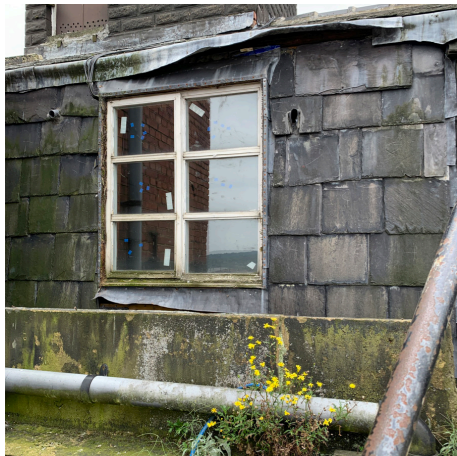
PHOTO E : Phase 2 existing top storey level roof and window condition
