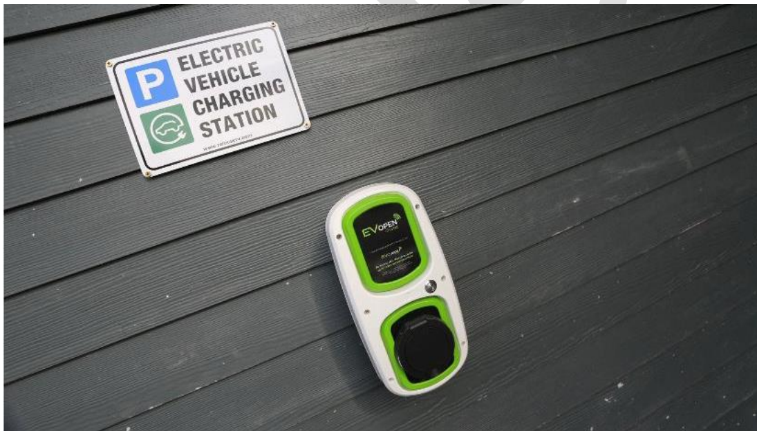
Electric Vehicle charging point
