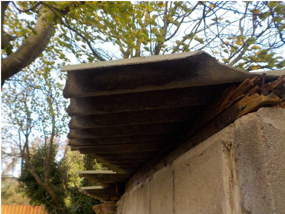
Photograph 8 Potential asbestos roofing material
