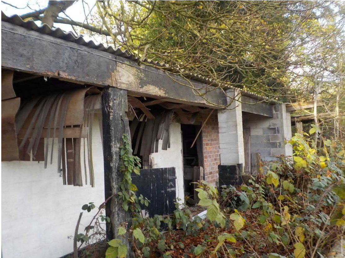
Photograph 7 Showing derelict stables in the western area of the site
