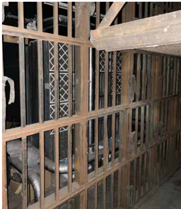
4.8.12 - Air Filter Chamber (Rm.37)
