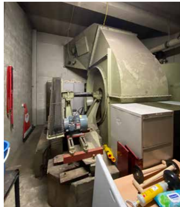
4.8.13 - Plant Room (Rm.38)
