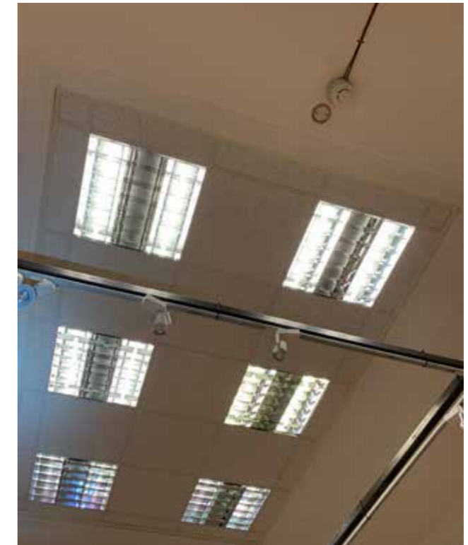
4.7.11 - Infilled rooflight opening to Gallery 1 (Rm. 87)
