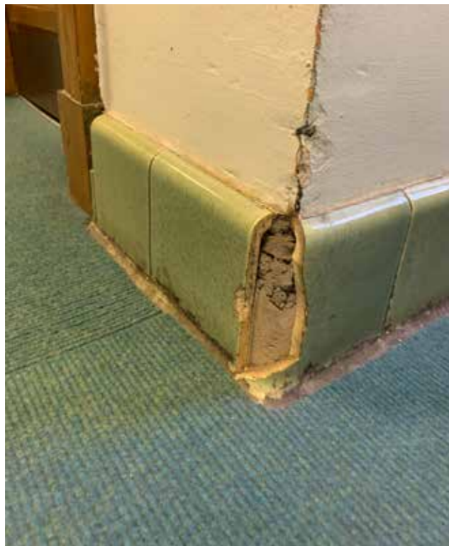
4.6.5 - Skirting to First Floor Stair Lobby (Rm.71)
