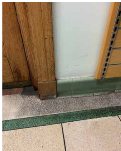
4.8.16 - Architrave to Boys WC (Rm.23)
