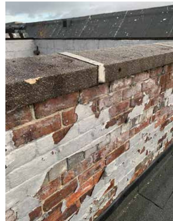
4.4.17 - Deteriorating roof parapet
