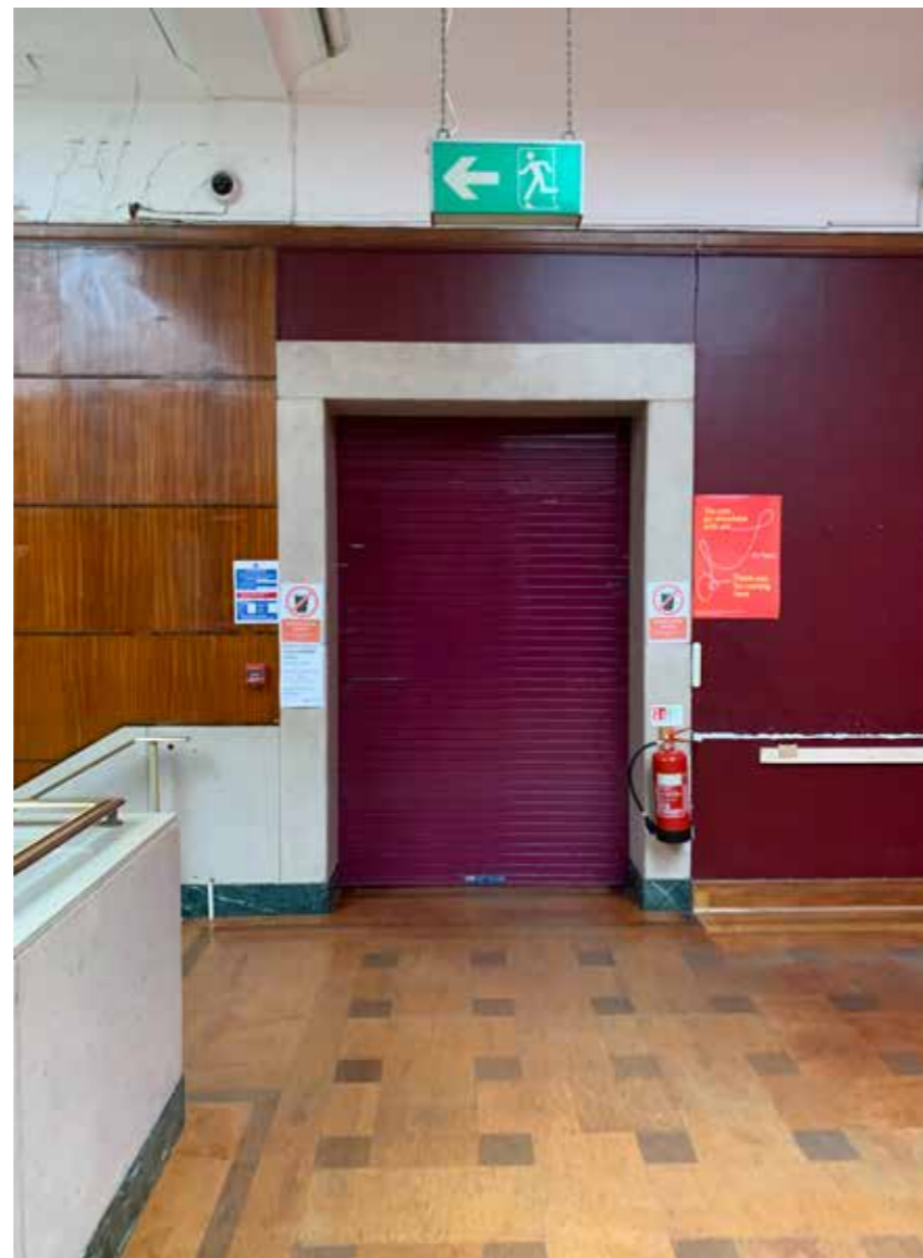
Lift and roller shutter to Gallery Entrance Lobby (Extension of Rm.91)
