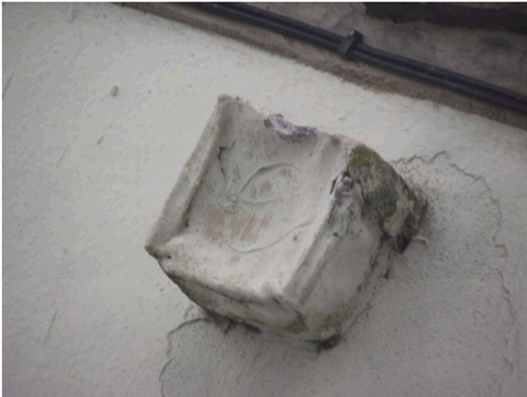
Photo 38 – Front elevation - assumed lead covering to nurlin end Chimneys
