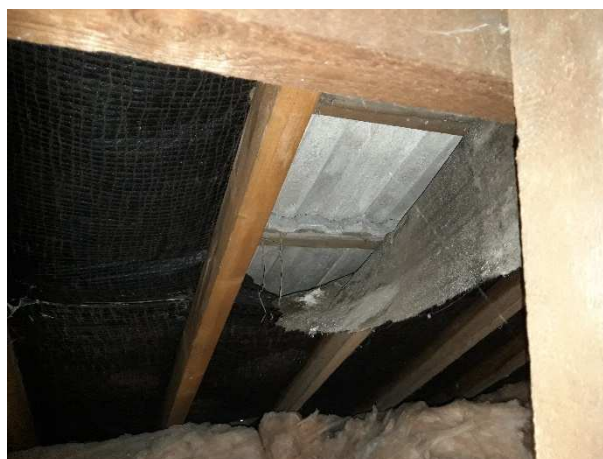
Photo 4: One of three areas of torn membrane.
