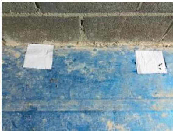
SAGM patches applied within Plot 5.
