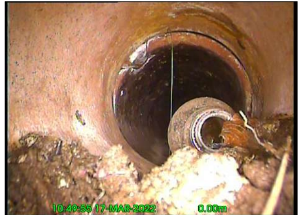
Photo: 4_3A 0m, Settled deposits, fine, 20% cross-sectional area loss, Start
