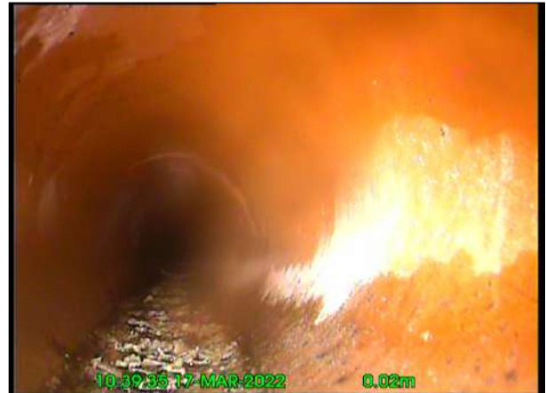
Photo: 2_3A 0m, Settled deposits, fine, 10% cross-sectional area loss, Start
