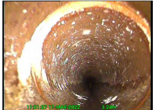
Photo: 5_9A 3.5m, Joint displaced, medium
