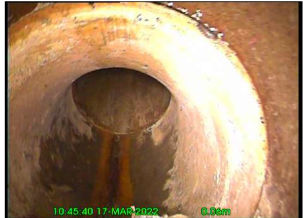
Photo: 3_3A 0.2m, Settled deposits, coarse, 15% cross-sectional area loss
