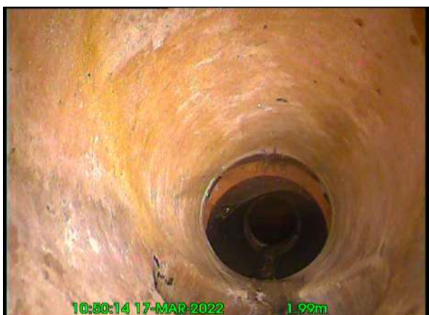
Photo: 4_7A 2.2m, Connection other than junction, at 6 o'clock, diameter 150mm Remarks: Dropshaft
