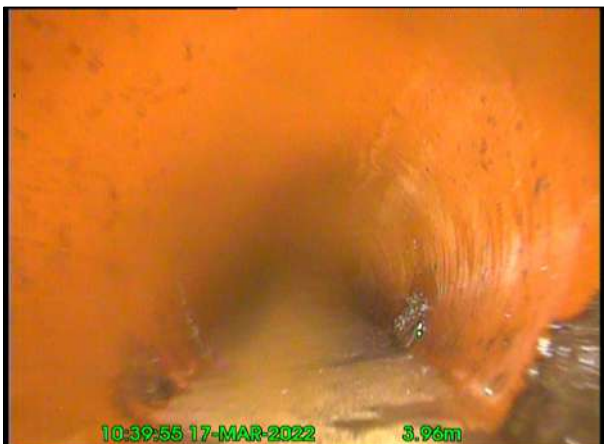
Photo: 2_5A 3.85m, Settled deposits, fine, 15% cross-sectional area loss, Start
