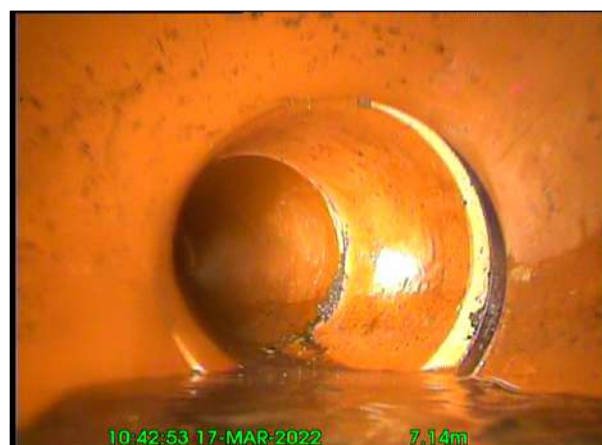
Photo: 2_10A 7.2m, Joint displaced, medium
