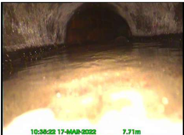
Photo: 1_8A 7.7m, Settled deposits, fine, 10% cross-sectional area loss, Start
