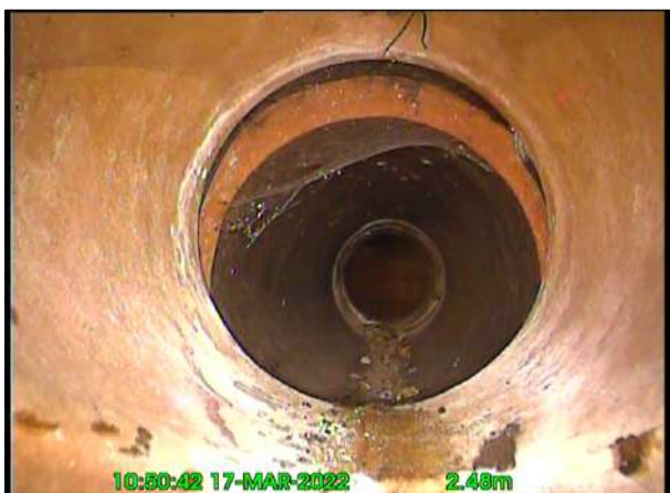
Photo: 4_9A 3.1m, Joint displaced, large
