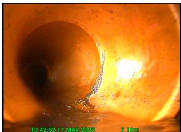
Photo: 2_9A 7.2m, Line deviates left
