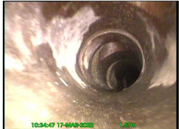
Photo: 1_3A 1.9m, Connection other than junction, at 1 o'clock, diameter 100mm
