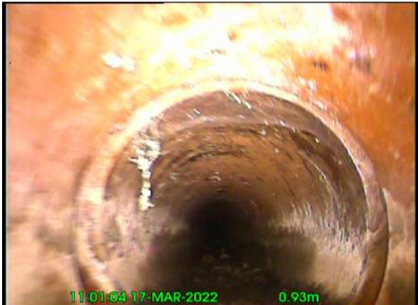
Photo: 5_7A 1.1m, Joint displaced, large
