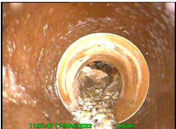
Photo: 5_10A 8.3m, Settled deposits, coarse, 10% cross-sectional area loss, Start
