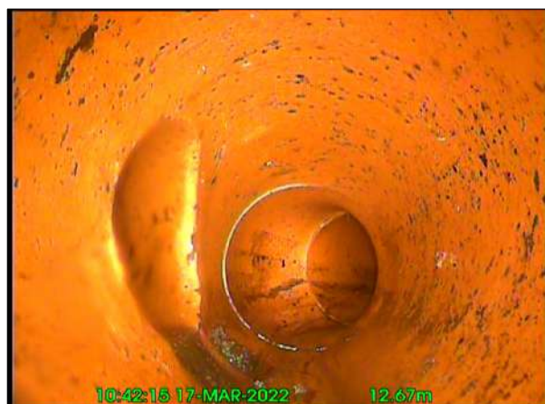
Photo: 2_12A 12.9m, Connection other than junction, at 9 o'clock, diameter 100mm
