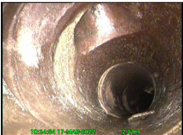
Photo: 1_4A 2.7m, Connection other than junction, at 11 o'clock, diameter 100mm
