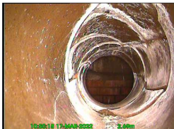
Photo: 4_8A 3m, Fracture, multiple at joint, from 9 to 5 o'clock, Start
