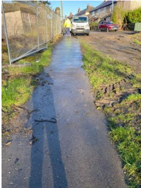
UNEVEN PUBLIC FOOTPATH DOWN FROM PLANE STREET
