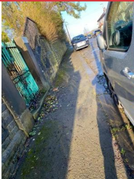
PUBLIC FOOTPATH WITH DISTURBED KERBS Facing back up plane street
