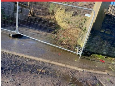
CHIPPED KERBS TO PUBLIC FOOT PATH
