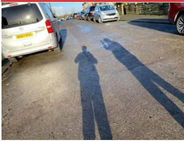
UNEVEN ROAD SURFACE FACING UP TO PLANE STREET
