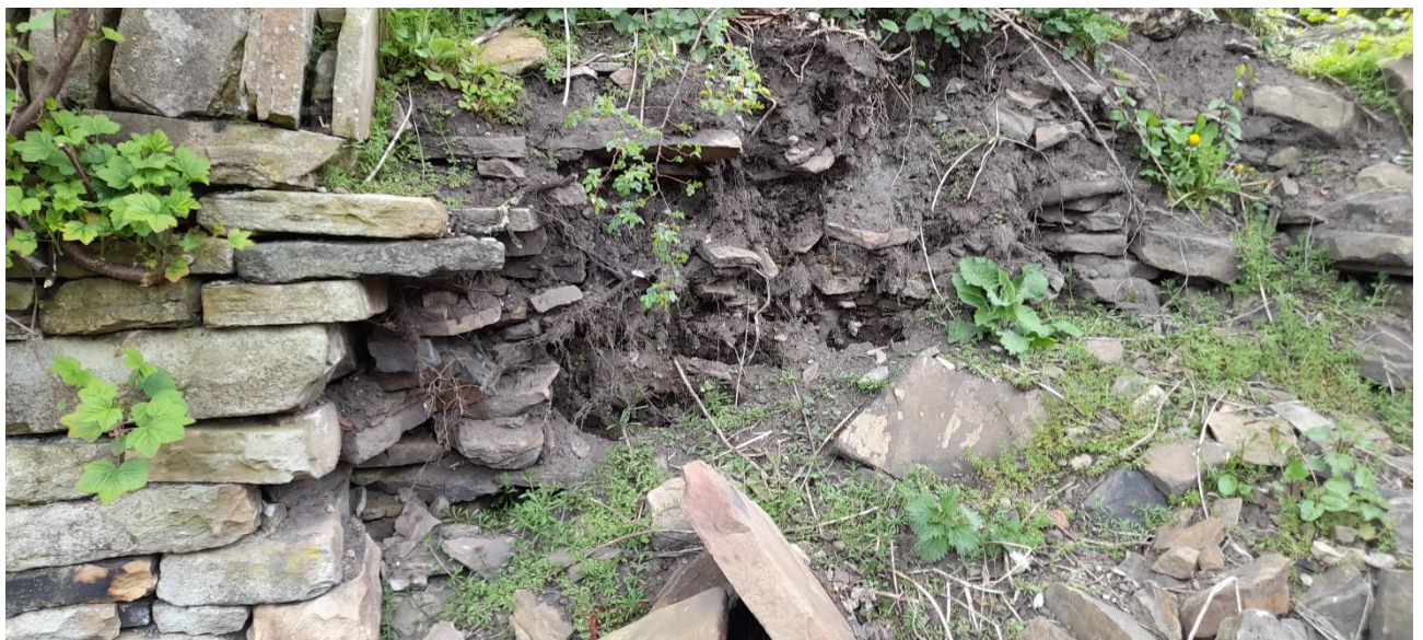
Photograph 4 – Enlargement of collapsed section showing root growth.
