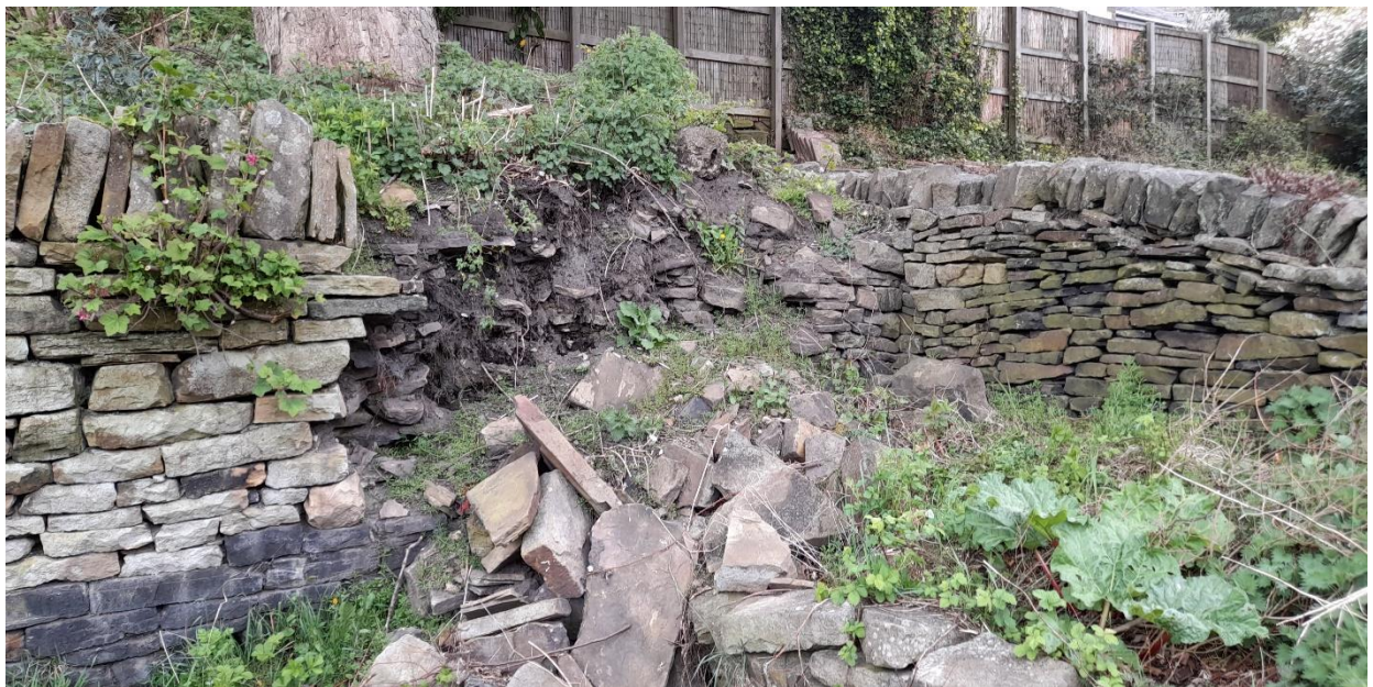
Photograph 2 – Collapsed section in corner, close up.
