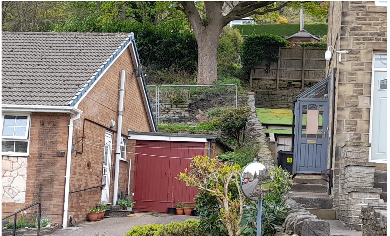
Photograph 1 – Collapsed section visible at rear of garden.
