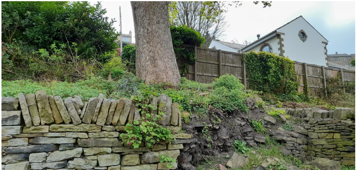
Photograph 3 – Collapsed section showing proximity of tree.
