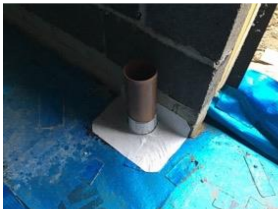
Plot 7 sealed pipe penetration
