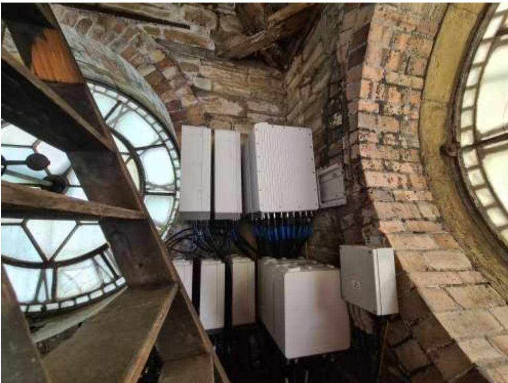
Figure 2: Shows the Combiners and ERS's locations which is not accessible to the public.
