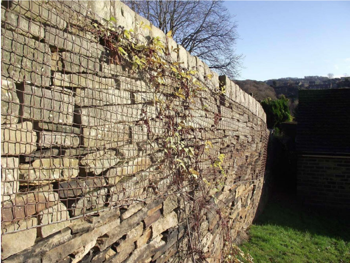
Photo 5 – Distortion, lateral movement and fracture to existing dry stone boundary retaining wall.
