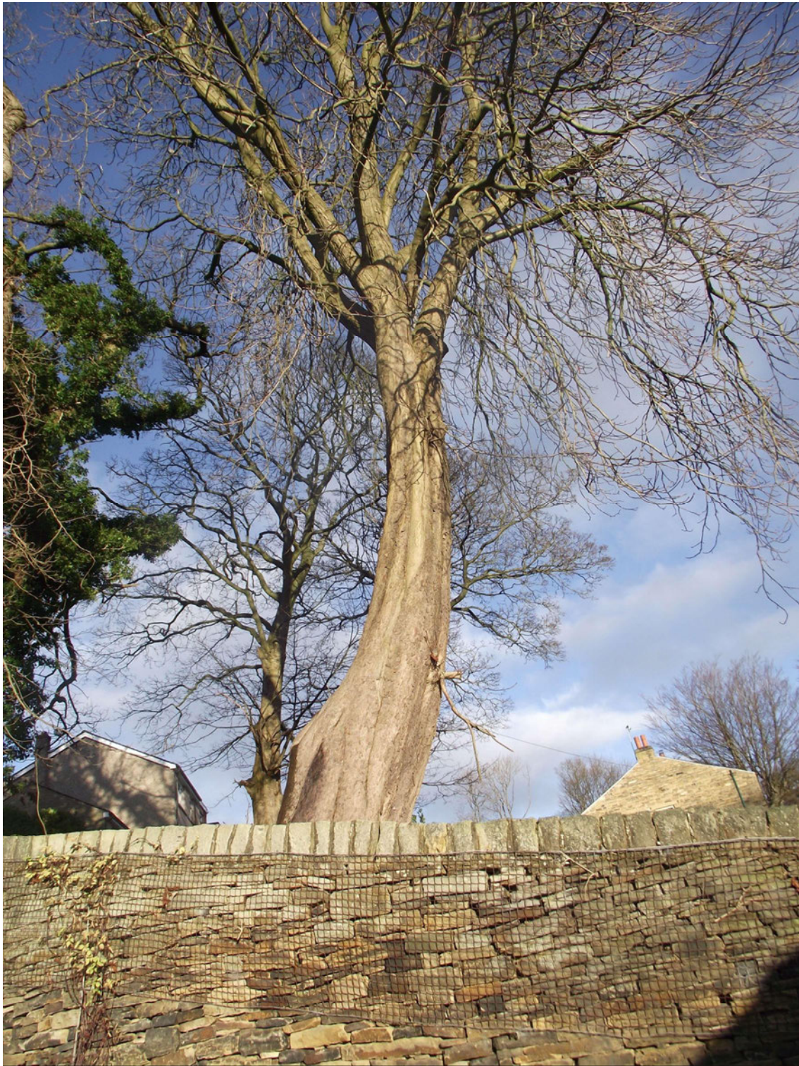
Photo 1 – Proximity of mature broad leaf tree to boundary retaining wall.
