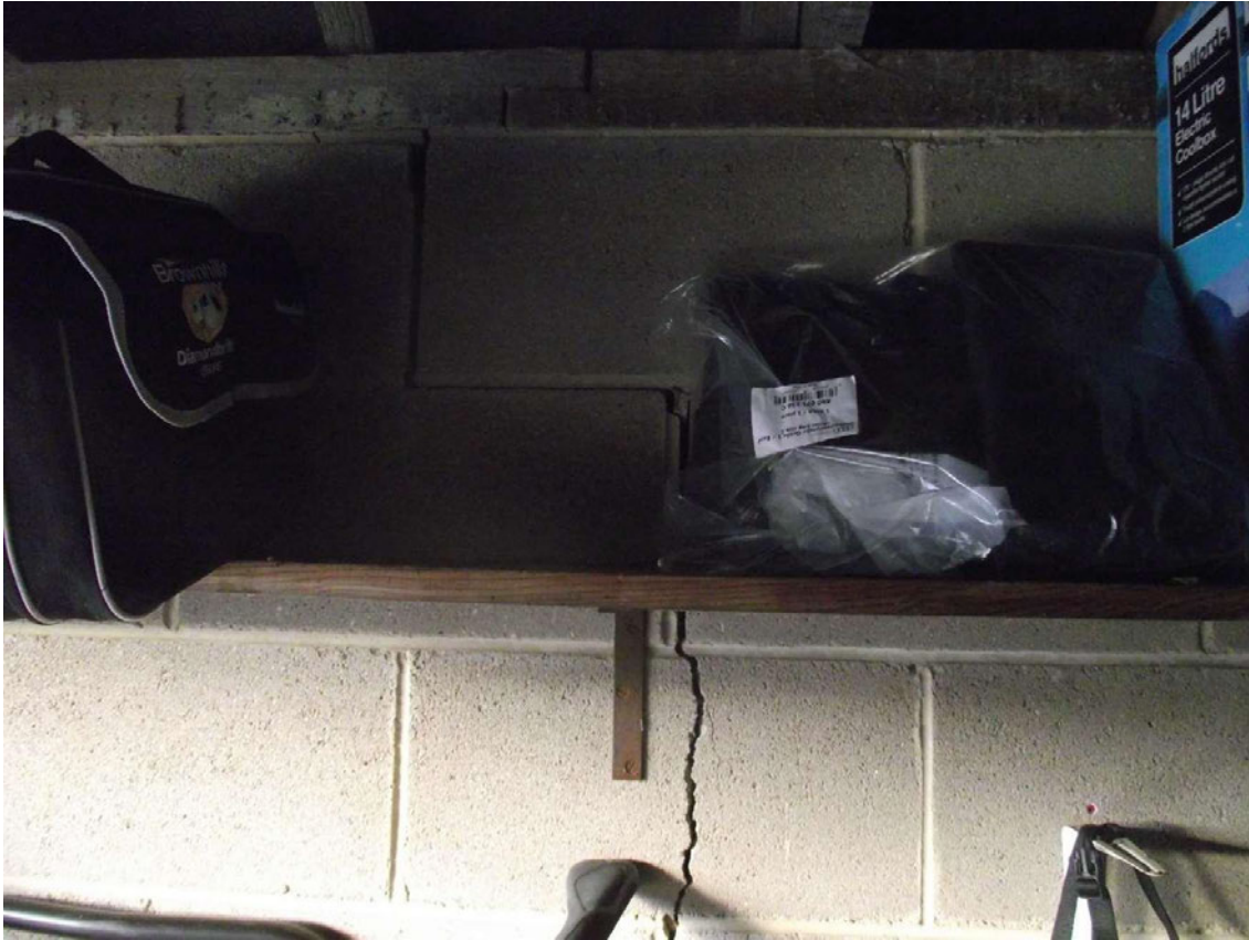
Photo 7 – Cracking to internal leaf of blockwork, garage. Coincident with cracking to external leaf, West elevation
