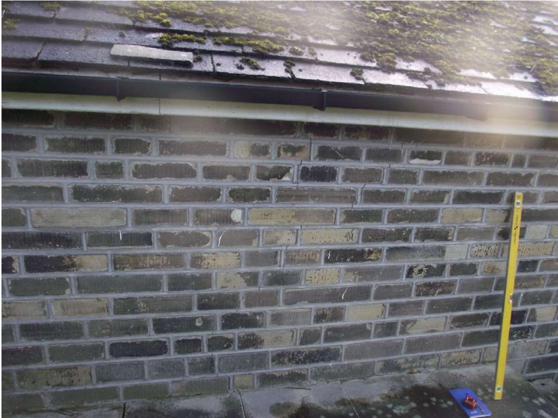
Photo 6 – Racking crack in mortar joints to stone outer leaf to existing Garage, West Elevation
