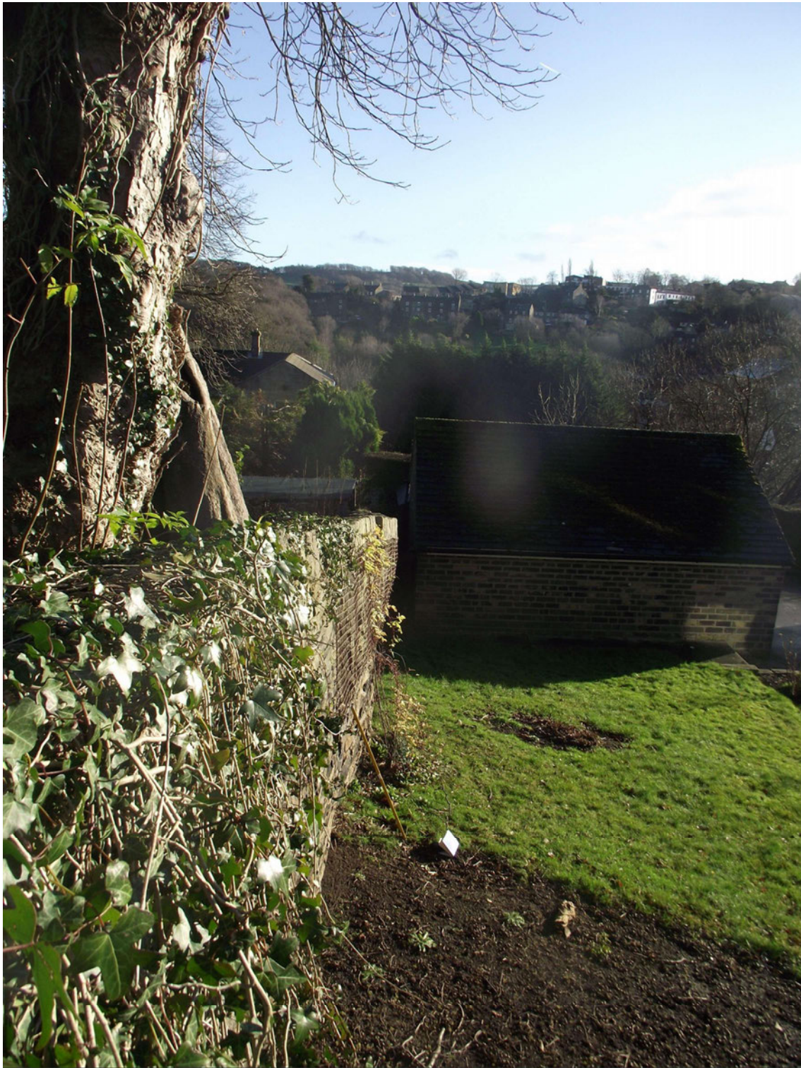
Photo 3 – Lateral movement and distortion to existing dry stone boundary retaining wall
