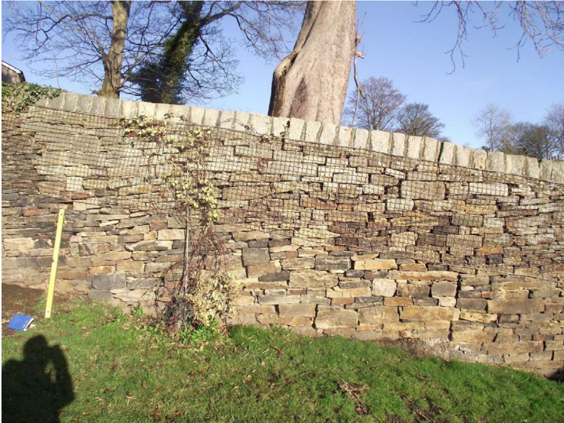
Photo 4 – Elevation on worst affected section of wall – fractures to wall each side of mature tree.
