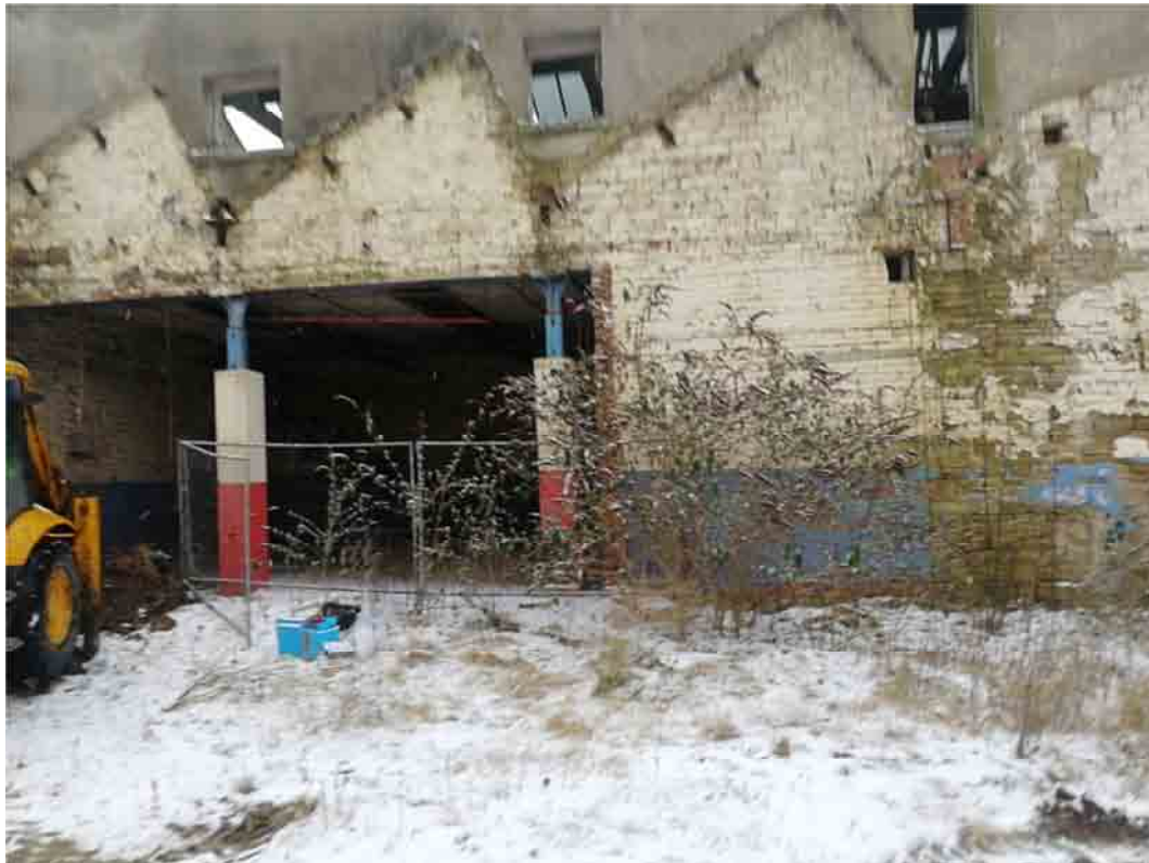
Photograph 14: Large dilapidated building in Area A.
