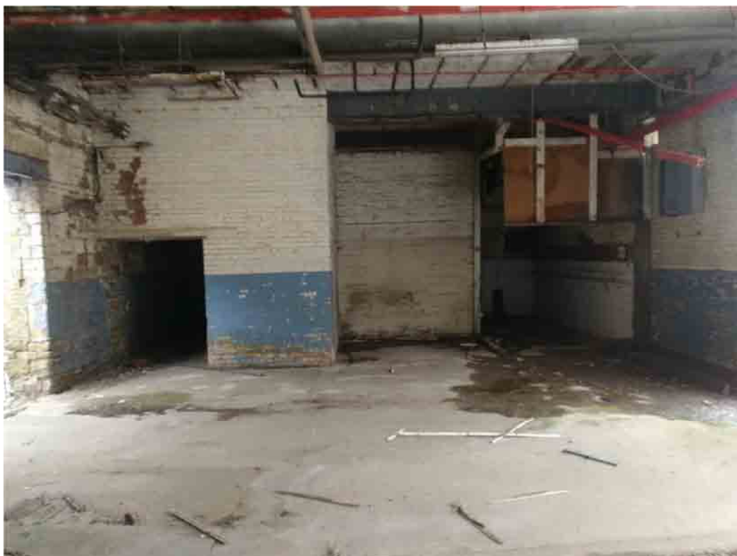
Photograph 15: Inside the dilapidated building in photograph 14.
