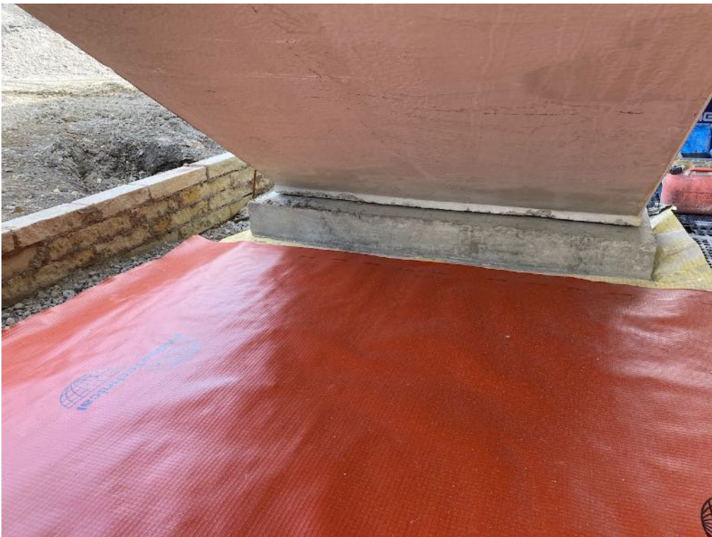
Plate 10: PAG membrane taken over membrane under internal stairs (13/08/2021)
