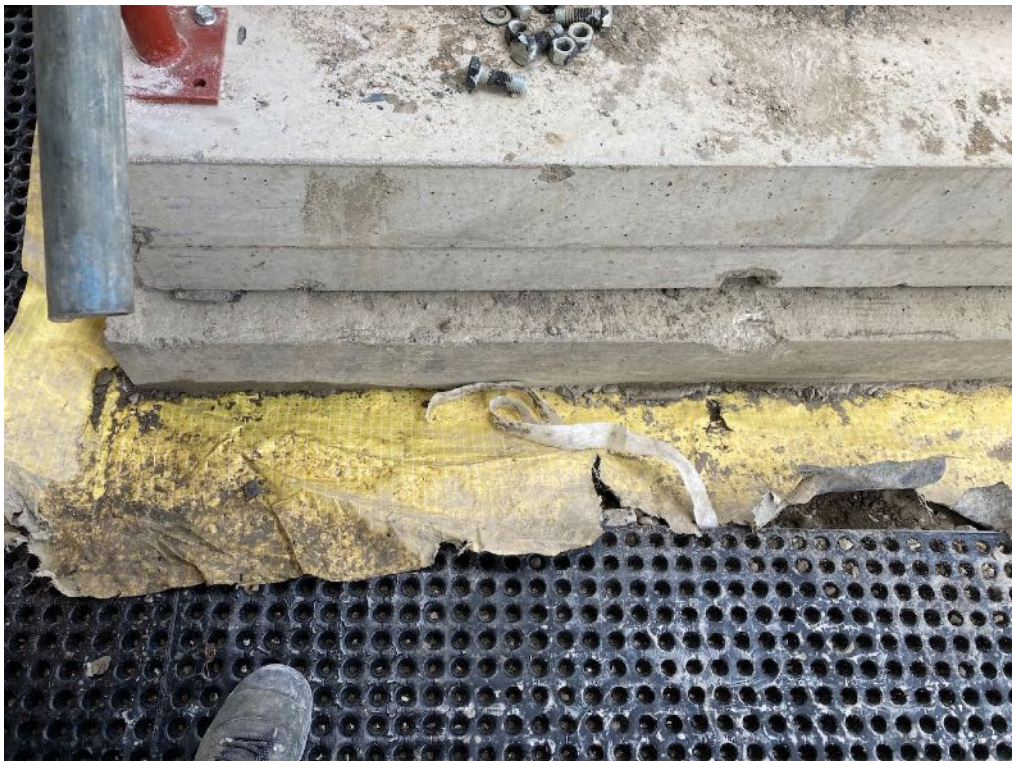
Plate 17: Membrane in front of NW internal staircase damage on front face (16/08/2021)
