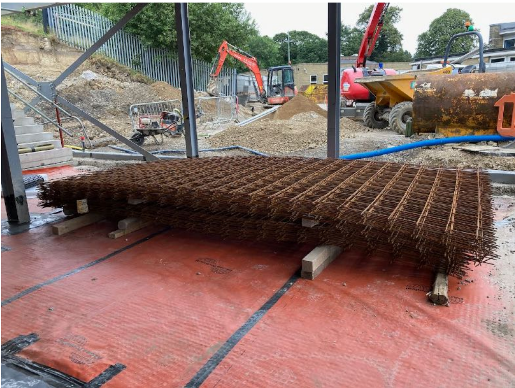
Plate 22: Mesh stored on timbers after previous damages noted (01/09/2021)
