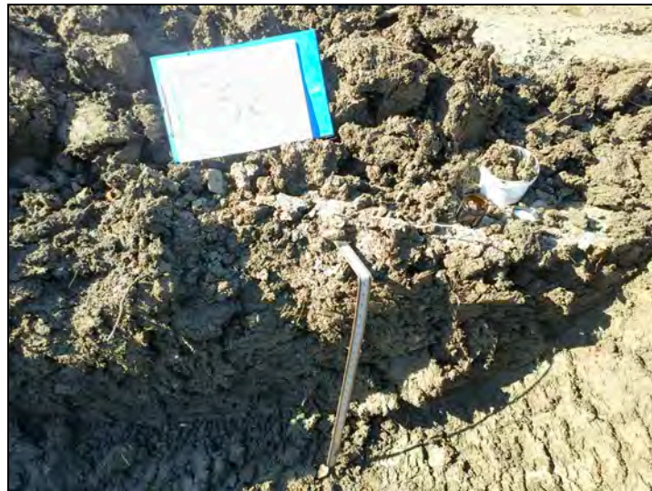
Trial Pit topsoil sampling for Plot 36 rear garden, ruler proving depths 600mm
