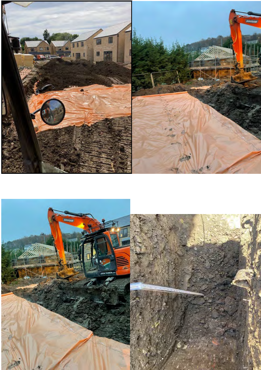
Figure 5 General View of Geotextile and Topsoil being placed and checked for thickness
