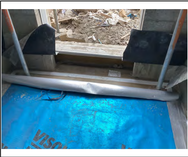
View showing incomplete Gas Barrier
