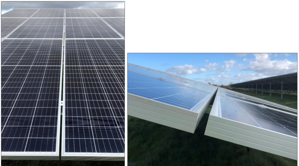
Figure 5: Photovoltaic Panel Gaps - Example
