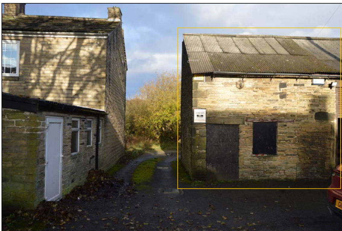
Photograph 5: Present access to the rear areas of the property's plot (looking north), with the barn (Building 1) indicated.
