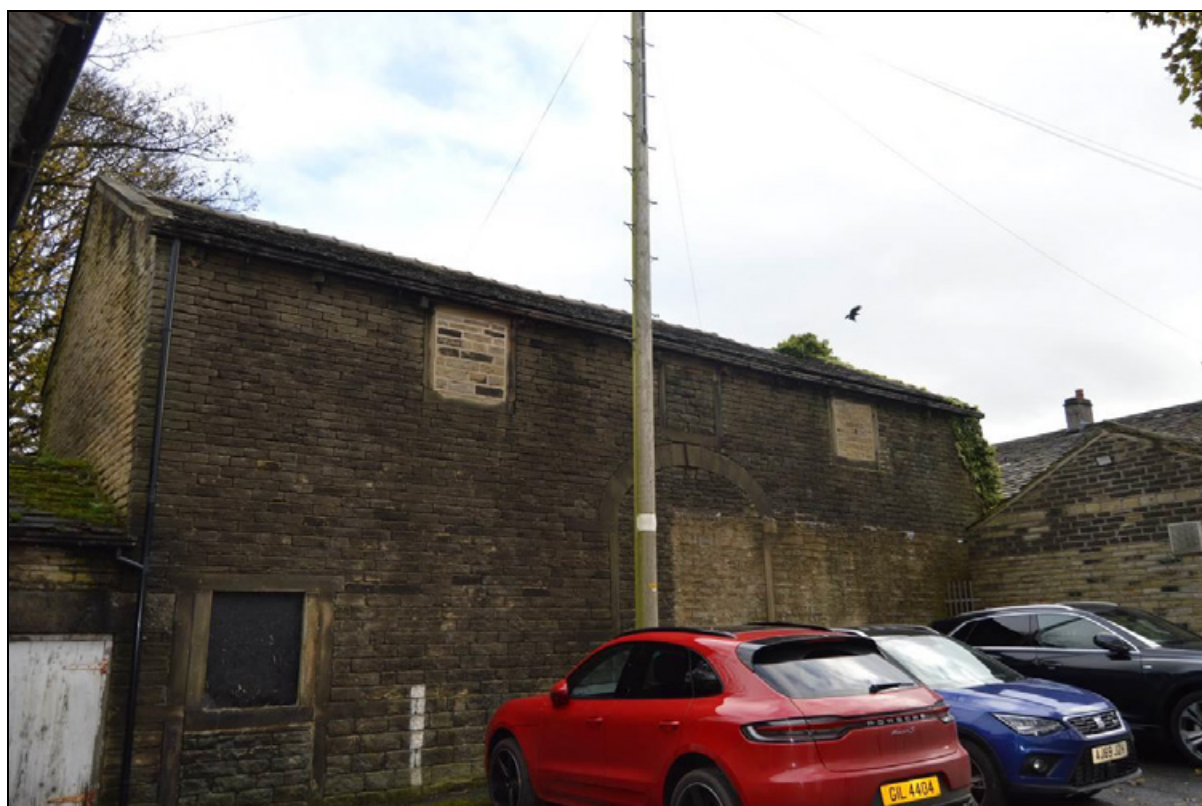
Photograph 25: Larger barn flanking the east of the weaver's house rear yard, outside the property boundary (facing south east).
