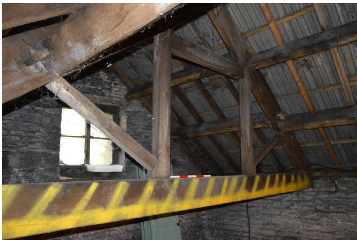
Photograph 22: Window to the east gable from the first floor level interior. Scale 0.5m.
