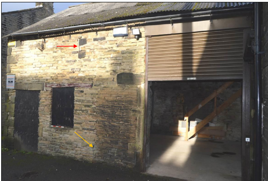
Photograph 15: Apertures to south elevation (facing north west) and construction breaks (indicated by red and yellow arrows). Scale 0.5m.
