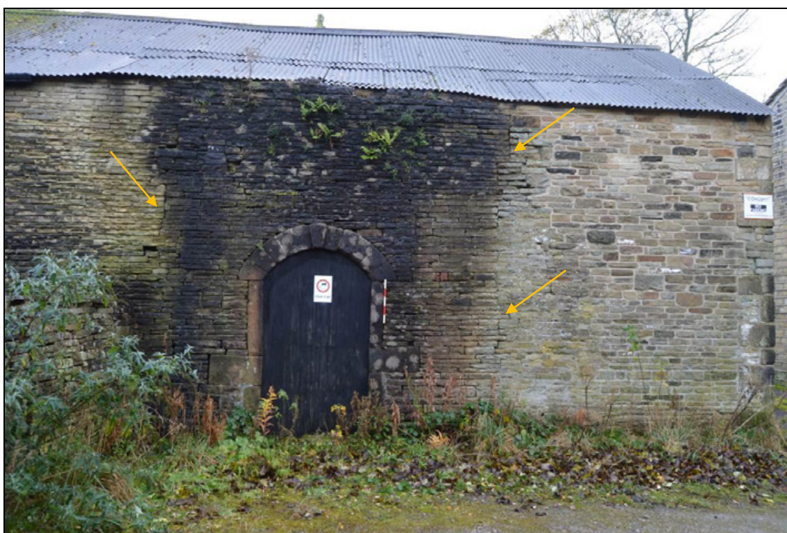
Photograph 14: North wall (facing south) with stone arched door and construction breaks (indicated by yellow arrows). Scale 0.5m.
