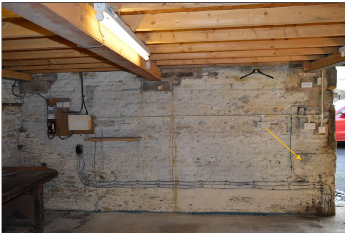
Photograph 17: Internal face of the barn's south elevation with quoin stone jamb indicated by yellow arrow: (facing south).
