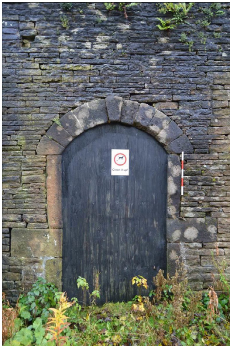
Photograph 12: North, field wall (facing south), with blocked stone framed doorway. Scale 0.5m.
