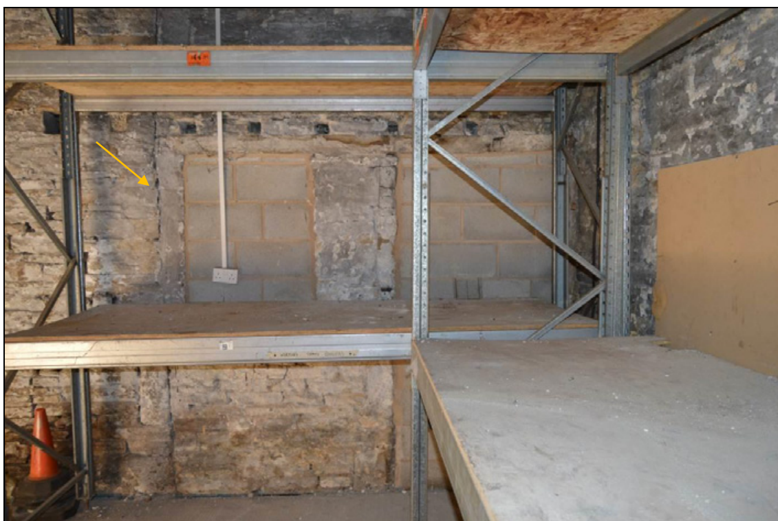
Photograph 16: Internal face of the barn's south elevation. Note construction break (indicated by yellow arrow) and joist slots.
