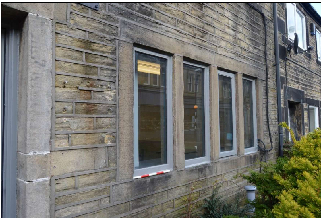
Photograph 9: Example of stone mullion windows to south elevation, ground level (facing north east). Scale 0.5m.
