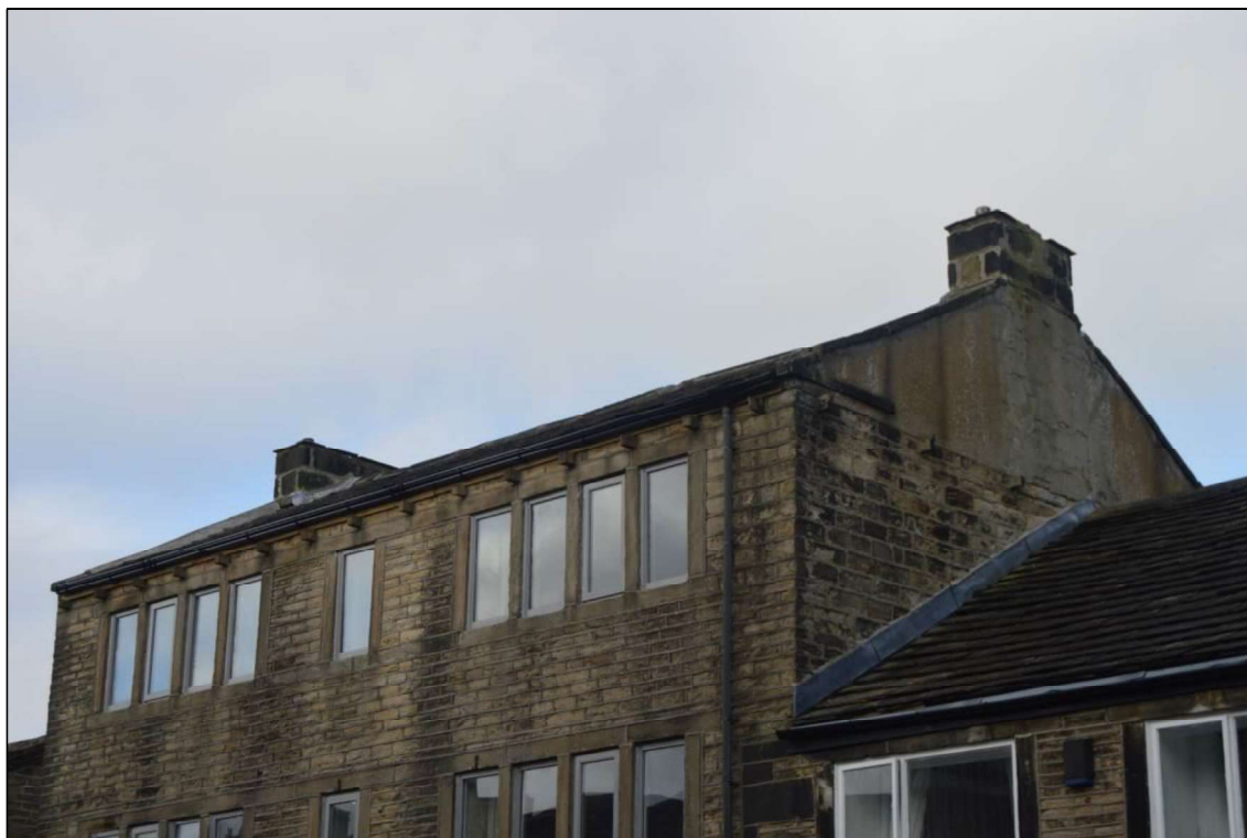
Photograph 11: Stone corbels set below the roof line and east gable features (facing north west).
