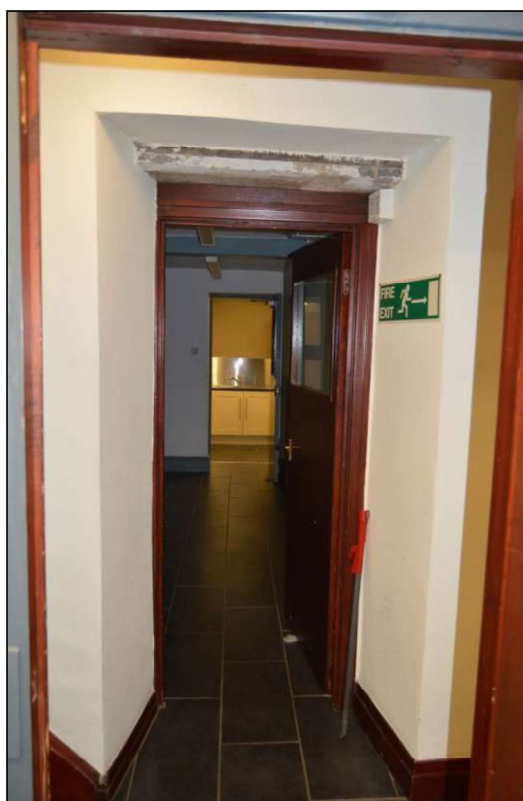
Photograph 24: Internal link through north elevation of three storey weaver's house to later extensions.
