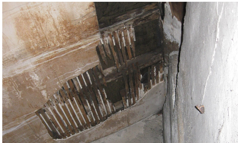
Figure 2.4.2 Water ingress damage to lath and plaster ceiling (BDP 2020)
