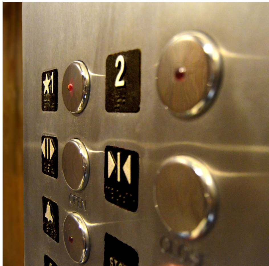
Figure 3.3.1 New lift (Photo by Russ Ward on Unsplash)
