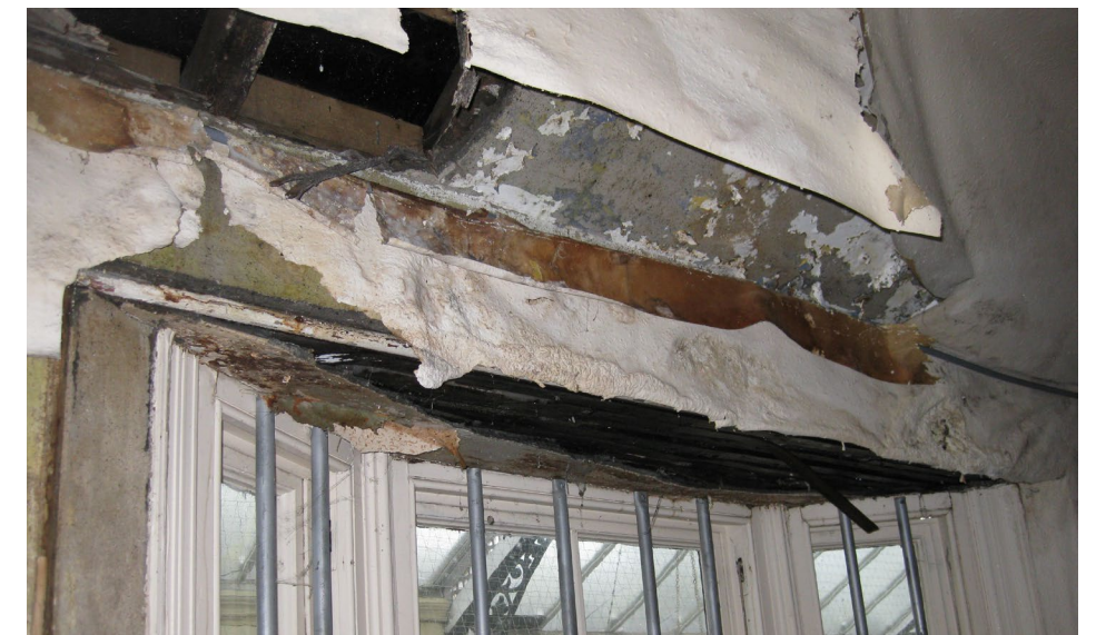
Figure 2.4.4 Water ingress damage to finishes and structure (BDP 2020)
