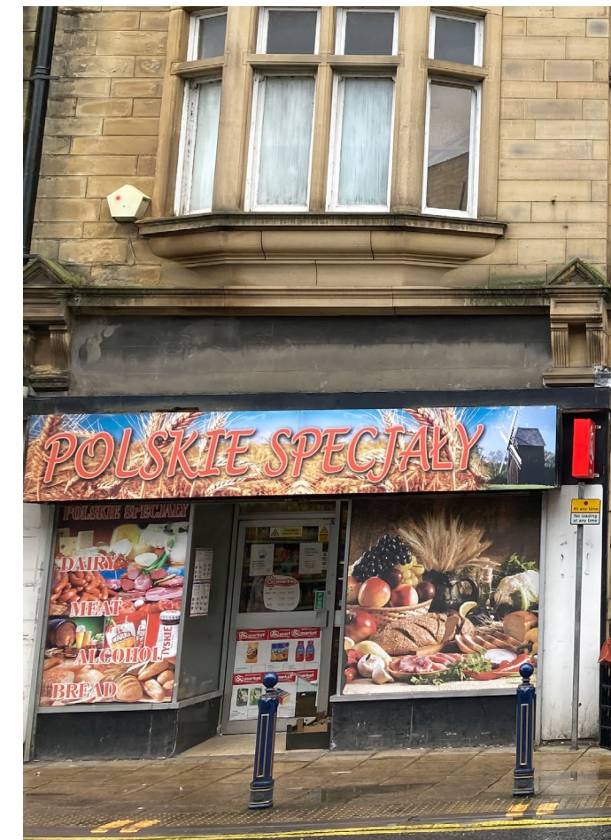
Figure 2.3.4 Poor quality adapted shop front with lost details (BDP 2020)
