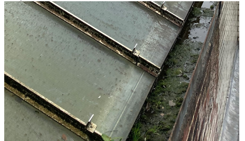
Figure 2.4.8 Blocked gutters due to lack of access (BDP 2020)
