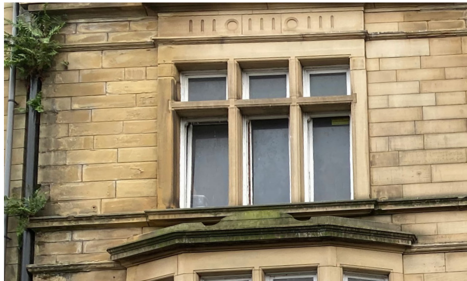
Figure 2.4.7 Failing rainwater goods resulting in build up of vegetation (BDP 2020)
