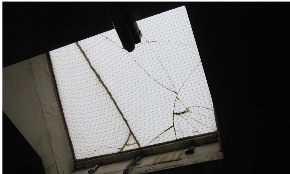
Figure 2.4.6 Broken skylights (BDP 2020)
