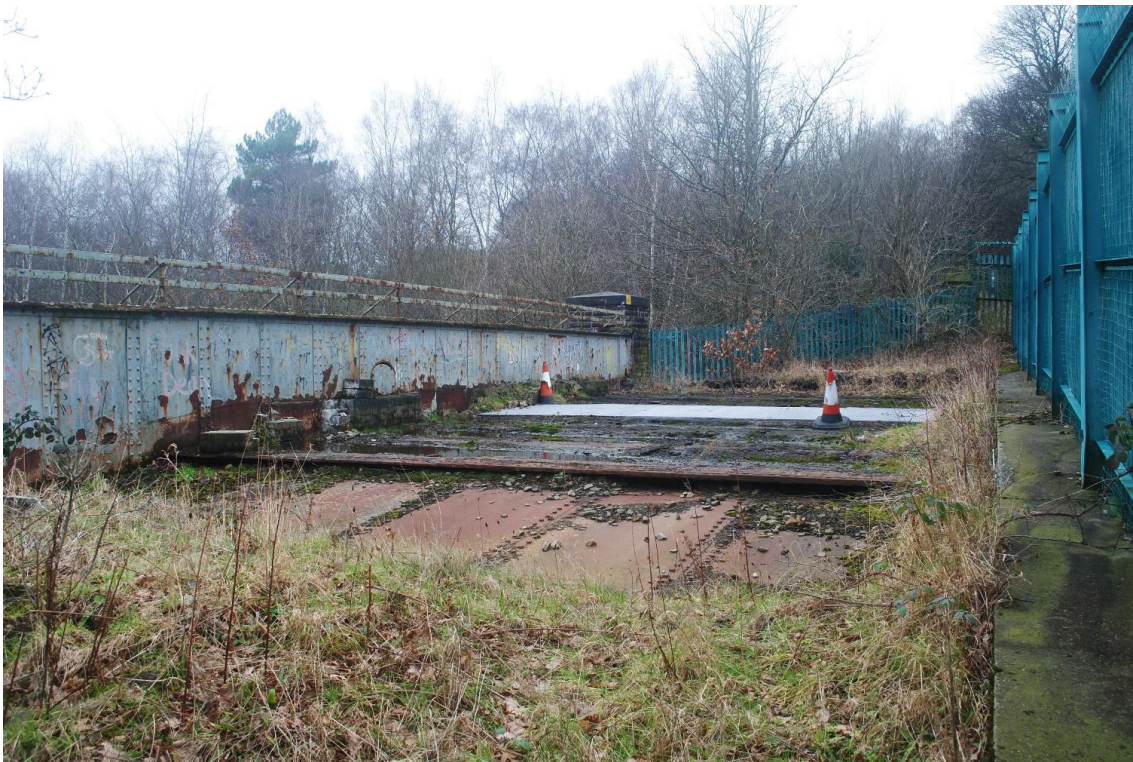
Plate 5-5 - Western part of bridge deck, fenced off due to structural condition, from south.
