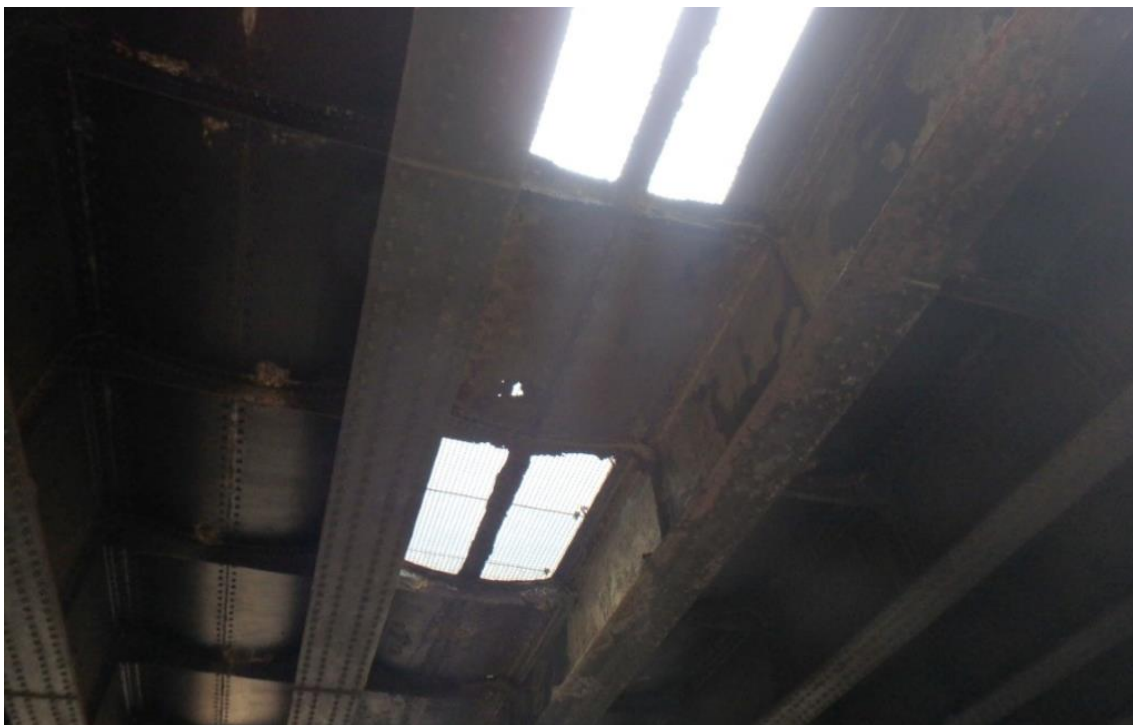
Plate A-6 - General view of the underside of the deck, showing corrosion and loss of deck plates between main cross girders (Network Rail Inspection Report, November 2020).
