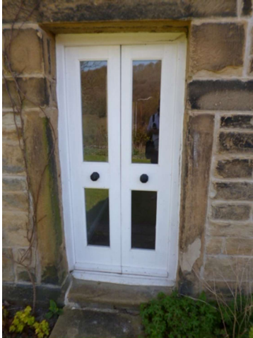
Typical single glazed door in listed side of dwelling and typical entrance door below
