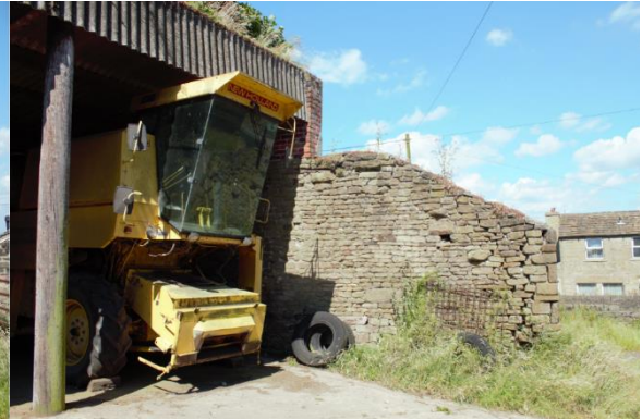
Figure 20: View of north end of open-sided shed, showing earlier structure beneath twentieth century building
