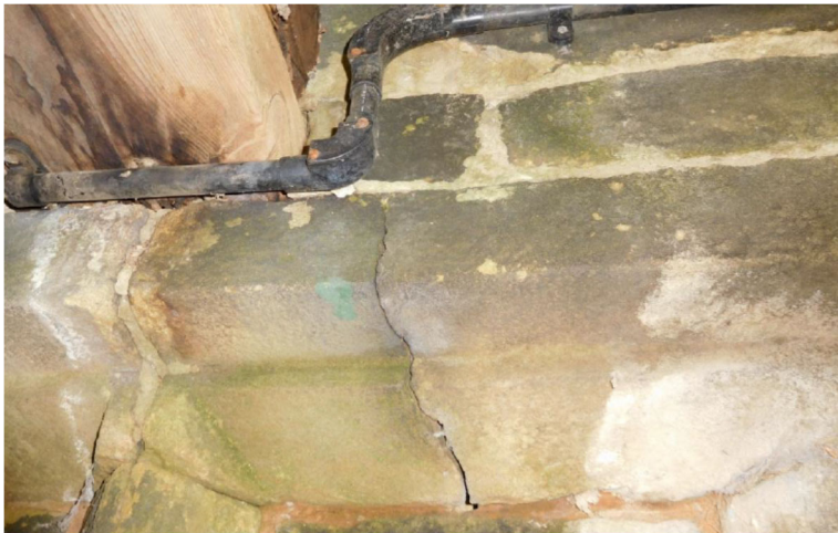
Failed external wall lintel
