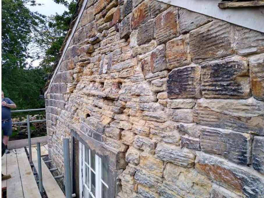
Photograph 2. Area of severely perished stonework
