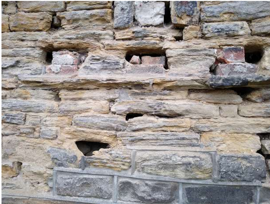
Photograph 3. Close-up of perished stones around doveholes
