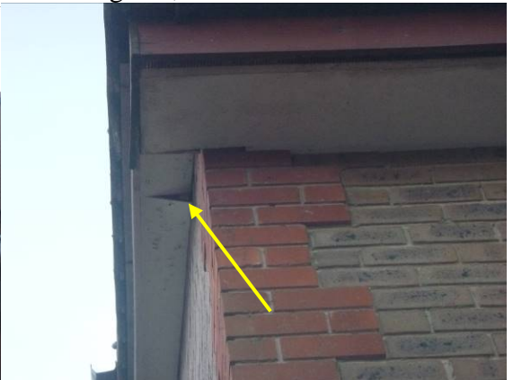
P6 Gap in soffit, East corner
