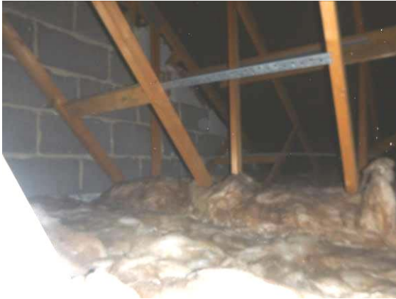
P7 Loft, felting in good condition
