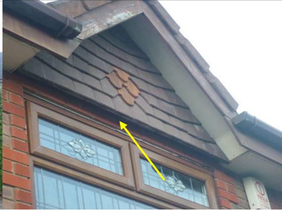
P2 Possible gap under hanging tiles
