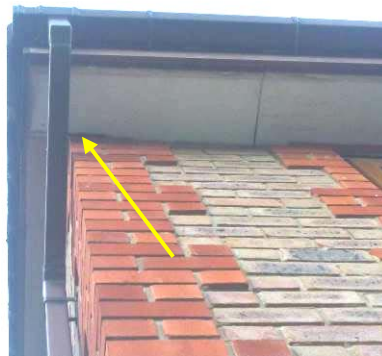
P3 West corner, gap under soffit
