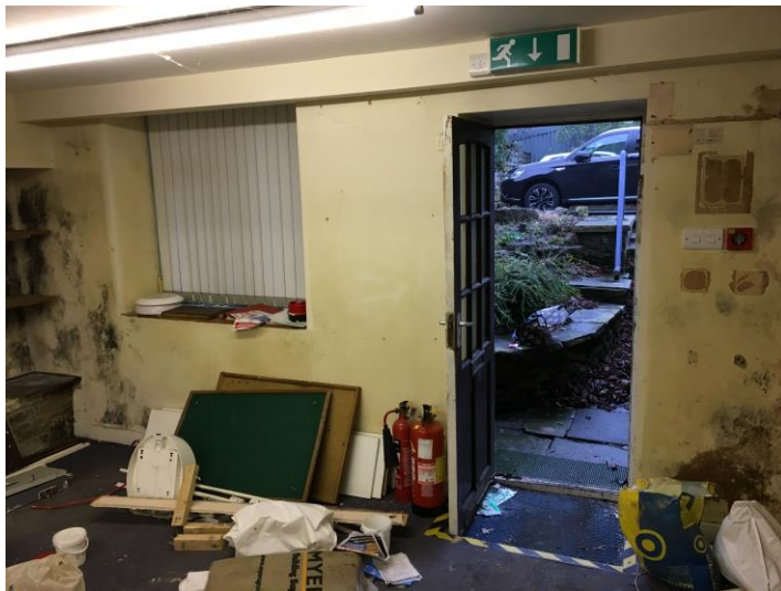
Figure 5: Mould to wall in basement unused office
