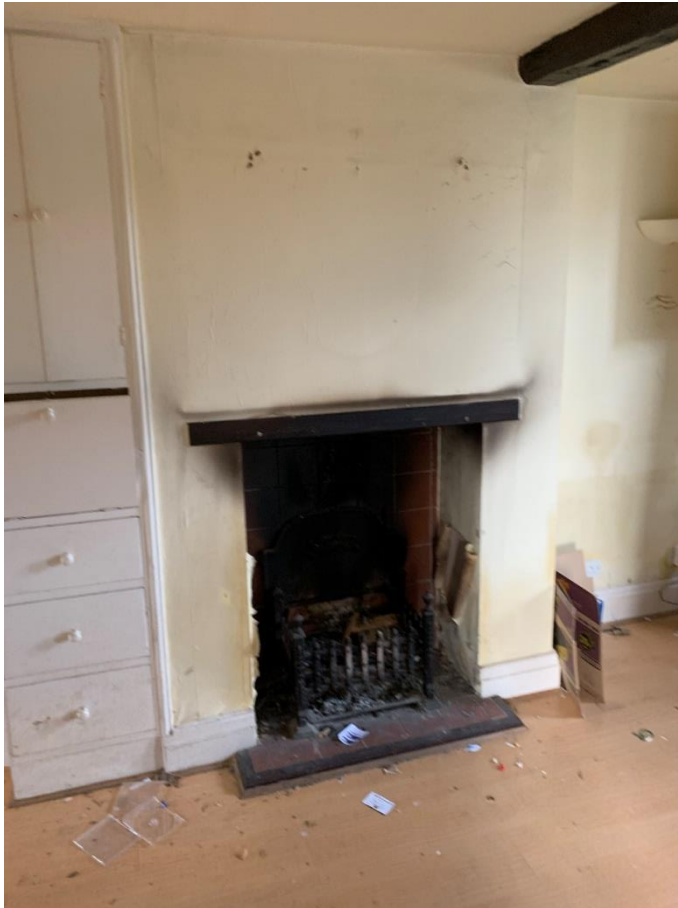
Unsafe fire within existing dining room posing risk to life with Carbon monoxide exposure.
