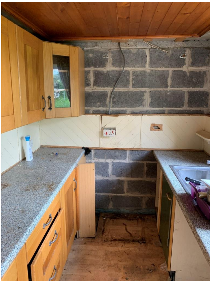
Unsafe/exposed electrics within kitchen.
