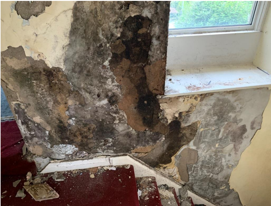
Severe water ingress at existing single storey roof abutment to head of staircase
