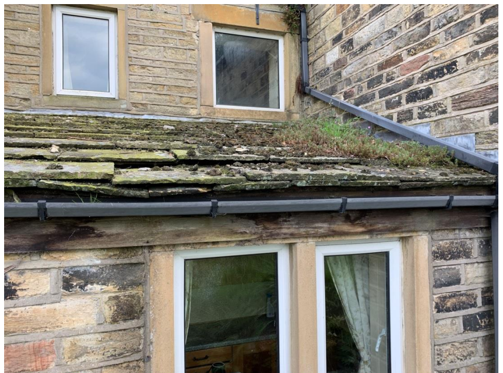
Rear lean to roof failure with rotten roof timbers not adequately supporting stone slate roof covering.
