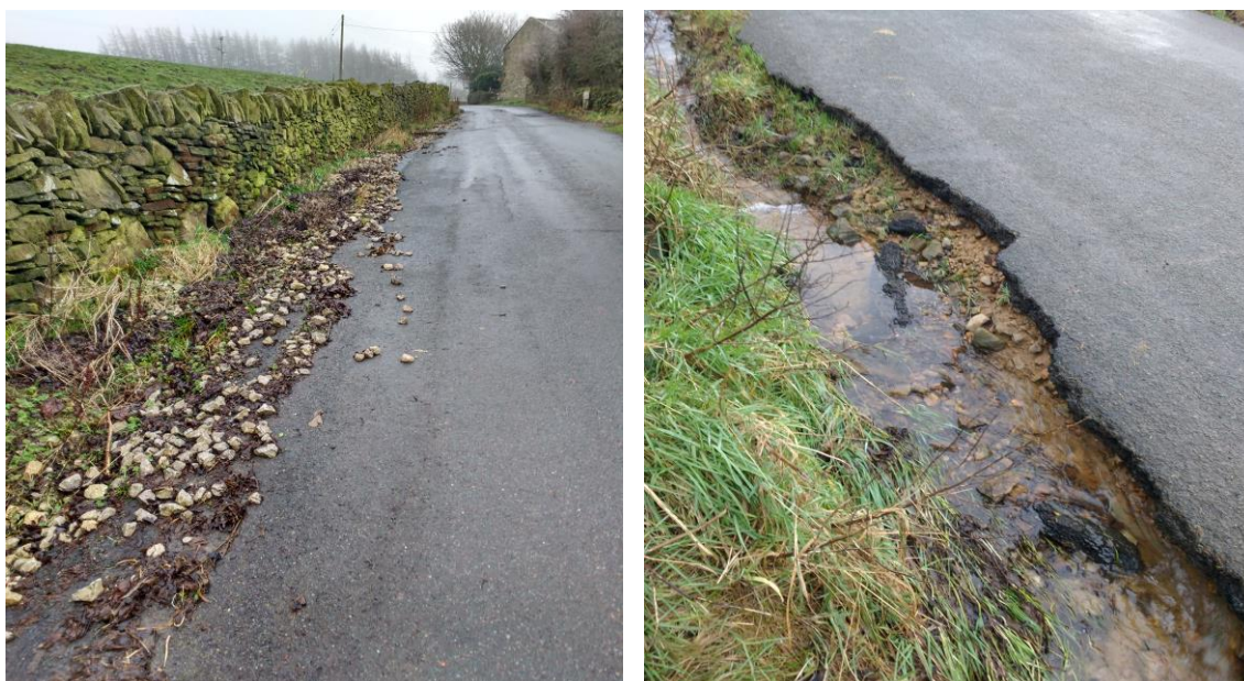
Illustration of drainage gulleys and water damaged tarmac on Lingards Road
