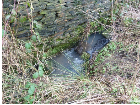
Water flow at northern end (note poor water quality)
