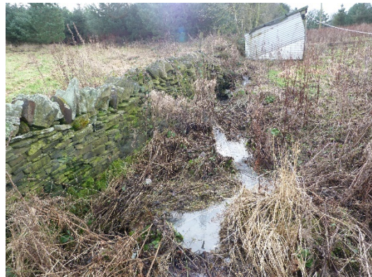
Segment of collapsed channel
