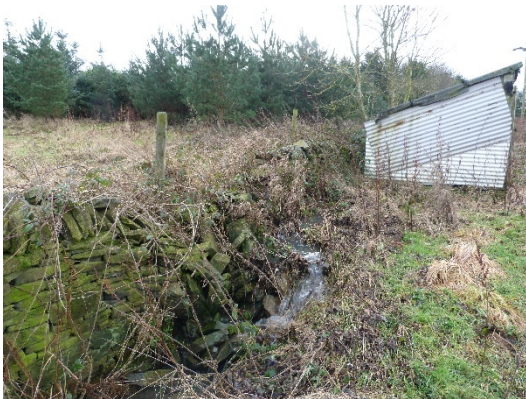
Segment of collapsed wall
