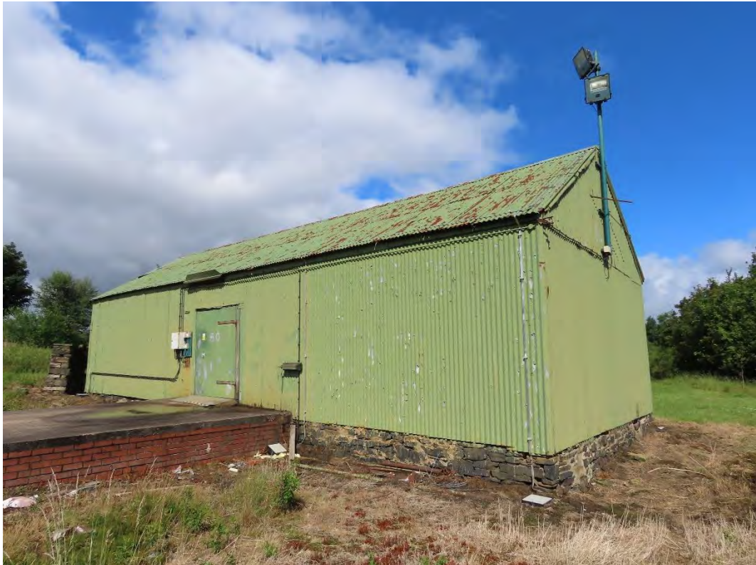
Photograph 7: Corroaged metal storage shed
