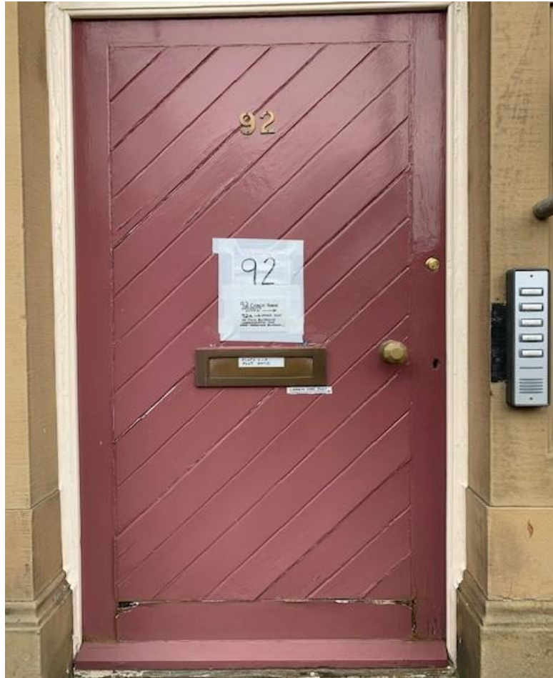
Photo of current over-boarded main rotten Front Door
