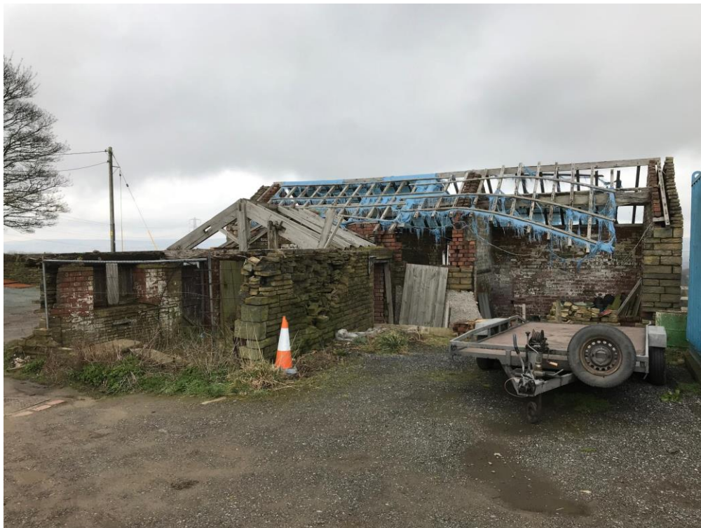
The Mistal existing condition of disrepair.
