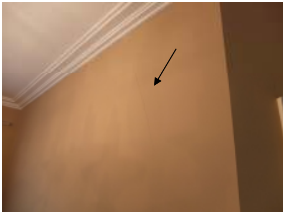
Internal crack to left internal wall on front stairs shared with front bathroom
