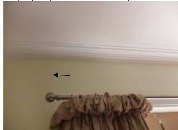
Internal cracking above left to rear left lounge French doors
