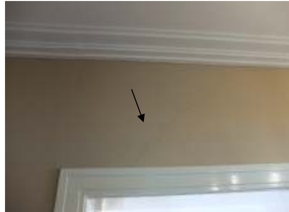
Internal crack above rear facing internal door leading to rear left lounge in front hallway
