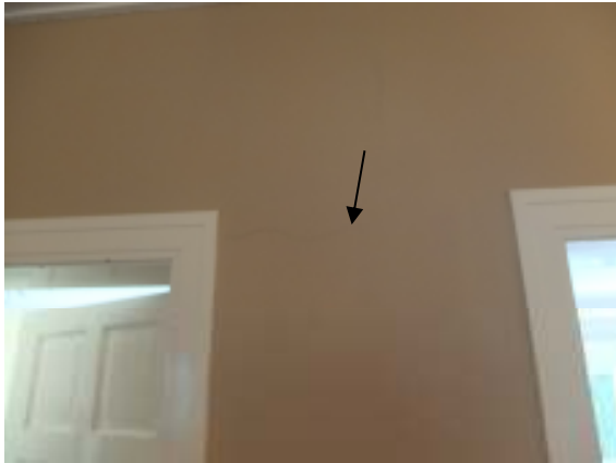
Internal horizontal crack between rear left and right bedrooms
