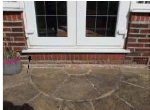
External cracking in loose bricks beneath rear left lounge French doors
