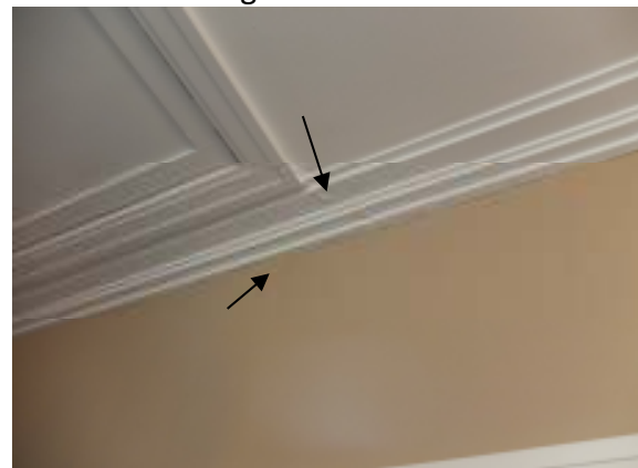
Internal cracking to wall and coving adjacent to loft hatch adjacent to internal door leading to rear left bedroom
