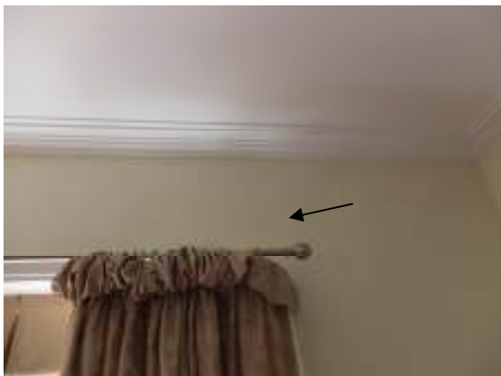
Internal cracking above right to rear left lounge French doors
