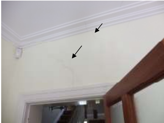
Internal crack above front right internal door to rear left lounge
