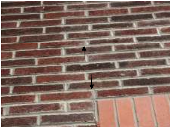
External cracking above right to rear left lounge French doors
