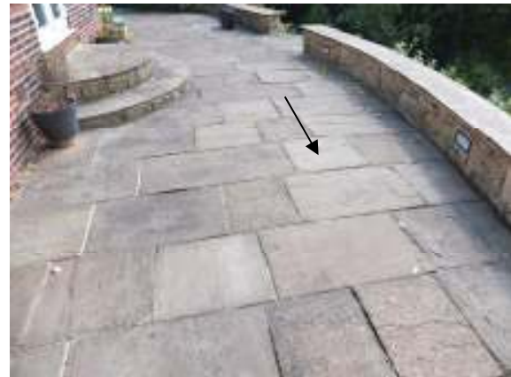
External movement to raised patio to rear of property due to rain water percolation
