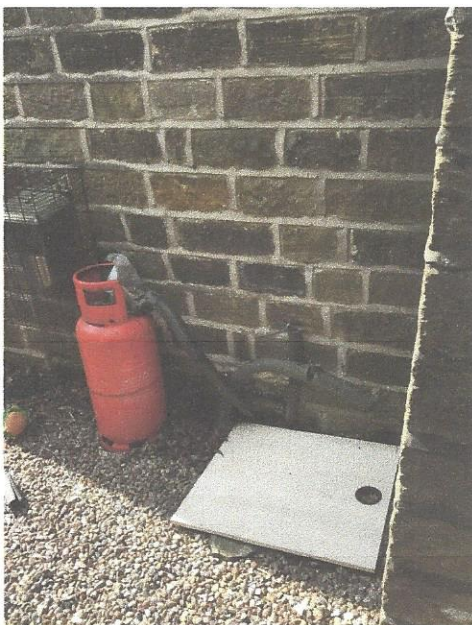
Image 3 - Location of Boiler
