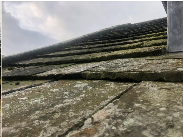
Plate 6. Slightly lifted roof tiles on southeast
