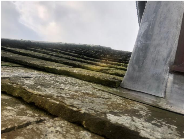
Plate 7. Slightly lifted roof tiles on southeast
