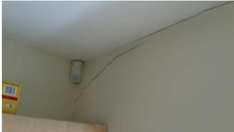
FIGURE 03 Kitchen - Diagonal crack damage to rear wall.
